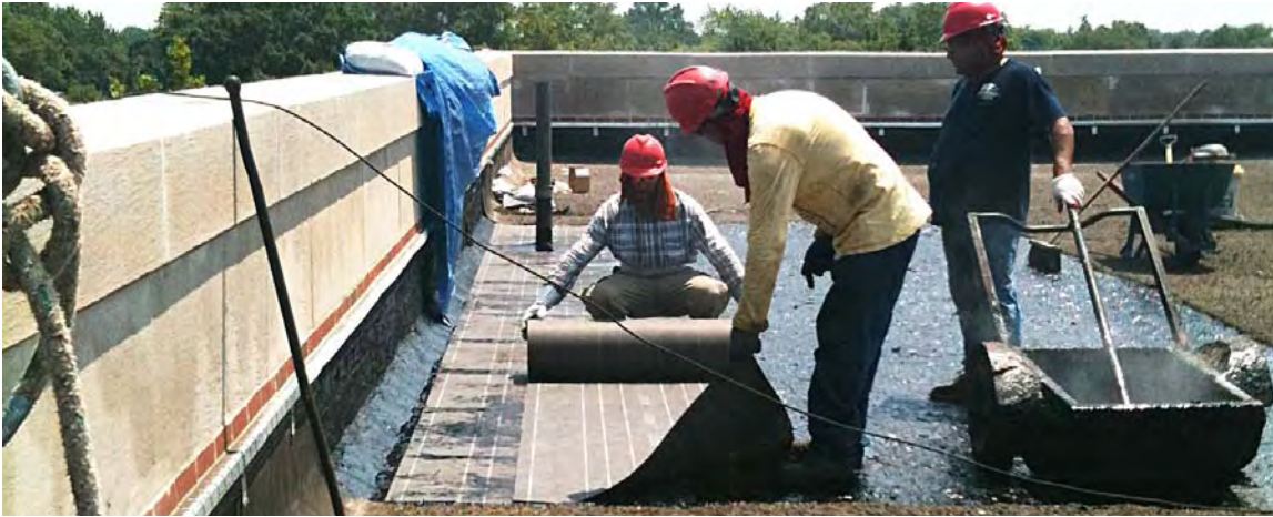
Figure 4-9: Installation of water- proofing membrane during construction of a green roof at PS118 in Queens.
