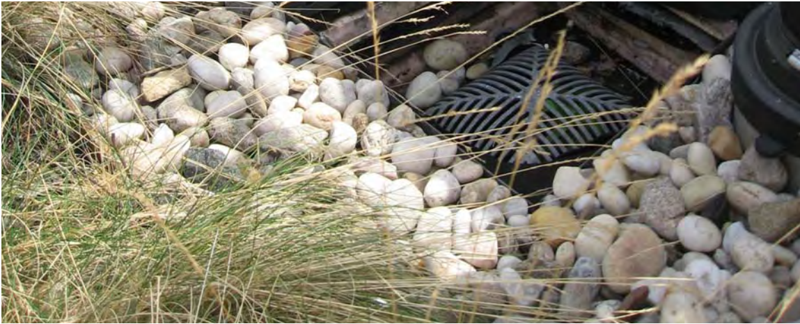
Figure 4-21: Green roof drain inspection cham- ber on St. Simon Stock School in the Bronx.
