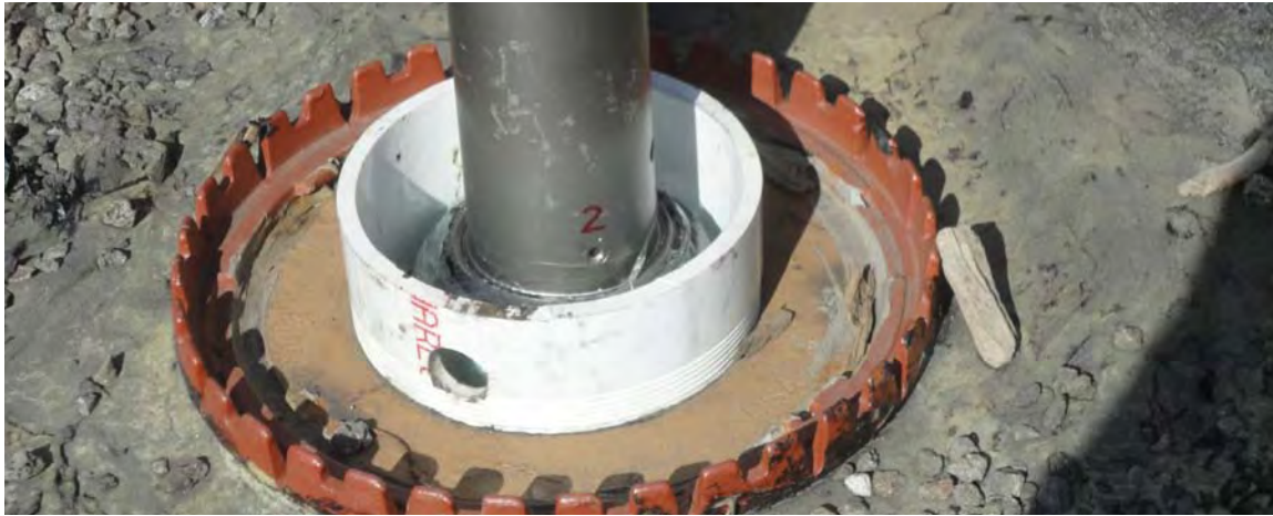
Figure 4-10: The orifice in this controlled flow drain sets the ponding depth and controls the out-flow from the roof on DEP's Storage Facility in Brooklyn.
