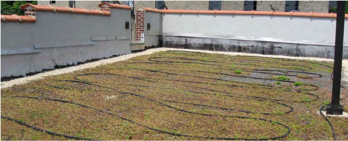
Figure 4-19: Drip irrigation on a constructed green roof at Fordham Bedford Housing in the Bronx.
