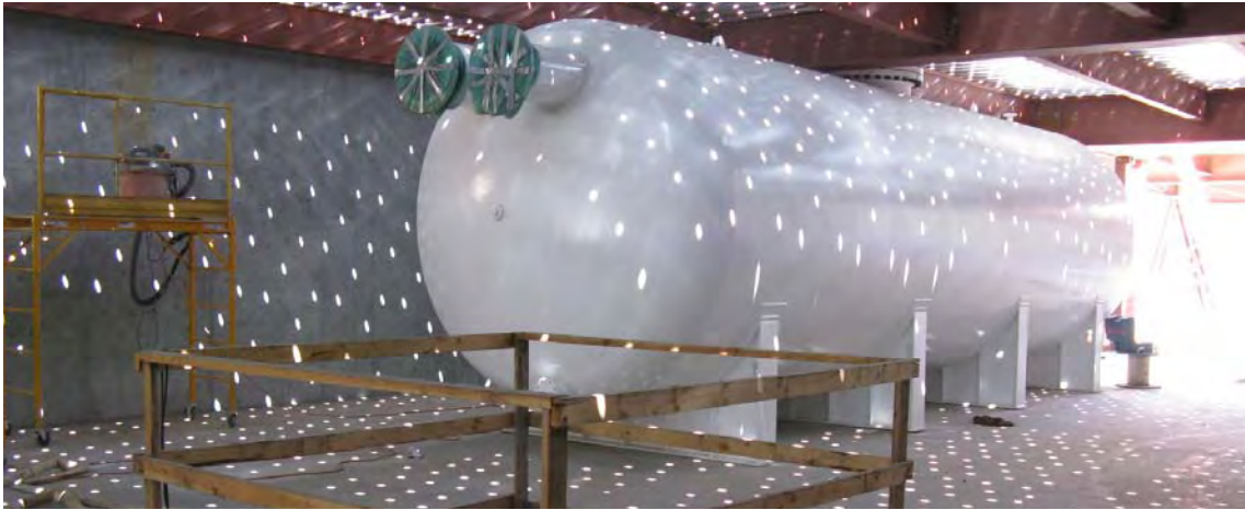
Figure 5-1: A 10,000 gallon tank at Remsen Yard used to store rooftop runoff to wash trucks and settle dust. The site, designed and constructed by DDC, also has a 72,000 gallon retention tank (not pictured), used to collect runoff from the entire site.
