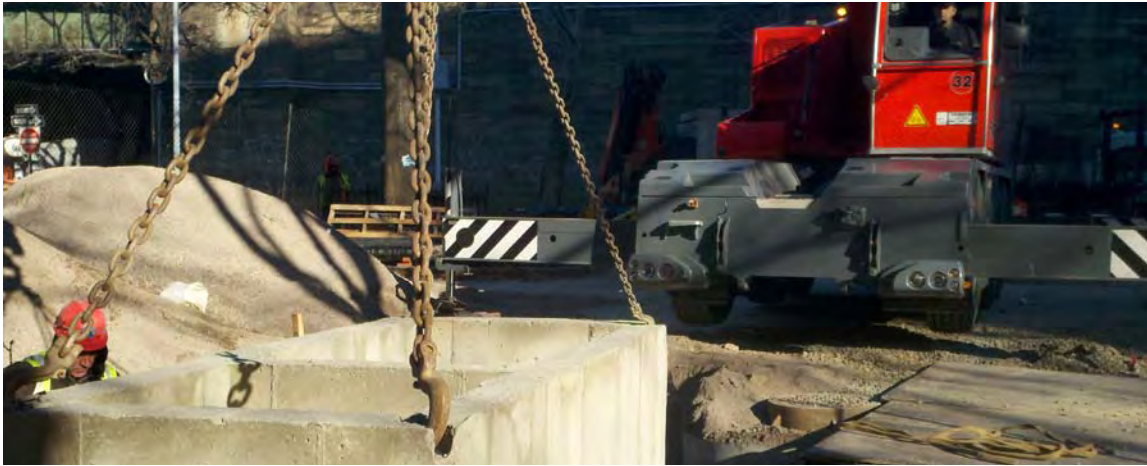
Figure 3-15: Pretreatment structures are typically installed after the geotextile and bedding stone is placed.
