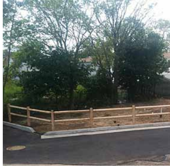
Figure 1-1: Stormwater chambers were installed prior to filling with soil for the construction of a constructed wetland at a DOT parking lot in Far Rockaway. The wetland area, to be planted in Spring 2012, will allow runoff to infiltrate directly into the subsurface system. The adjacent parking lot is paved with porous pavement and excess flow will be directed to the constructed wetland.
