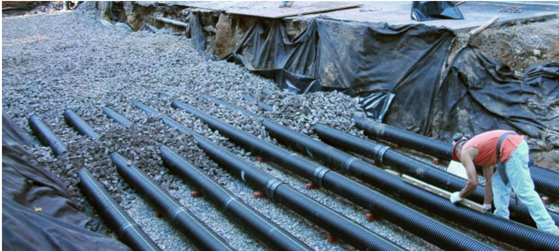
Figure 3-2: Construction of a perforated pipe system at NYCHA's Bronx River Houses in the Bronx.
