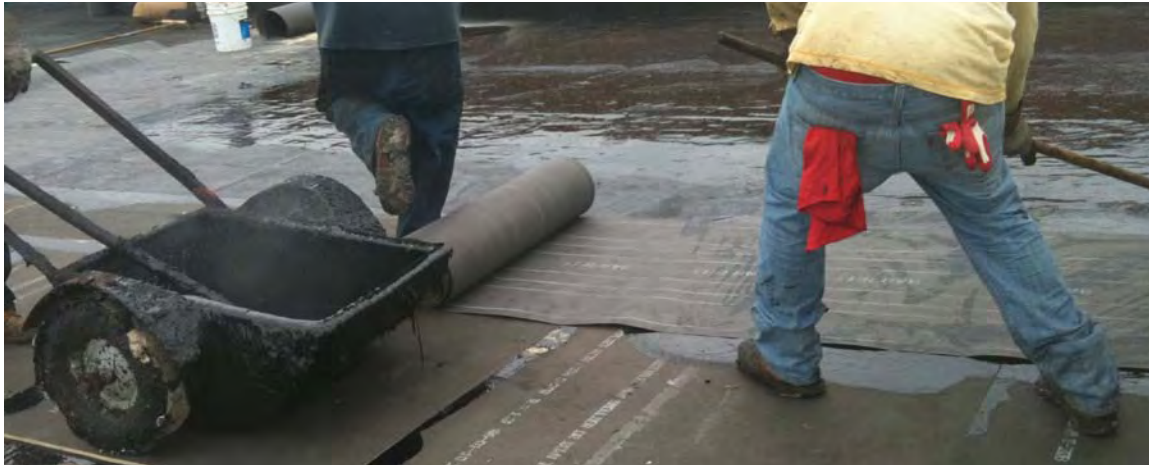
Figure 4-8: Installation of fiberboard and first ply of waterproofing membrane during construction of a blue roof at PS118 in Queens.
