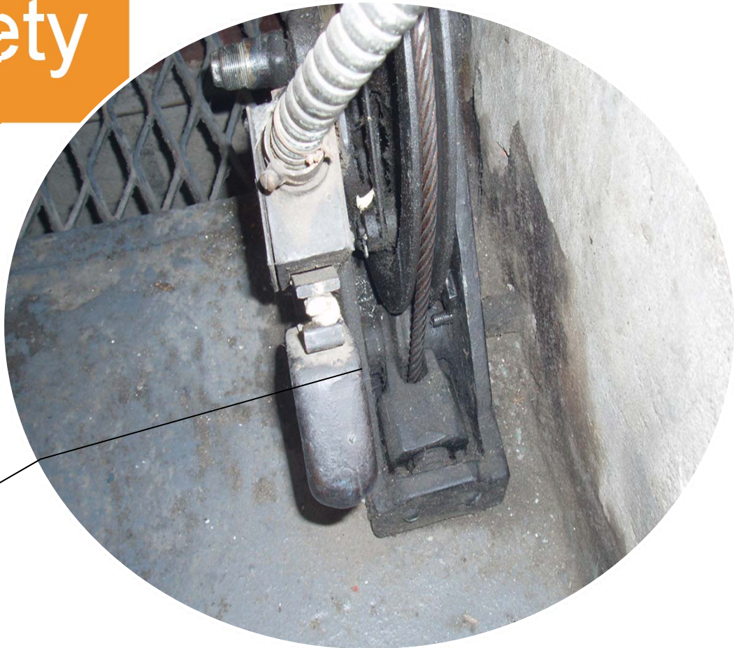
Governor switch blocked
