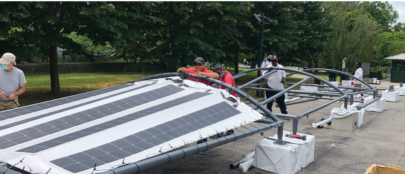
Installation of solar PV canopies at the New York Botanical Garden | Source: DCAS
