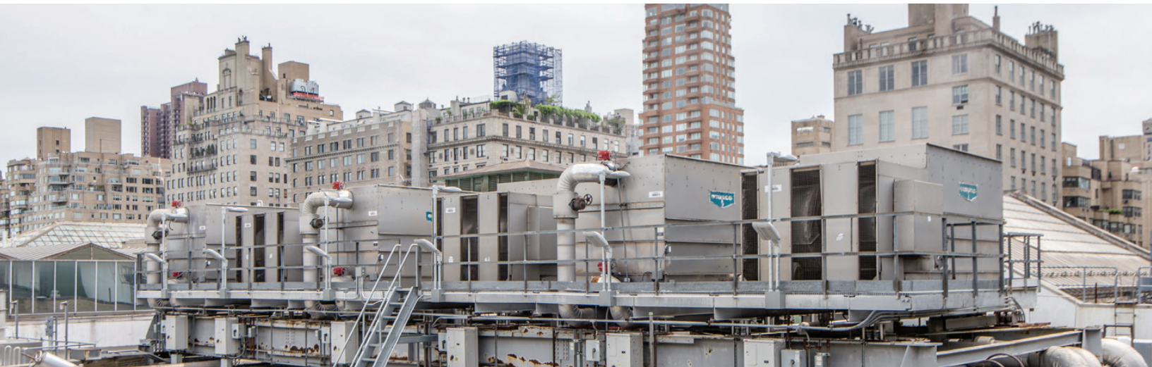
Cooling towers on roof of Metropolitan Museum of Art | Source: DCAS
