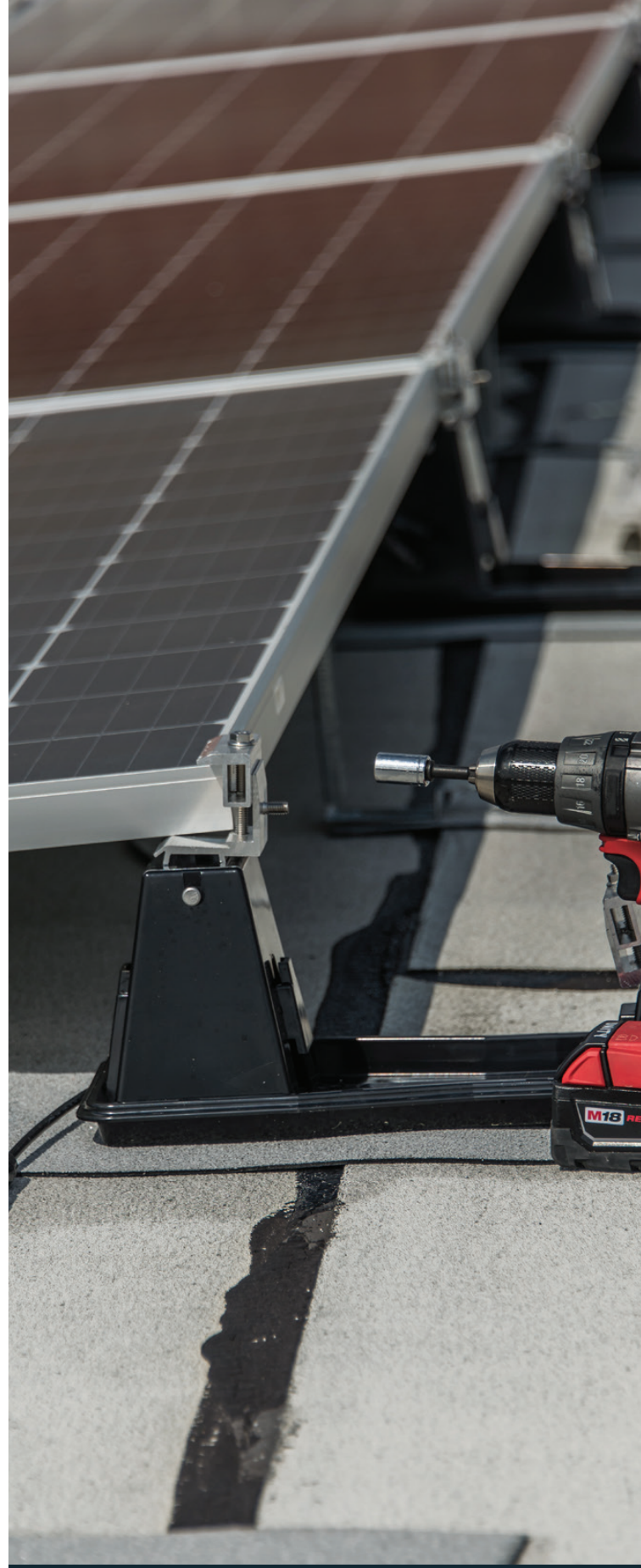
Solar installation on roof of Queens Junior High School 157 Stephen A. Halsey | Source: DCAS
