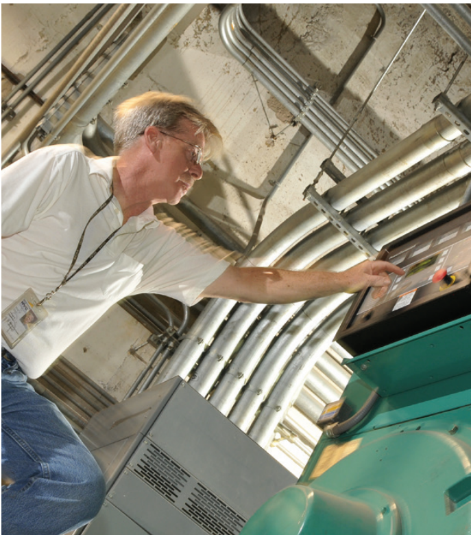
DCAS Facilities Management building operator examining building generator control panel Source: DCAS
