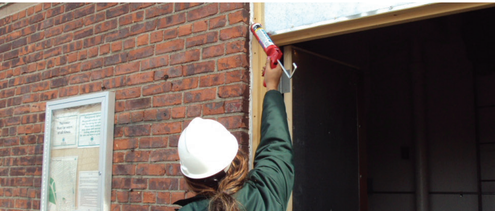
Department of Parks and Recreation staff weather-sealing a comfort station entrance | Source: DCAS
