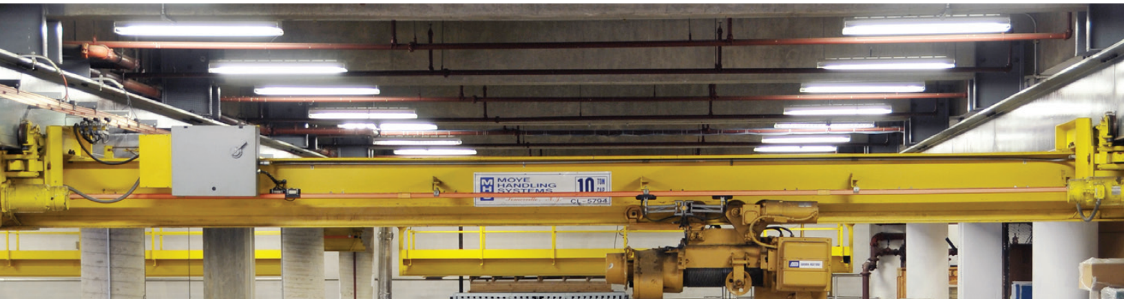
Lighting upgrades installed at the Staten Island Ferry Maintenance Facility | Source: DCAS
