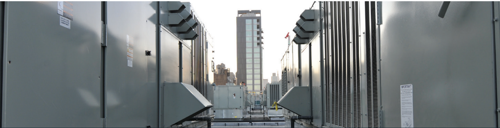
Rooftop air handling units on Department of Sanitation's 26th St Garage | Source: DCAS
