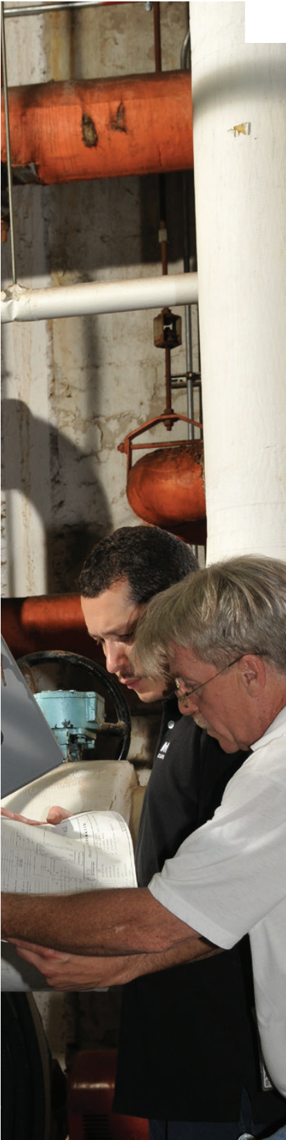
DCAS FM Building Operators examining building electrical systems.
