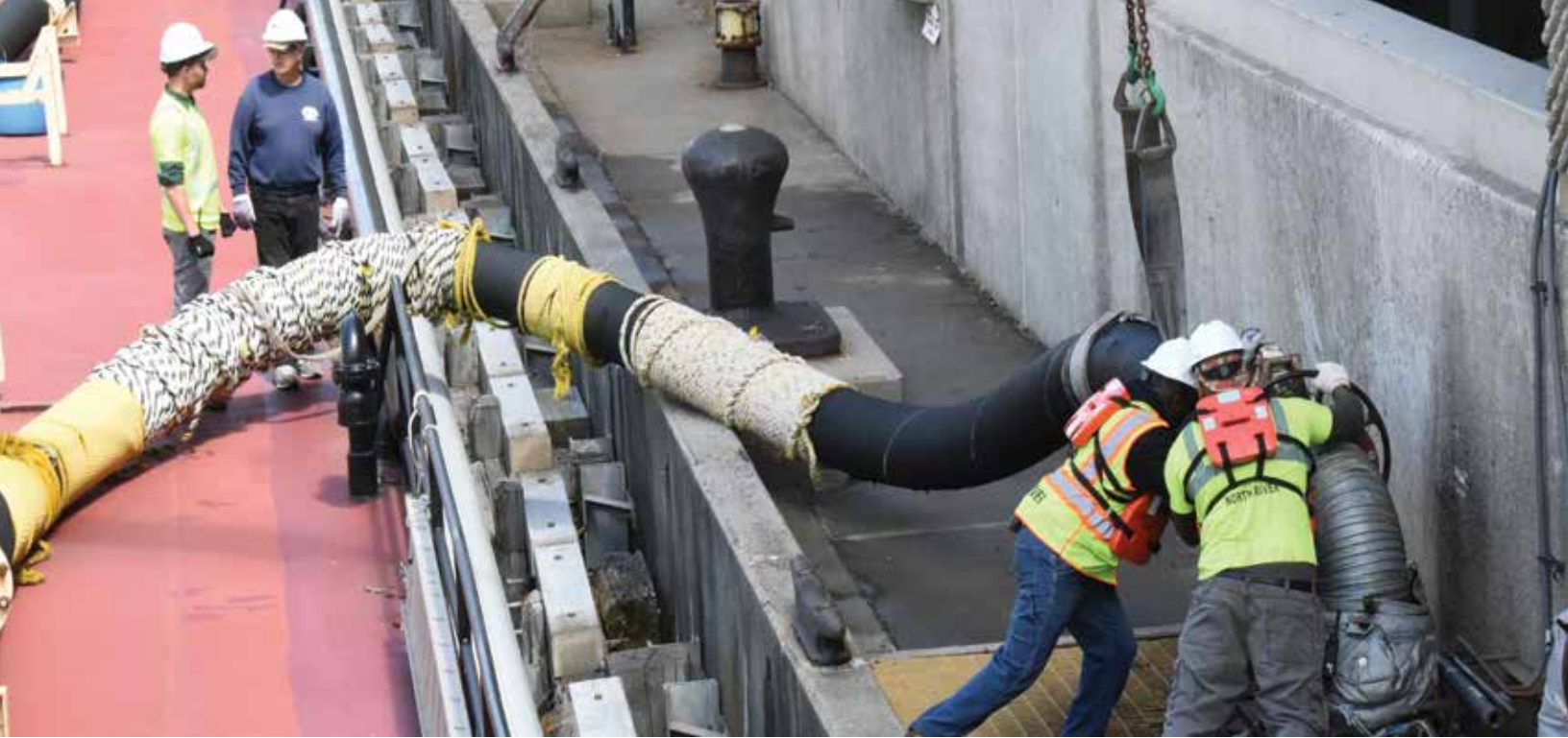
Sludge Delivery at North River Wastewater Treatment Plant
