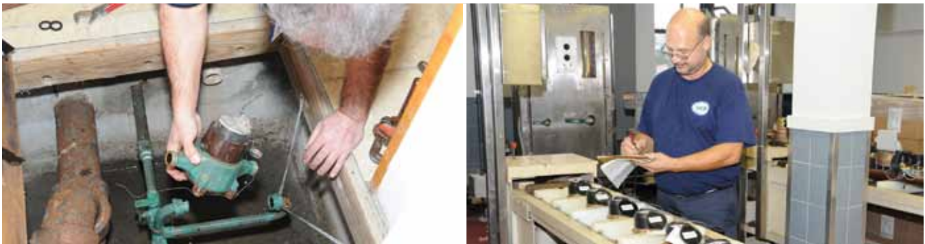
Replacing water meters on a regular basis is critical to ensure accurate consumption data and billing information.
