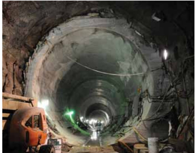
Mayor Bloomberg has made finishing City Water Tunnel No. 3 a top priority, investing more funds for the tunnel than the previous five administrations combined.
