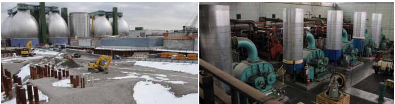
Recent investments, including those at the Newtown Creek Wastewater Treatment Plant, will help DEP meet mandated treatment standards in 2011.
