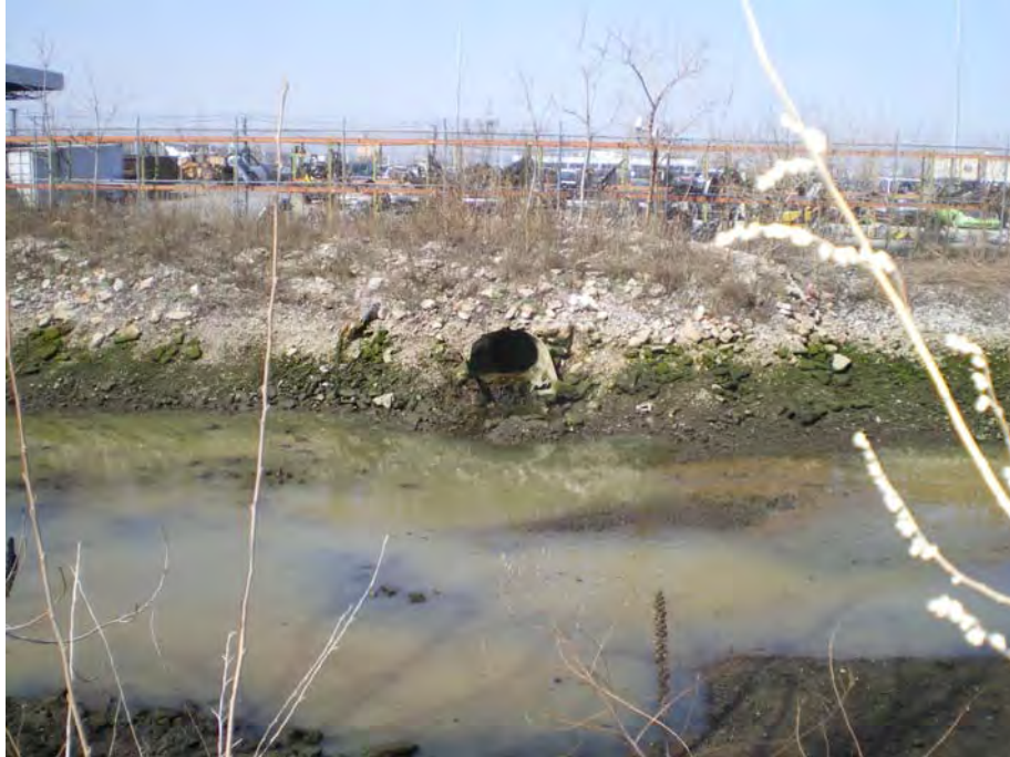
Site Photograph 5-8: Outfall into drainage ditch from western portion of NYPD Tow Pound.
