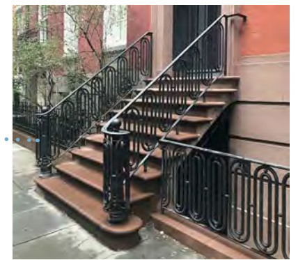
BROWNSTONE STOOP TO MATCH 278 WEST 11TH ST. (PROPOSED RAILINGS NOT SHOWN ABOVE)
