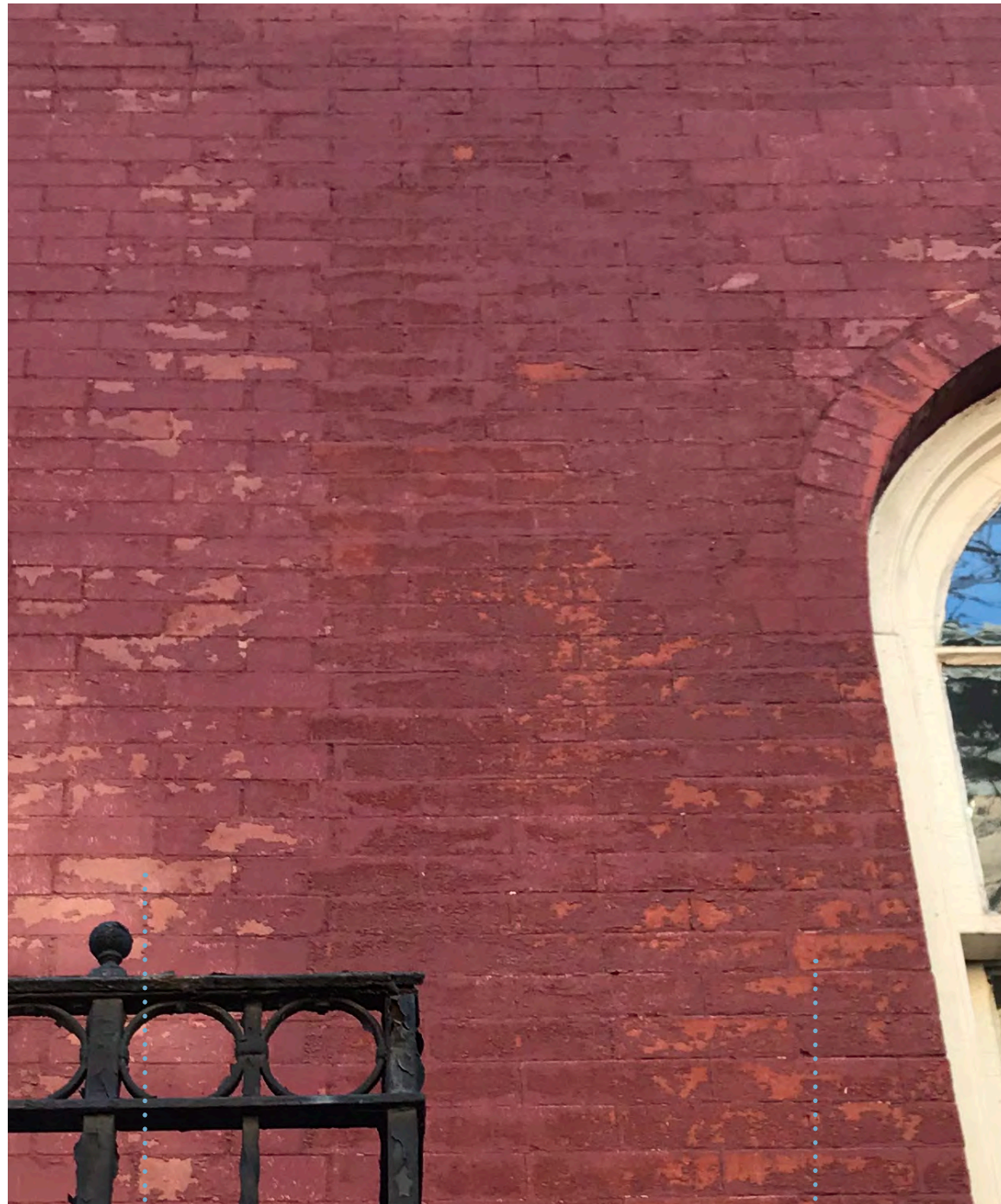
BRICK FROM 1924 CONVERSION VISIBLE BELOW PEELING PAINT
