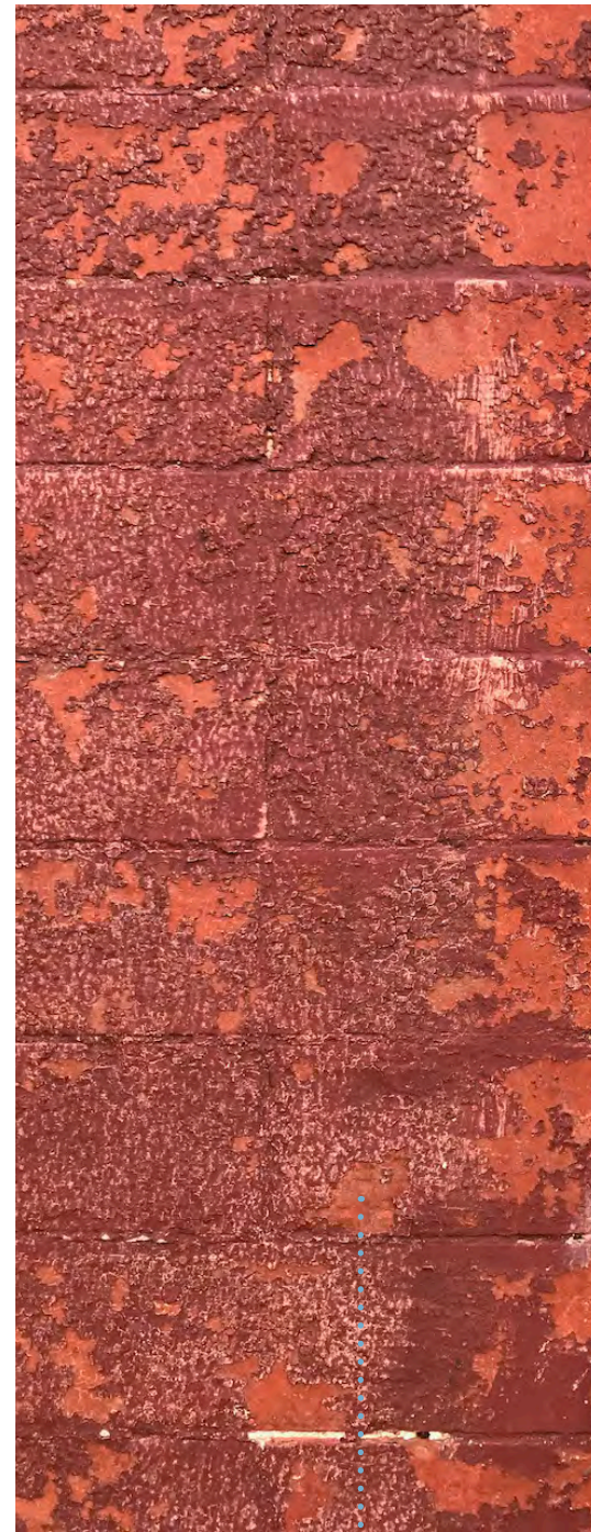
ORIGINAL BRICK VISIBLE BELOW PEELING PAINT
