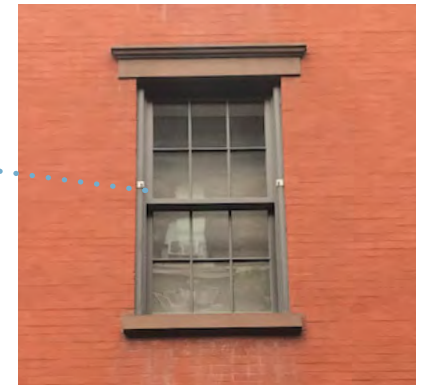
CAST STONE LINTELS AND SILLS TO MATCH 278 WEST 11TH ST. LIGHT PAINTED DOUBLE HUNG WINDOWS (PROPOSED WINDOW COLOR NOT SHOWN ABOVE)
