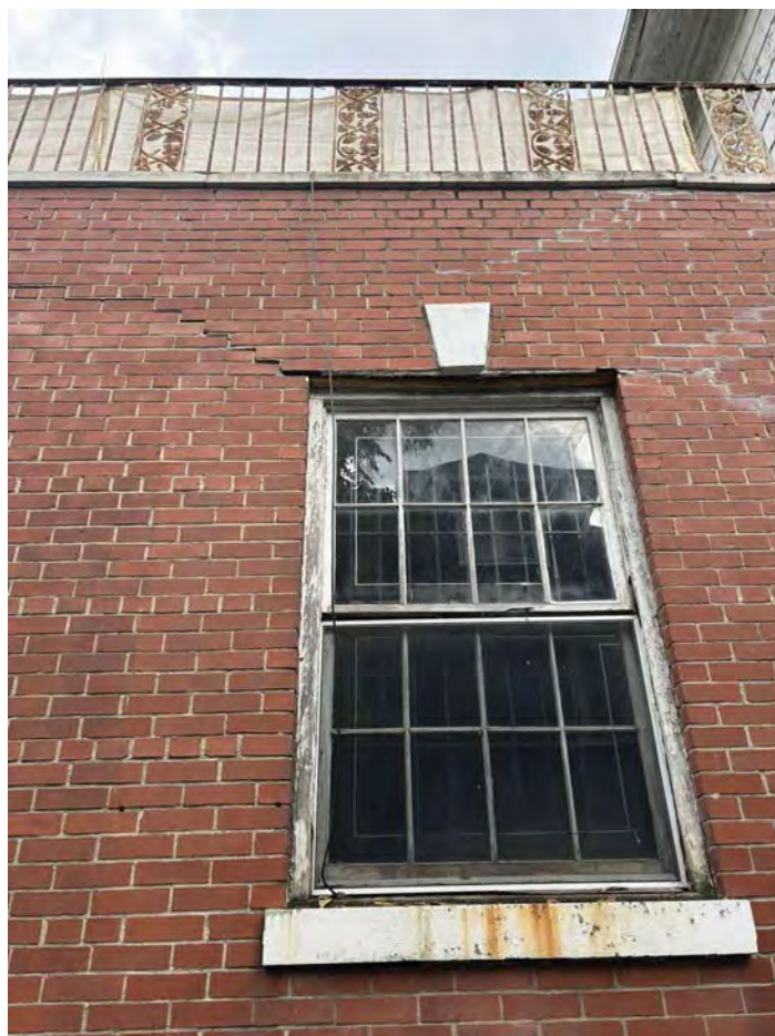
STAIR-STEP BRICK WALL CRACK
