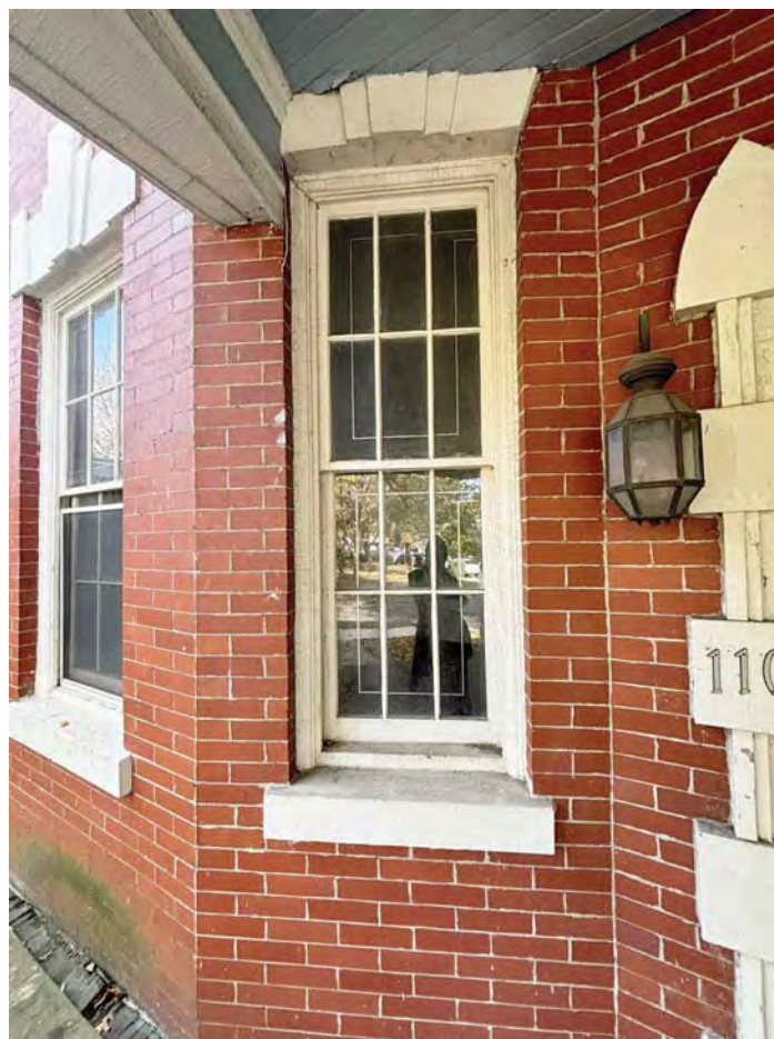
BEAM/WINDOW LINTEL CONFLICTION
