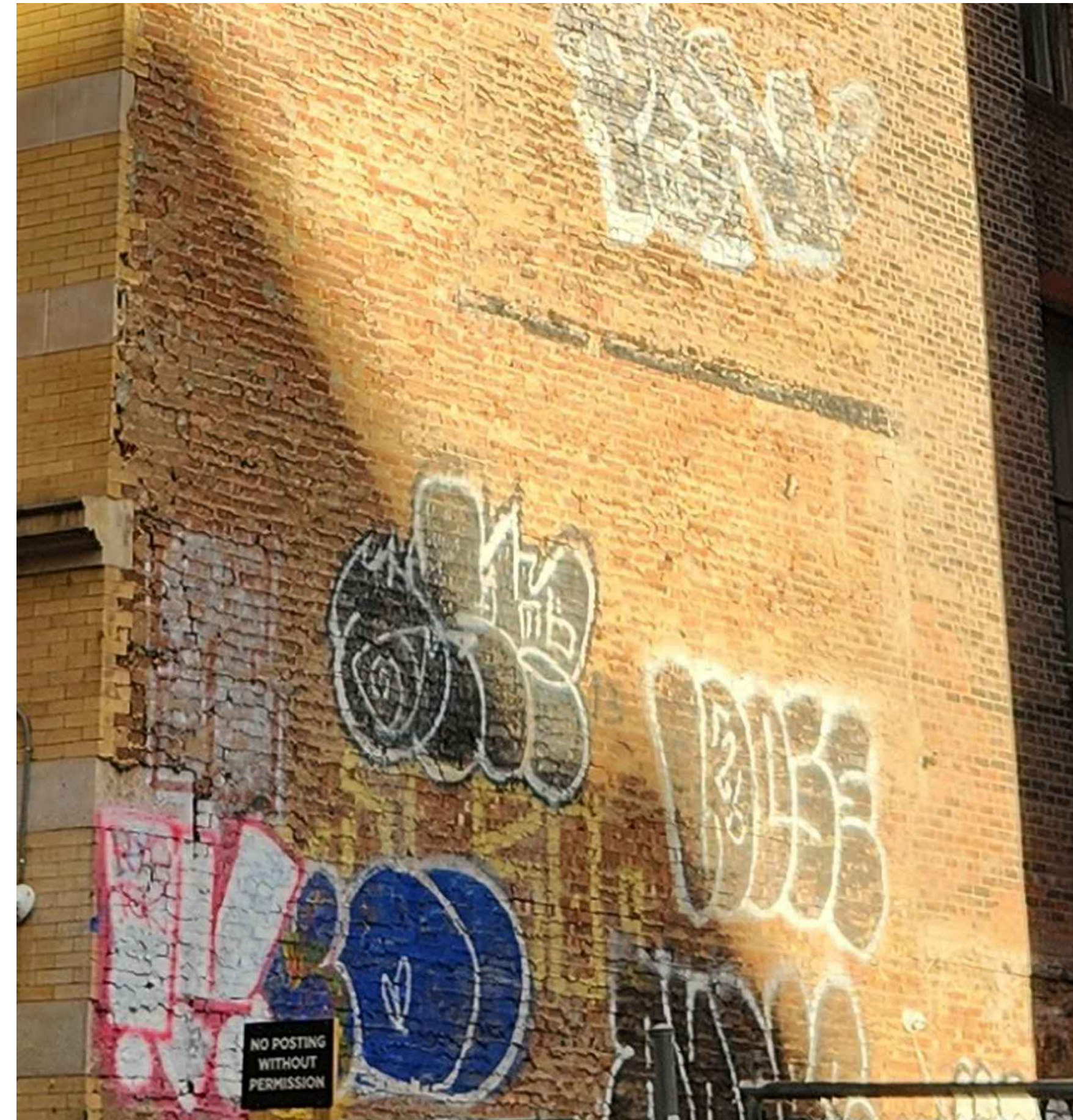
2 SOUTH ELEVATION, GRAFFITI AND OPEN JOINTS
