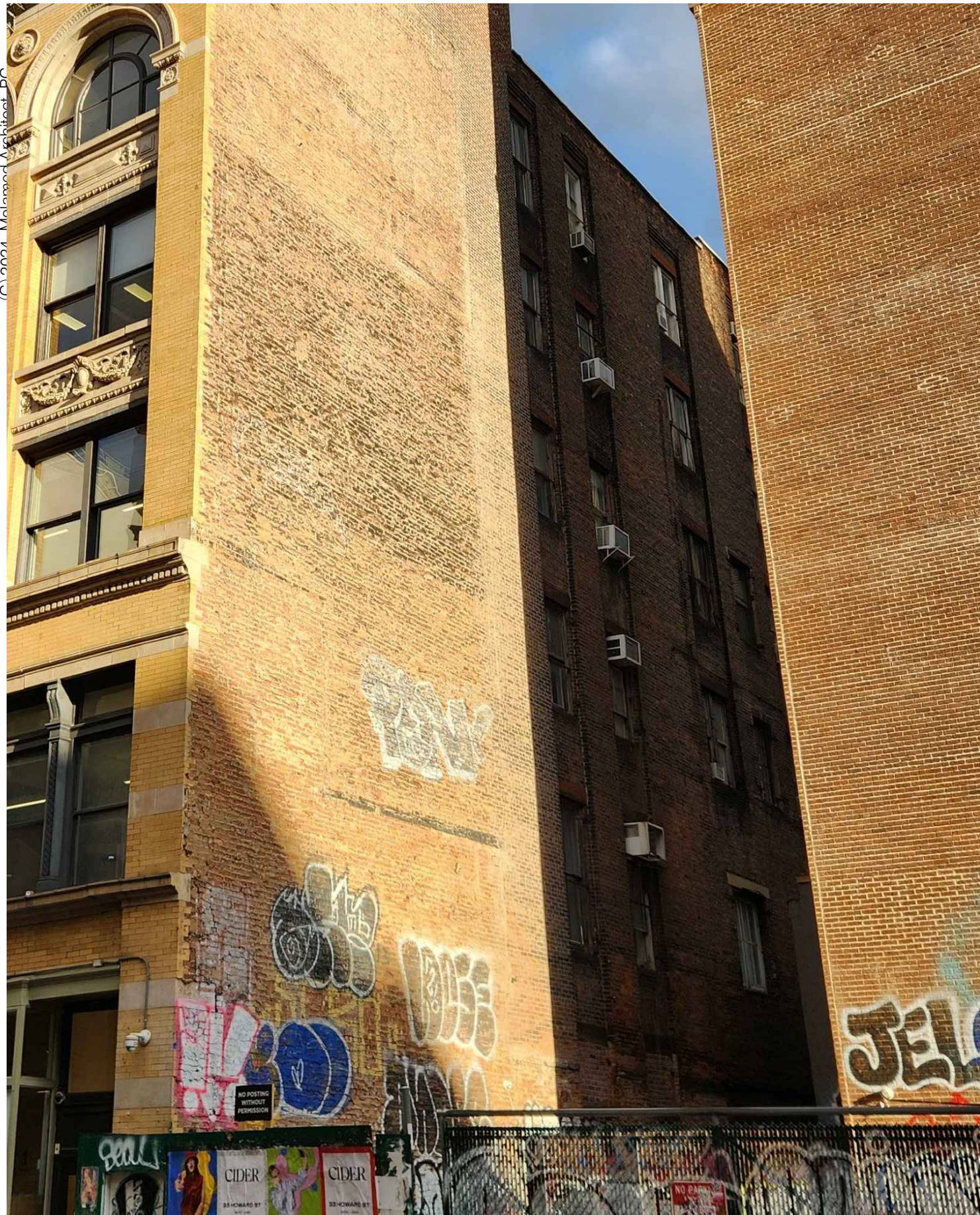
1 SOUTH ELEVATION, GRAFFITI & OPEN JOINTS
