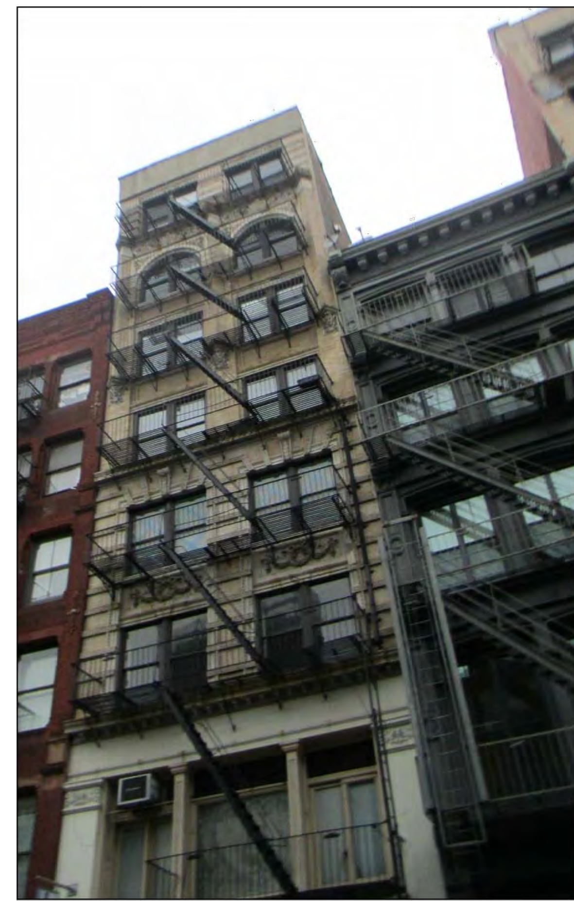
9 METAL FIRE ESCAPES
