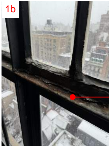
Rust through historic steel
