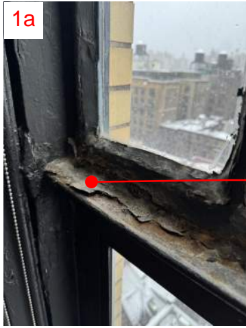
Rust through historic steel
