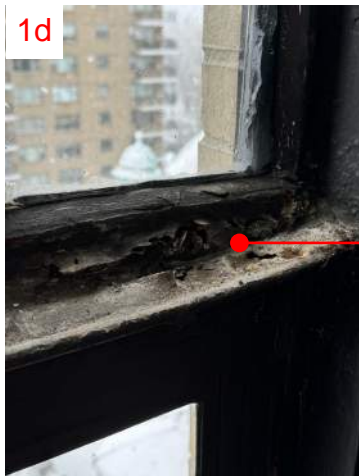
Rust through historic steel
