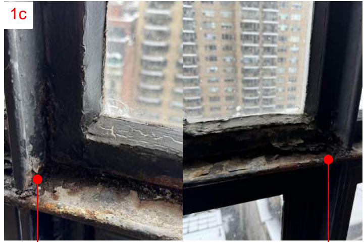
Rust through historic steel structural members
