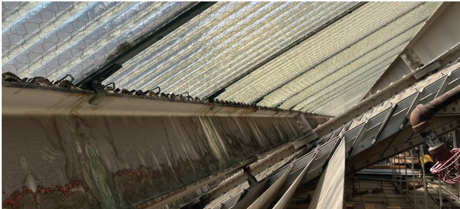
1 EXISTING WING J SKYLIGHT DETAIL SHOWING RUST DUE TO LEAKS
