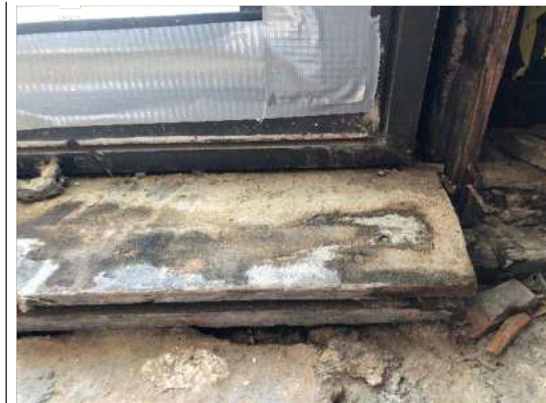
THE LEVEL OF DECAY OF THE TIMBER REVEAL ENCAPSULATING THE WINDOW ASSEMBLY IS EXTREME AND REQUIRES IMMEDIATE REMOVAL.
