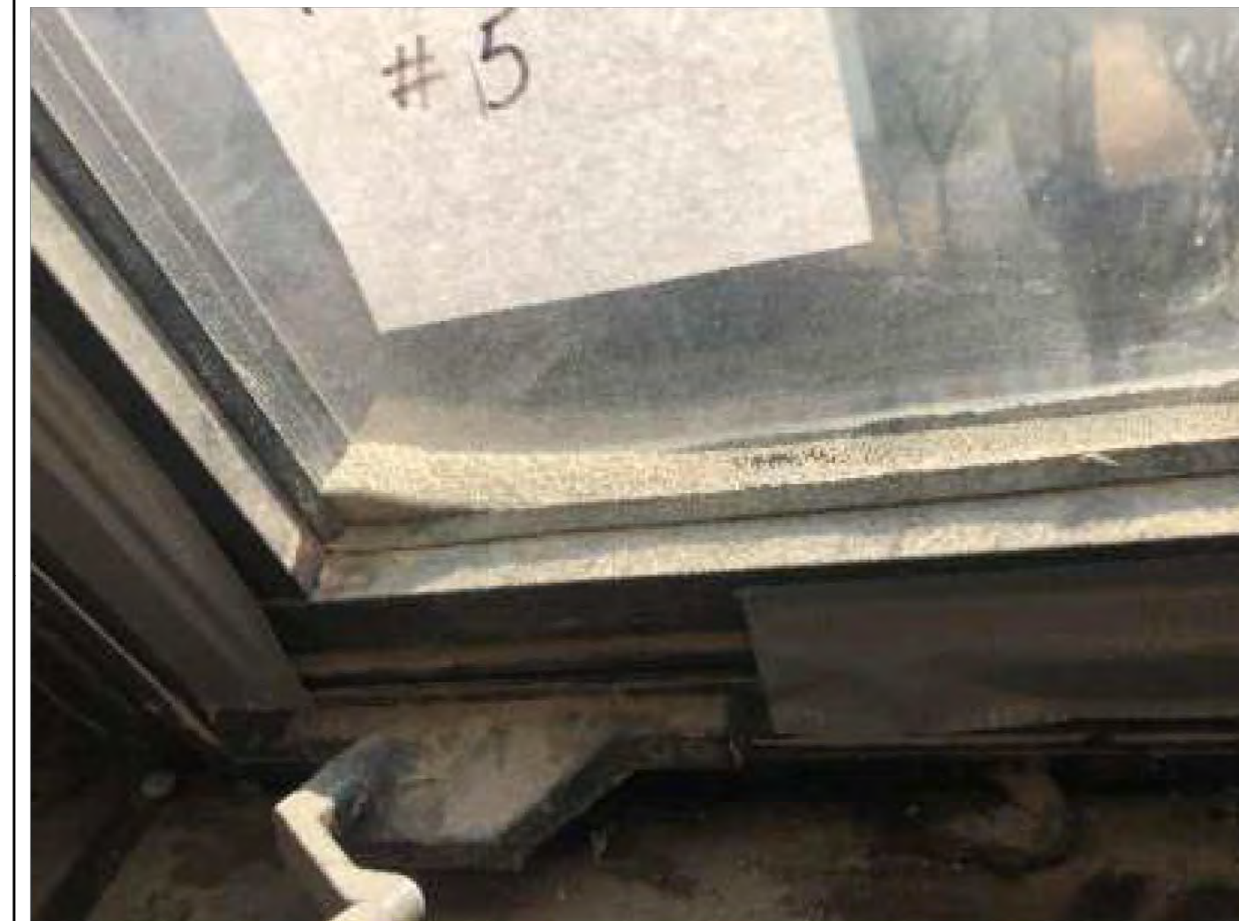
THE LEVEL OF OXIDIZATION TO THE WINDOW SNAP BEADS DEMONSTRATES THE INFILTRATION OF THE GLAZING CAVITY.
