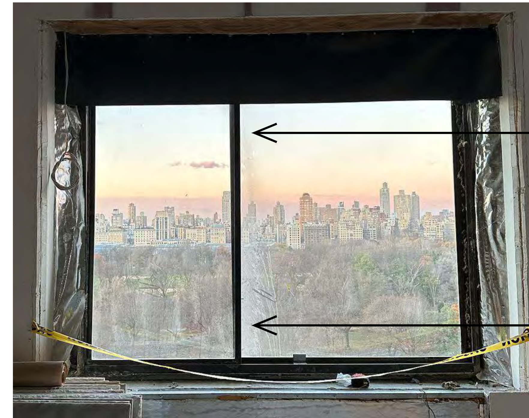
WINDOW LEANS FORWARD, THIS IS WHY THE MULLION LOOKS WIDER & CLOSER AT THE TOP
