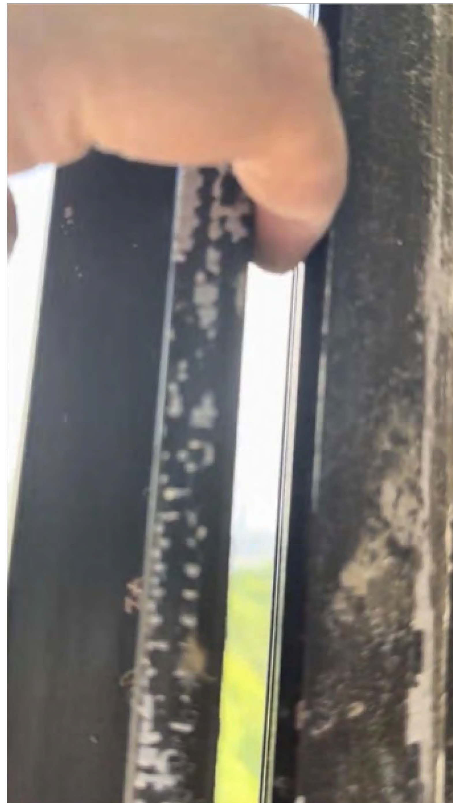
WRACKED FRAMES WITH GAPS EVEN WHEN CLOSED
