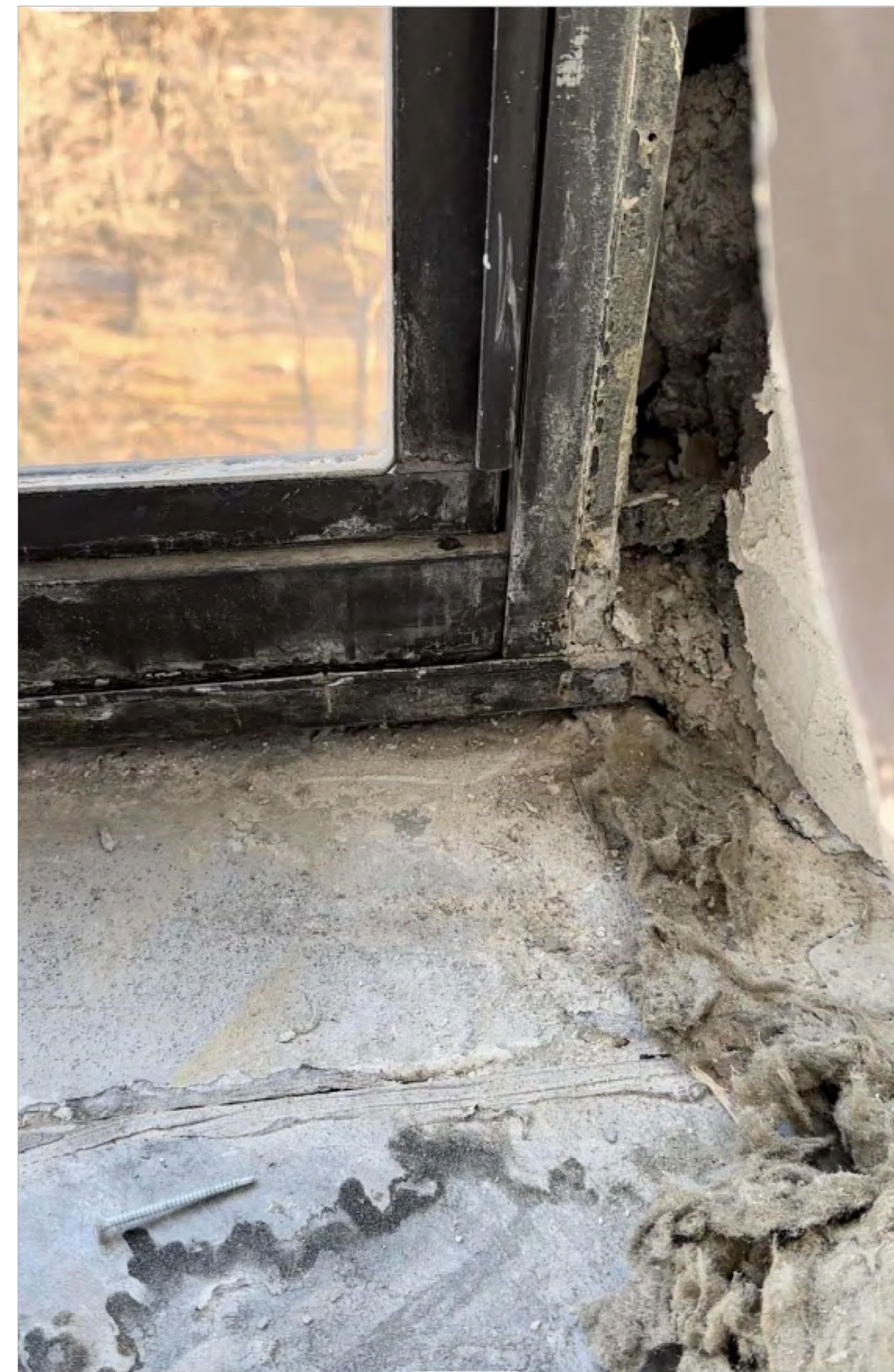
CORROSION & OXIDATION OF FRAMES FROM WATER EGRESS, THROUGH ALL WINDOWS
