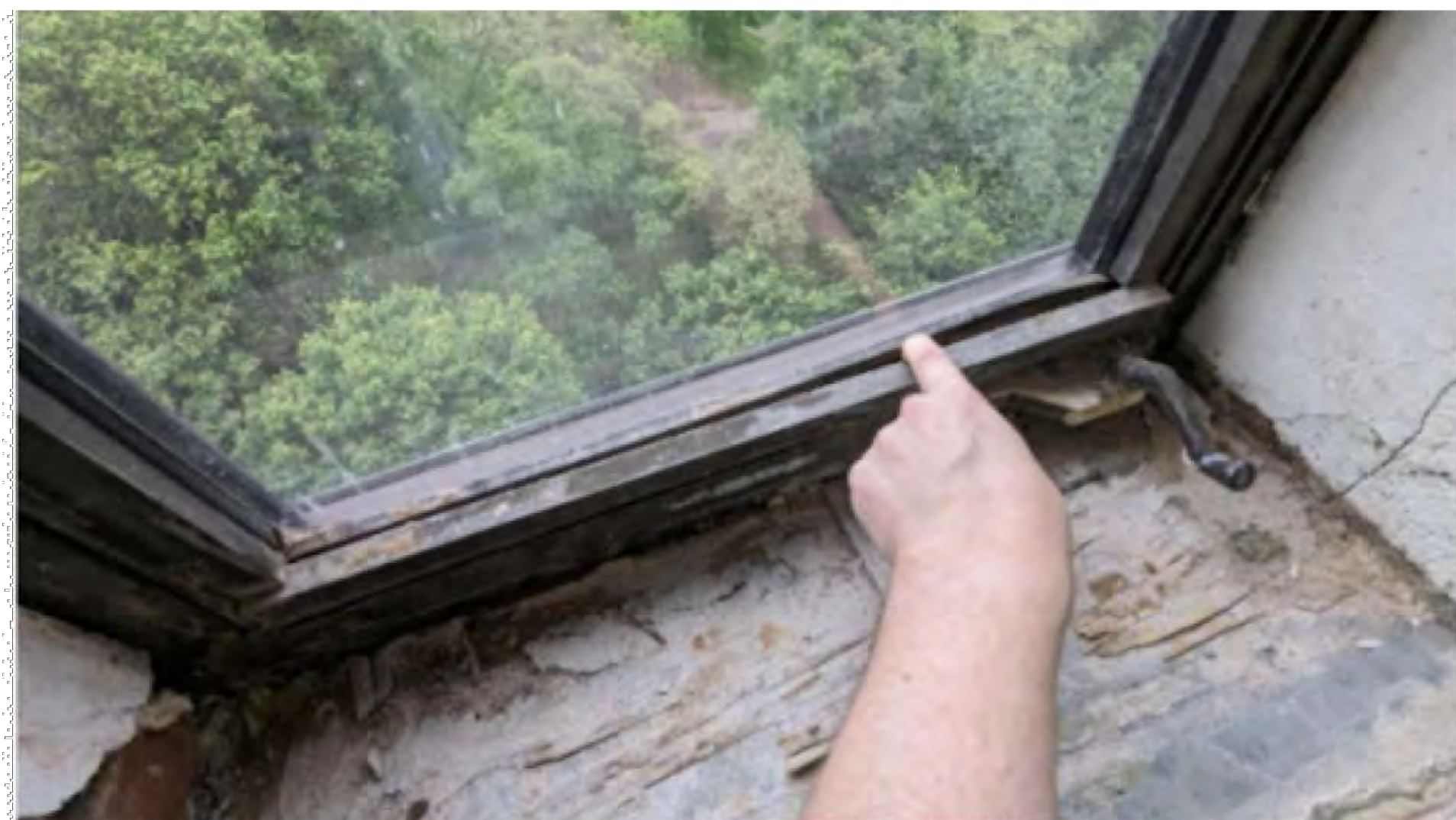
THE GASKETING AND GLASS STOP AT THE WINDOW SASH FRAME OF WINDOW WAS VISIBLY LOOSE AND ABLE TO REMOVED BY HAND.
