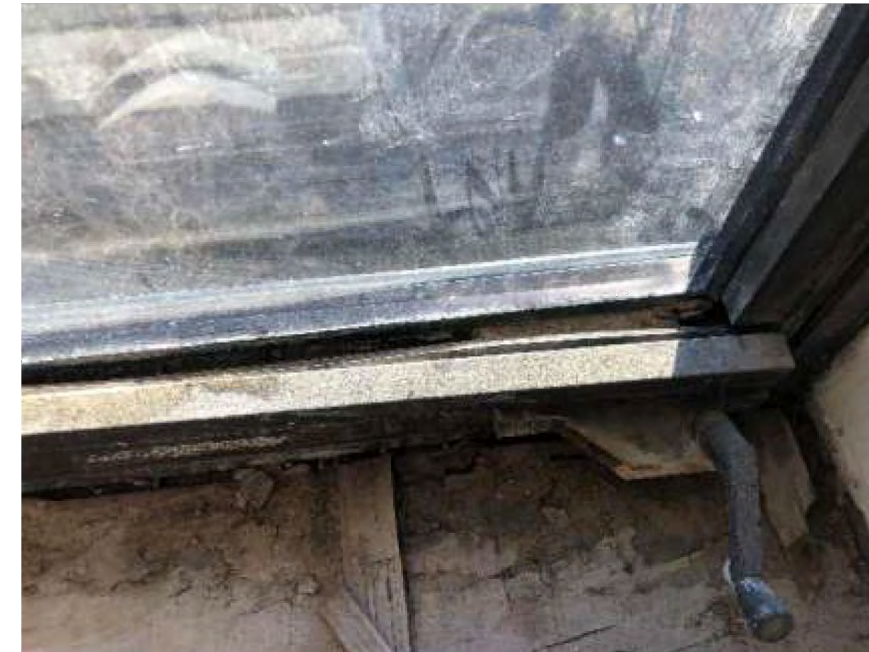
FRAME SNAP PROFILE HAVE BROKEN, MOST LIKELY DUE TO WATER PENETRATION AND OXIDIZATION.
