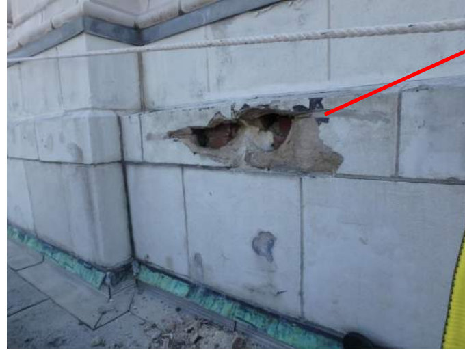
PHOTO # 1: West Elevation Main Roof Close-up photo of main roof spalled terracotta.
