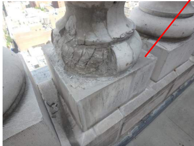
PHOTO # 2: West Elevation Main Roof Close-up photo of spalled precast balustrade at perimeter of main roof. Photos by CANY
