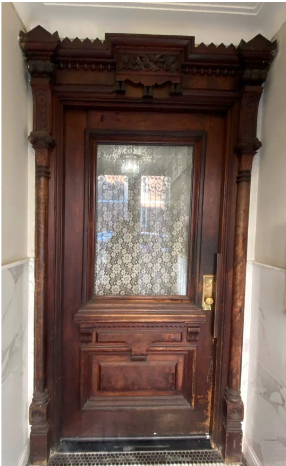
Photo of the existing vestibule door with upper glazed pane and lower raised wood panel. The clear width of the vestibule door is 3'-3".
