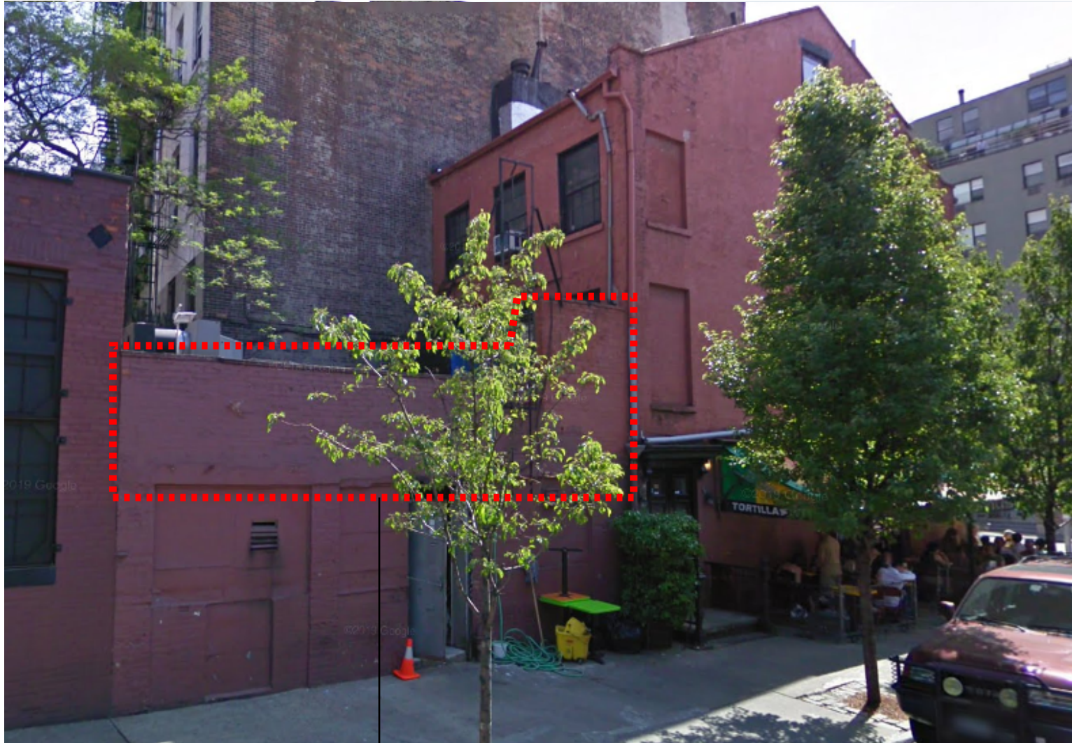
Rear Addition as of 2018, before Copping, parapet and stone lintel removed under #CNE-132234
