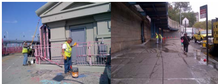
May 2014: Bridge Painter Russell Newme, Supervisor Bridge Painter Cesar Pazmino, Bridge Painters Goncalo Lima and Samuel Martinez, and Supervisor Bridge Painter Robert Avellino Removing Graffiti From the Williamsburg Bridge. September 2014: Supervisor Bridge Painter Cesar Pazmino and Bridge Painter Goncalo Lima Removing Graffiti From the Manhattan Bridge Market Place. (Credit: Earlene Powell)
