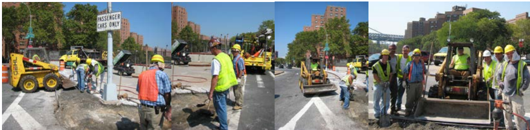
Sidewalk Repairs in August 2010 at Houston Street Bridge over the FDR Drive: Tractor Operator Robert Noordzy (in Tractor), Bricklayer Vincent Sciulla, Cement Masons Frank Finizio and Victor Porowski, and Bricklayer Luigi Cuffari. Bridge Repairer and Riveter Brook Budd and Bricklayer Luigi Cuffari. Tractor Operator Noordzy (in Tractor), Cement Masons Frank Finizio (Foreground) and Victor Porowski (Background), and Bricklayer Vincent Sciulla. Bricklayer Vincent Sciulla, Bridge Repairer and Riveters James Philip and Brook Budd, Bricklayer Luigi Cuffari, Tractor Operator Robert Noordzy, Supervisor Bricklayer Edward Alfano, and Cement Masons Frank Finizio and Victor Porowski. (Credit: Russell Holcomb)
