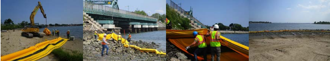
Installation of a Turbidity Curtain to Protect the Shore During Construction of the Temporary City Island Bridge in 2014.
