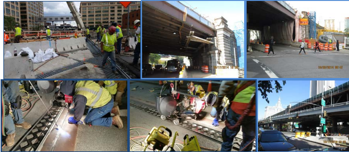
October 2014: Sands Street Structure – Preparing for Closure Pour. Containment Installation at Brooklyn Approach Structures. October 2014: Franklin Square Structure – Deck Alignment and Welding. Painted Manhattan Ramp.
