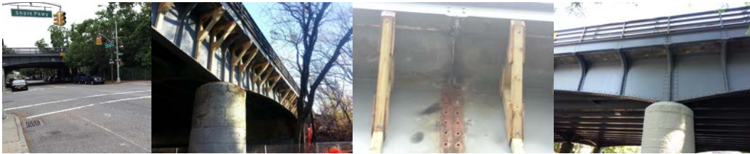
Replacing Deteriorated Fascia Brackets From the North and South Girders of the Belt Parkway Bridge Over Bedford Avenue. Temporary Supports Were Installed at the Bracket Location. Bracket was Removed. New Brackets Were Installed and Painted. (Credit: Vadim Sokolovsky)
