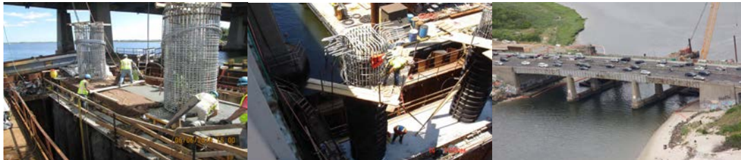
Finishing and Covering Plinth Concrete at Pier #1 in June 2014. Setting Rebars and Forms for Columns at Pier #2. Jamaica Bay at Left. Construction Barges and Cranes Constructing new Piers #1 and #2. Eastbound Traffic at Bottom.
