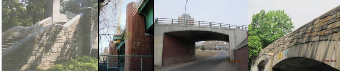
Abutment Wingwall Cladding on the West 173 rd Street Bridge. Hutchinson River Parkway Bridge. Brooklyn-Queens Expressway Over Ramp to Brooklyn-Queens Expressway (Eastbound). Right Side Fascia on the Bronx Pelham Parkway Bridge.
