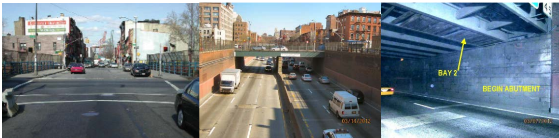
Union Street Bridge. March 2012: Right Elevation. Timber Shielding in Bay 2 of Span 1. (2012 Credit: NYSDOT)
