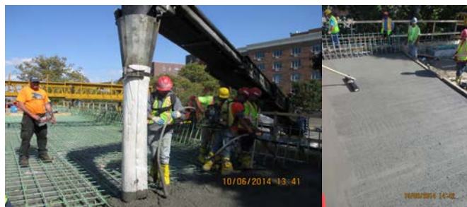
October 2014: Placing and Vibrating the Concrete Deck at the Bridge Facing West. Applying a Broom Finish Texture to the Deck Concrete.
