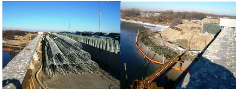
January 2014: Rebar Cages for Cast-in-Place Piles Temporarily Stored on the North Side of the Gerritsen Bridge. Northeast Abutment Wall Formwork and Rebars. Turbidity Curtain in Place at Work Site. Existing Bridge at Right.
