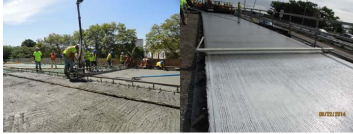
Screed at East 8 th Street Ramp in 2011, and at West Approach of Gerritsen Inlet Bridge in 2014.
