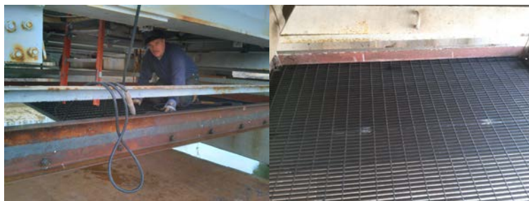
March 2014: Bridge Repairer & Riveter Daniel Jederlinic Welding New Steel Grating and Support Framework on the Rikers Island Bridge. (Credit: Steve Havemann)
