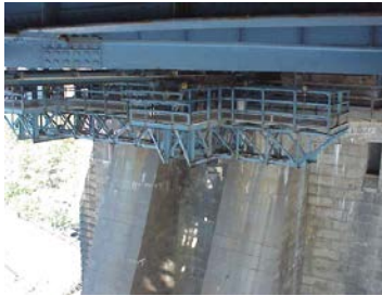
Manhattan Bridge Traveler. (Credit: NYSDOT)
