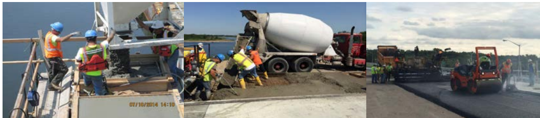
July 2014: Bottom Dump Bucket Used to Place Concrete for Pedestals at Pier #1 Cap Beam. Placing PCC Pavement at East Approach. Spreading and Compacting Hot Mix Asphalt on Belt Parkway East Side of Bridge.
