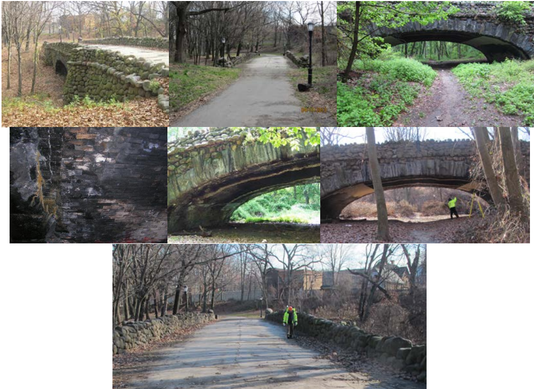
Highland Park Bridge. Dirt Pathway Under Bridge. Under-Deck Cracks and Missing Bricks - North-East Side. Under-Deck Arch Wall Showing Efflorescence Along the Cladding Stone and Brick Arch. Inspecting the Bridge in December 2014.
