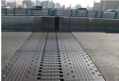
Manhattan Bridge Finger Dam. (Credit: Jagtar Khinda)
