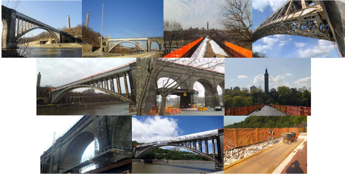
Northern and Southern Views of High Bridge in 2013. Winter 2013: Installation of Safety Shield Materials on the Walkway. Winter 2013: Safety Cables Installed on the Bridge. Early Spring 2013: Temporary Work Platform on the Bridge. Temporary Work Platform on Sedgwick And Undercliff Avenues. Spring 2013: Mast Climber and Lead Abatement Containment on the Bridge. Summer 2013: Brick Paver Removal. (Credit: NYCDDC)
