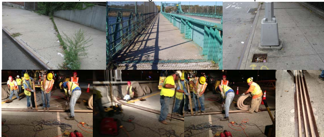
August, October, and November 2008: Examples of Tripping Hazards. July 2013 Safety Flag: Ironworker and Mason Crews Repairing Missing Joint Seal Materials on the Brooklyn-Bound Williamsburg Bridge. The Joint Sealer Spaces Were Widened on Each Part of the Joint Utilizing the Shop-Made Jack Expansion Blocks, and Then Completely Cleaned With a Needle Gun to Prepare the Surface to be Rough Contacted With Epoxy Glue. After the Glue was Spread on the Sealer Space Surfaces, the Seal Strip was Installed and Tightened. (Credit: Hany Soliman)
