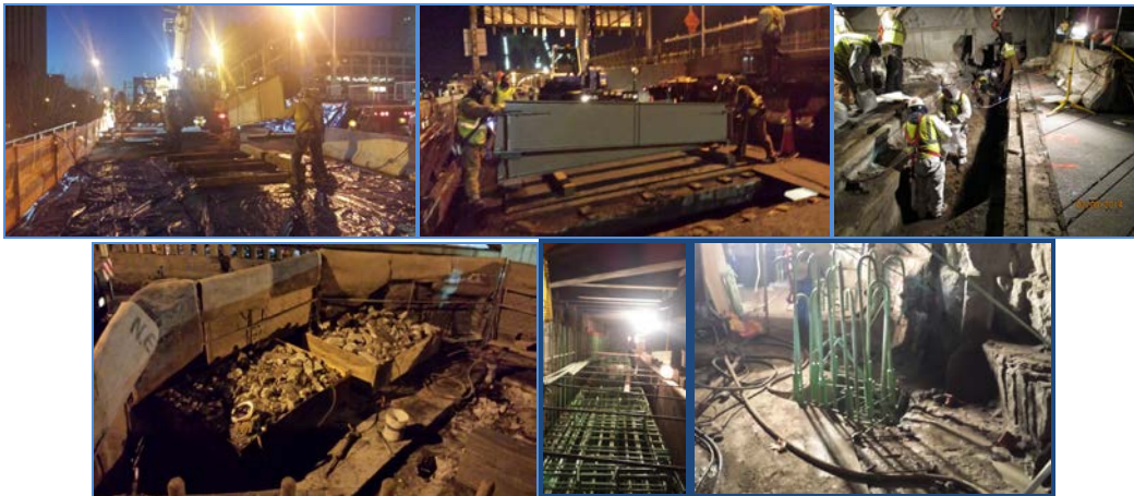
February 2014: Fascia Removal – Park Row Structure. Franklin Square Structure – Floorbeam Installation. York Street Structure – Demolition and Steel Removal. Main Street Structure – Cap Beam Installation.
