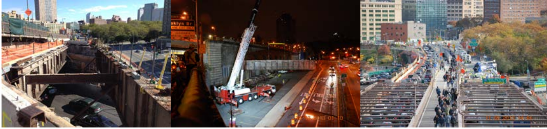
October 2013: Eastbound Brooklyn-Queens Expressway Traffic Flowing Under the Exposed Steel of the Eastbound York Street Structure. Removing the Fascia Steel From the Eastbound York Street Structure. November 2013: Concrete Placement at the Eastbound York Street Structure.
