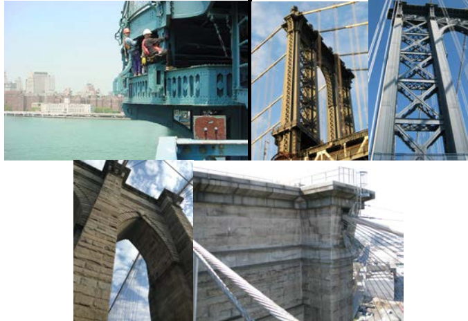
Inspectors on Manhattan Bridge Tower. (Inspector Credit: NYSDOT) Manhattan Bridge Tower. (Credit: Michele N. Vulcan) Manhattan Bridge Tower Detail. (Credit: Russell Holcomb) Brooklyn Bridge Tower. (Credit: Earlene Powell) Brooklyn Bridge Brooklyn Side Tower Detail. (Credit: Jagtar Khinda)
