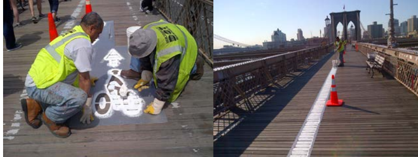
May 2014: Bridge Painters Jamie Andrade and Goncalo Lima Refreshing the Bicycle Path Markings. June 2014: Bridge Painter Brian Kavanagh Reapplying the Brooklyn Bridge Line Striping. (Credit: Earlene Powell)
