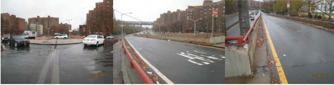
2011: Main Bridge – Top of Deck Looking West. South Approach Ramp – Top of Deck Looking South. North Approach Ramp – Top of Deck Looking North.
