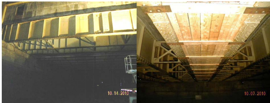
West 79 th Street Bridge Over Amtrak in 2010. Underside of Bay 7. (Credit: NYSDOT)
