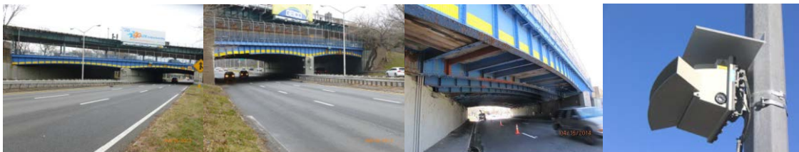
Westchester Avenue Bridge Elevation Left and Right in 2012. (Credit: NYSDOT) April 2014: Span 2 – Deteriorated Areas Shielded With Planks. Overheight Sensor Unit on the Hutchinson River Parkway. (Sensor Credit: Roly Parroco)
