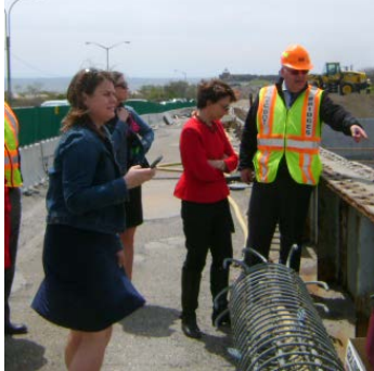
Pier 1 Plinth and Footing Inside the Cofferdam in May 2014. Commissioner Polly Trottenberg (in Red Jacket) and Chief Bridge Officer Robert O. Collyer Inspecting the Gerritsen Inlet Bridge Project in May 2014. (Credit: Moshin Rizvi)
