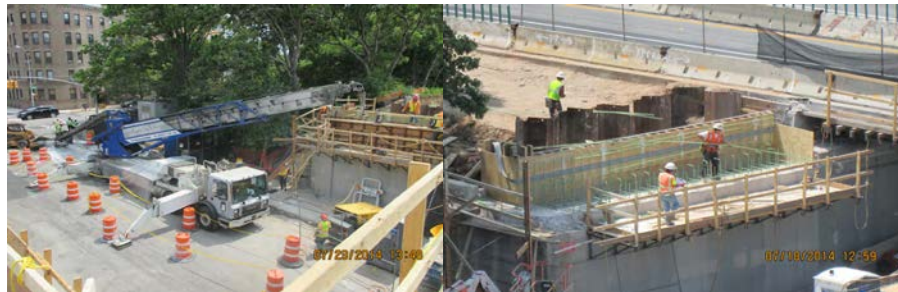
July 2014: Placing Concrete for Northeast Abutment Using a Conveyor. Setting Rebars at the Northeast Abutment.
