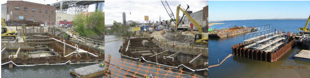
April 2010: Cofferdam With Filter Fabric and Gravel Placed Prior to Pile Driving During the Emergency Repair Project on the Borden Avenue Bridge over Dutch Kills. February 2011: Fresh Creek Cofferdam Pad.
