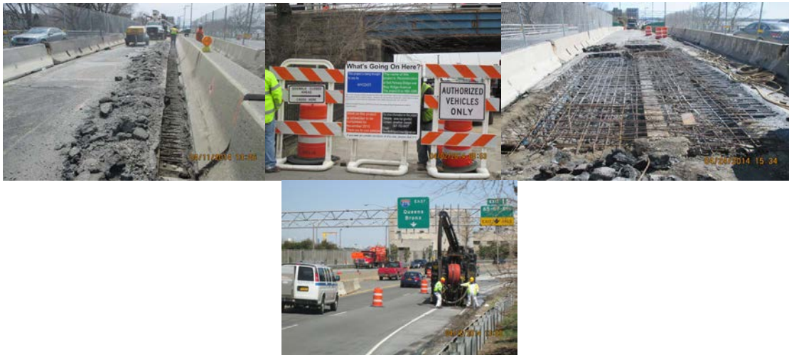
April 2014: Laborers Removing the Bridge Deck to Facilitate Removal of the Existing Concrete Median Barrier at Right Side of Trench During Stage I MPT. Stage I MPT Work Area After Removal of Structural Deck Concrete and Asphalt Wearing Courses, Exposing Deck Rebars and Structural Beams. Workers Cleaning out Catch Basins Using a High Pressure Water Hose and Vacuum Pipe for Debris Removal.
