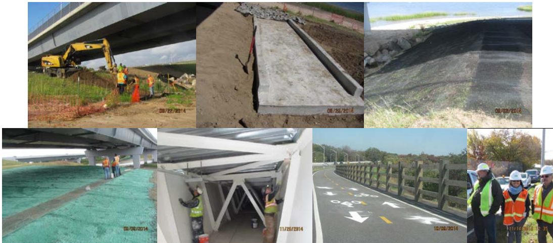
August and September 2014: Erosion Control at the Eastbound Paerdegat Bridge. Placing Fabric and Hydro-Seeding Under the Bridge. November 2014: Tub Girder Touchup Painting. October 2014: Bike Symbols on the Bicycle/Pedestrian Path East of Rockaway Circle. Three Rail Wood Fence. Associate Staff Analyst Kim Mulcahy, Civil Engineering Intern Jessica Wang, and Civil Engineer Reza Sharif at the Final Landscaping Inspection in November 2014.
