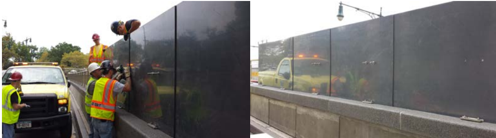
August 2014: Carpenters Stephen Buckley and William Sic, Supervisor Carpenter Joseph Vaccaro (in White Hard Hat), and Carpenters Gregory Nolan and Edward Alfano Jr. Testing the Installation of Polyvinyl Chloride Protection Boards Around the West Street Portal of the Battery Park Underpass. These Would be Placed in the Event the Coastal Storm Plan is Activated. (Credit: Paul Schwartz)
