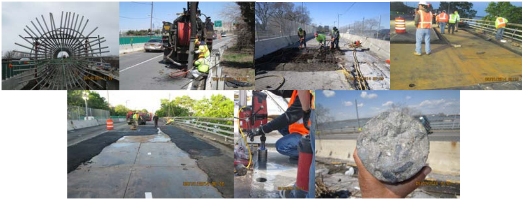
March 2014: Rebar Cage. April 2014: Workers Cleaning out Catch Basins Using a High Pressure Water Hose and Vacuum Pipe for Debris Removal. Pavement Breakers used to Demolish the Existing Bridge Deck During Preparation for Stage I MPT. May 2014: Temporary Deck Repair of Eastbound Roadway Using Steel Plates. Placing and Compacting Hot Asphalt Over Steel Plate Deck Repair at Eastbound Bridge. May 2014: Core Sampling.
