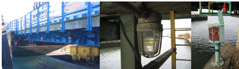
Inspection in Late 2012: Carroll Street Bridge - Navigational Fixtures on North Side of Span – Only the Center Span Fixture was Operational. Grand Street Bridge – Standing Water in the Access Light Fixture at the East Wedge Walkway. Typical impact damage to pier light.
