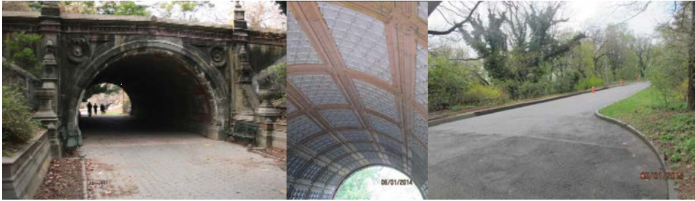
Hill Drive Bridge (Cleft Ridge Span) Bridge. May 2014: Tiles on Underside of Span 1. Top of Bridge.
