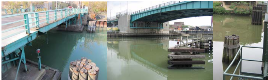
2014: Union Street Bridge Dolphins. Greenpoint Avenue Dolphin & Fender System. (Greenpoint Credit: Peter Basich) Hunters Point Avenue Dolphins. (Credit: Michele N. Vulcan)
