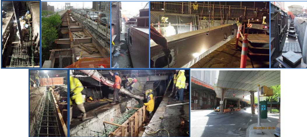
April 2014: Main Street Structure – Cap Beam Concrete Placement. May 2014: North Cantilever Demolition. York Street Structure – East Abutment Cap Beam. May 2014: Main Street Structure – Abutment Concrete Placement. Protective Shield and Work Platform at Manhattan Ramps and Approaches.
