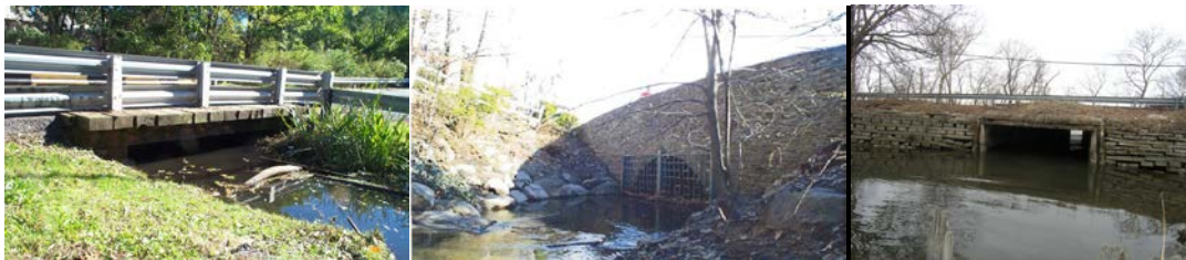
Idlesee Place Culvert. Sweet Brook Road Culvert. Richmond Terrace over Snug Harbor Culvert.
