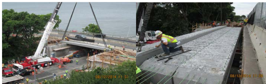
August 2014: Unloading and Placing the Pre-cast Concrete Box Beam on the North Side Abutments. Lowering the Third Pre-cast Concrete Box Beam.
