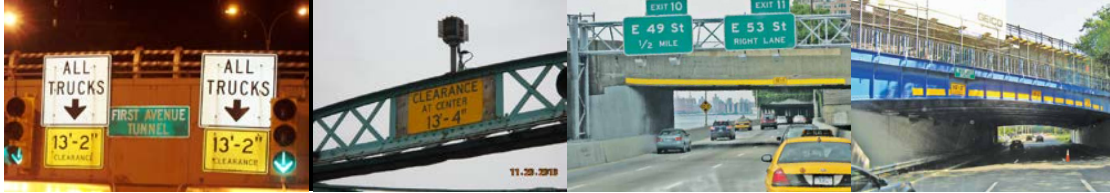
United Nations – 1 st Avenue Tunnel Vertical Clearance Posting. Grand Street Vertical Clearance Posting. (Credit: NYSDOT) Retro-reflective Material Improves Visibility of These Low Vertical Clearance Bridges: East 60 th Street Bridge Over FDR Drive and Westchester Avenue Bridge over Hutchinson River Parkway.
