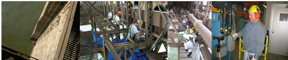
Repairing the Brooklyn Bridge Standpipe System, 130 Feet Below the Roadway. Maintenance Crew Conducting the Annual Cleaning and Lubrication of the Solid Rod Suspenders Spherical Bearings on the Brooklyn Bridge. 2 nd Photo - Oilers Steven Marxhausen, Rene Francis, Richard Morreale, Thomas McAuliffe, and Andrew Sorrentino. (Credit: Anatoly Orlov) Oiler T. McAuliffe at the 9 th Street Bridge
