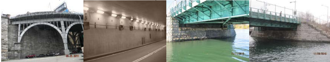
Riverside Drive Viaduct Abutment End. Battery Place Underpass Abutments. City Island Bridge Beginning and Ending Abutment. (Credit: NYSDOT)
