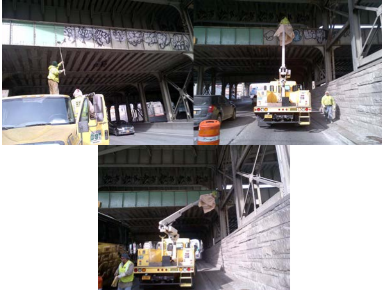
February 2014: Bridge Painters Michael Scotti (on Truck), Russell Newme (Operating Truck), and Willie Tyler, Supervisor Bridge Painter Cesar Pazmino, and Bridge Painter Frank Duic (in Lift Truck) Removing Graffiti on the LIRR Bridge Over the Van Wyck Expressway. (Credit: Earlene Powell)
