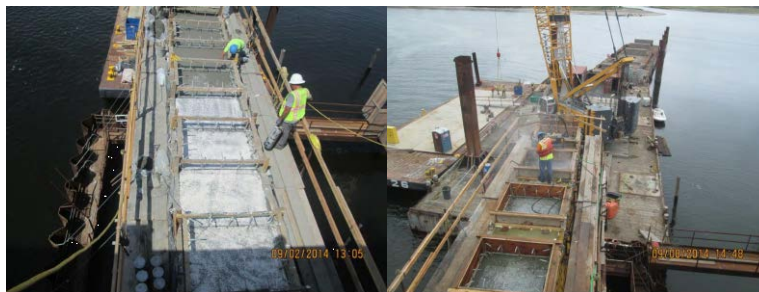
September 2014: Finishing Concrete on Pier Cap at Pier #2. Setting Forms for Concrete Pedestals at Pier #2 Cap Beam. Work Barge and Crane in Background.
