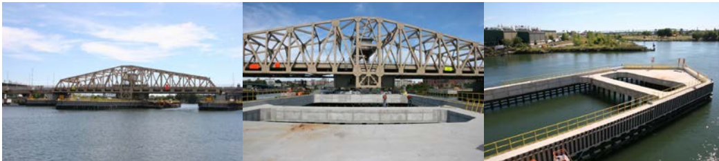
September 2012: Bridge Fender North Elevation Looking South. Bridge South Elevation Looking North. Pier 6 South Fender Looking South.
