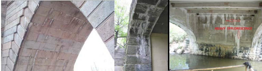
Moderate Efflorescence on the Brooklyn Bridge Brooklyn Tower North Gothic Arch in 2004. (Credit: NYSDOT) Efflorescence on the Underside of the Masonry Stones on the End Abutment of the Margaret Corbin Drive Bridge over Pedestrian Path Near Café. Heavy Efflorescence on End Abutment Stem Wall of Bridge Over Dam at Clove Lake.
