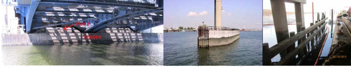
Metropolitan Avenue Bridge Fender. Rikers Island Dolphin & Fender System. (Credit: NYSDOT) Installing the Fresh Creek Bridge Fender System in 2013.
