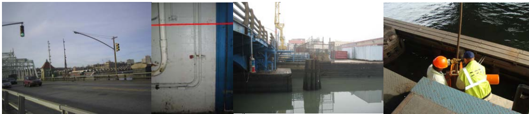
Inspection in Late 2012: East End of the West 207 th Street Bridge - Missing Traffic Signal was Knocked Down by the Hurricane Winds. Borden Avenue Bridge Operator's House Basement Level – Depicted Flood Line was Approximately 5 Feet Above the Floor. Third Street Bridge – Northwest Channel Light Missing. Ninth Street Bridge – Manually Pulling the Cable Reel Because the Motor Failed.
