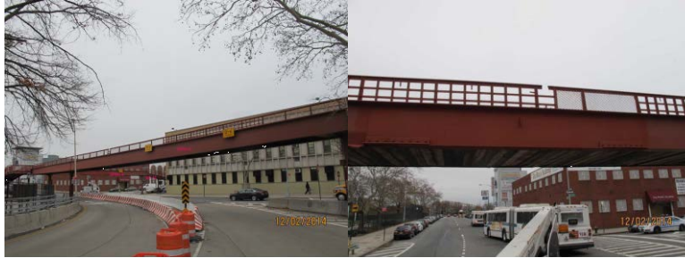
East 128 th Street Pedestrian Bridge Strike and Emergency Repairs. Left Elevation of Bridge. Timber Shielding Installed on Underside of Span #9 to Prevent Loose Concrete From Falling on the Road. Right Girder at Span #9 After Repair.
