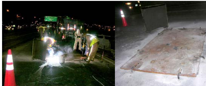
Ironworkers Setting a Steel Plate on Top of a Through-Hole on the Brooklyn-Queens Expressway. (Credit: Clara Medina)
