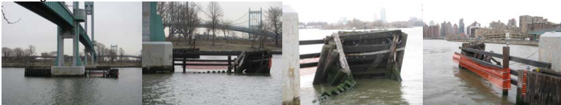
Wards Island Pedestrian Bridge – Collapsed Fender.
