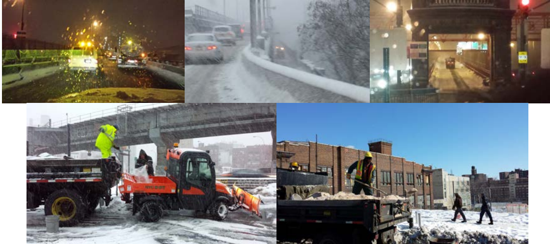
February 13, 2014: Brooklyn, Manhattan, and Williamsburg Bridges. Loading Solid Chemical for Spot Applications on the Williamsburg Bridge Walkway/Bicycle Path. February 14: Sanding at East 153 rd Street and Grand Concourse. (Credit: Paul Schwartz)
