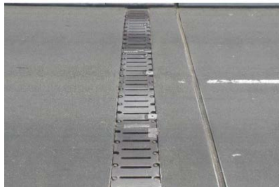
Manhattan Bridge Trench Drain.
