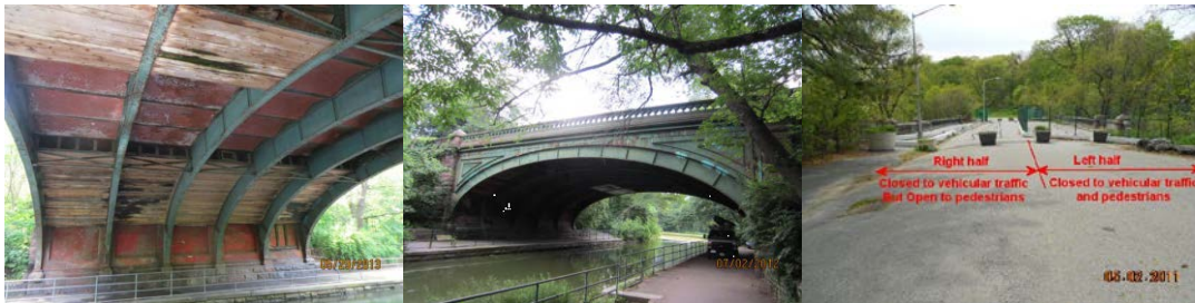
Hill Drive Bridge Span 2 Pier 1 End Face in 2013. View of Bridge in 2012. End Approach in May 2011: The Bridge is Closed to Vehicular Traffic. The Left Half of the Bridge is Closed to Pedestrians. (Credit: NYSDOT)
