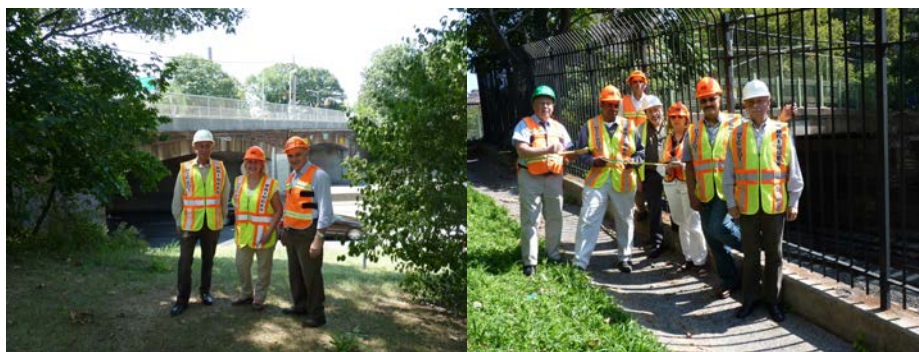
August 2014: In-House Design Engineers Inspecting the Union Turnpike Bridge over Cross Island Parkway – Assistant Civil Engineer Leonid Sagalovskiy, City Planner Ristina SekullaNessel, and Civil Engineer Edvard Jeamgocian. (Credit: Paul Schwartz) In-House Design Engineers Inspecting the East 169 th Street Bridge over Metro North Railroad – Civil Engineer Gregory Novofastovsky, Director of In-House Design Ferdinand John, Civil Engineers Kamran Sikandar and Lev Gold, Assistant Civil Engineer Elena Marresova, Civil Engineer Kirolos Dimian, and Assistant Civil Engineer Leonid Sagalovskiy.
