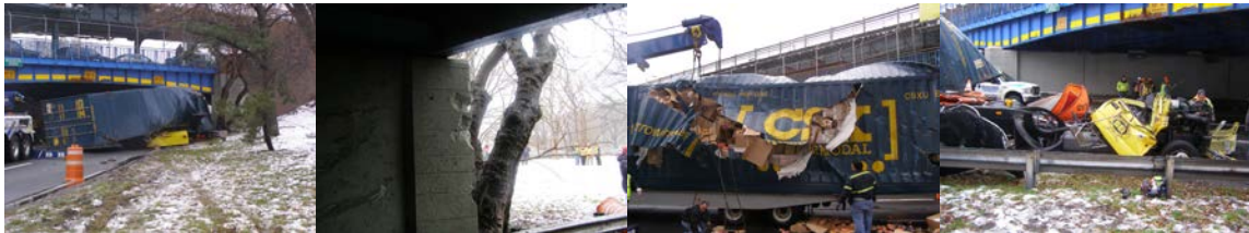
Damaged Bridge, Cargo Container, and Contractor Truck After An Over-Height Trailer Struck the Bridge in January 2012.
