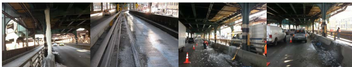
Huge Icicle (Caused by a Broken Water Pipe) Between the South Outer Roadway and the Inner Roadway at the Queens Approach of the Ed Koch – Queensboro Bridge. Icing on the South Outer Roadway. Division Engineers Closed Parts of the Roadway Until NYCTA Crews Completed the Removal of the Icicle and All of the Ice From the Roadway Surface and Barrier. Salt was Placed on the Remaining Ice on the Roadway. (Credit: Artemio Angeles)
