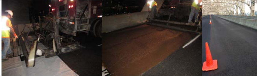
Resurfacing the Deck of the Queens-Bound Upper Roadway of the Ed Koch - Queensboro Bridge in June 2014. (Credit: Sunil Desai)
