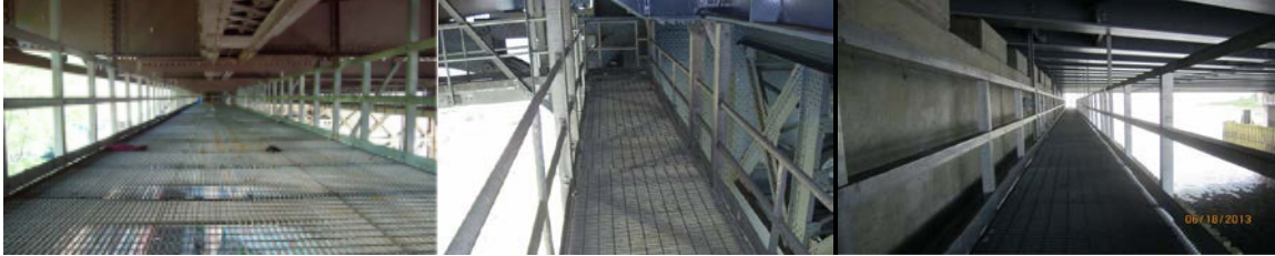
Ed Koch Queensboro Bridge Lower Level Flooring System Catwalk under Lower Level Queens Approach. Manhattan Bridge Brooklyn Tower Catwalk. (Credit: NYSDOT) Fresh Creek Catwalk Under Deck.
