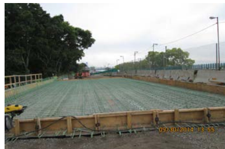
September 2014: Rebars in Place Prior to Placing Concrete Deck on Precast Concrete Beams on the North Side.
