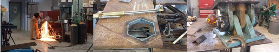
July 2014: Supervisor Bridge Repairer and Riveter Steve Havemann Fabricating a Wrench to Remove Nuts From a Seized Rocker Bearing.
