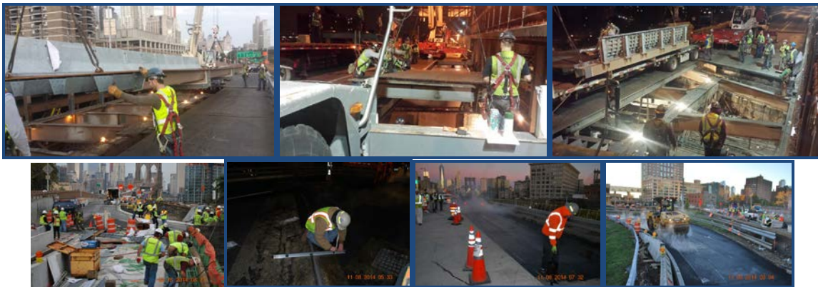
September 2014: Franklin Square Structure – New Orthotropic Deck. October 2014: Contractor Setting Rebar for Cast-in-Place Curb at Manhattan-Bound Tillary Street Access Road/Sands Street Access Road. November 2014: Manhattan-Bound Brooklyn Approach Paving.
