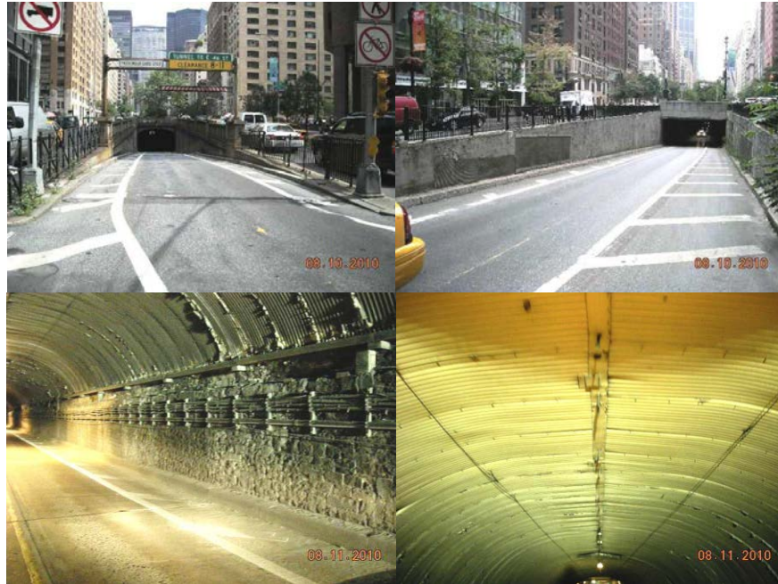
Two Views of Park Avenue Tunnel in 2010. Abutment Beginning. Underside of South Arch. (Credit: NYSDOT)
