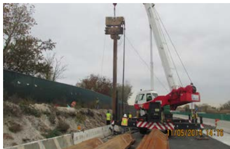
November 2014: Driving Steel Sheeting at East Approach for the Future Temporary Access Roadway.
