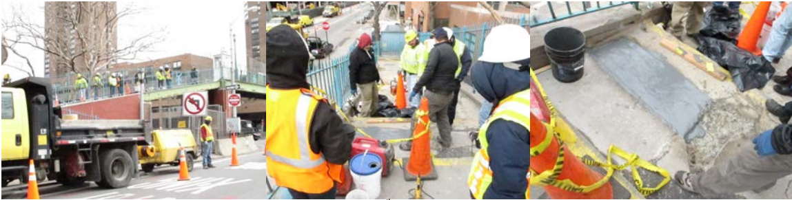
Division Staff Testing a New Patch Material on the East 25 th Street Pedestrian Bridge Over the FDR Drive in March 2014. (Credit: Bojidar Yanev)
