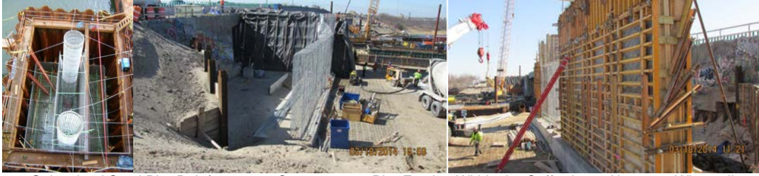
Galvanized Steel Pier Reinforcement Cages, set on Pier Footing Within the Cofferdam. Abutment Wingwall Reinforcement Steel, Prior to Setting Wall Forms on Previously Placed Wall Footing at Northeast Corner of the Abutment. 3/18/14 Wingwall Forms at North-West Abutment Wingwall. The existing bridge is at right.
