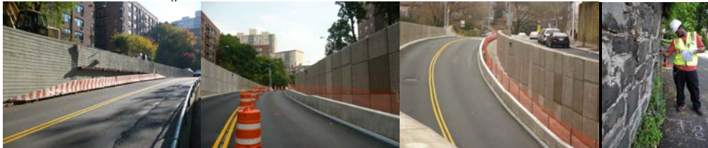
Kappock Street Retaining Wall in Riverdale, Before and After Repairs. The Existing 300-Foot Long Parallel Concrete Roadway Retaining Walls on Both Sides of Kappock Street Were Deteriorated and Leaning, and Were Replaced with New Modular Retaining Walls in the Summer of 2009. Inspecting a Bulge in a Retaining Wall Along Douglas Road in Staten Island in 2014.
