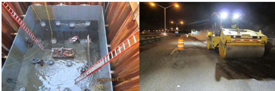
Workers Preparing to Dewater Cofferdam at Pier No. 1. . Steel Wheel Roller Compacting Hot Mix Asphalt During Nighttime Operation on Eastbound Belt Parkway West Side.
