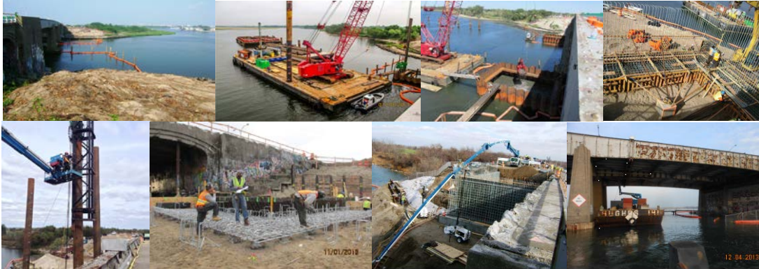
June 2013: North Side of Gerritsen Bridge - Turbidity Curtains Placed on Both Sides of Navigable Channel. July 2013: Work Barges Driving Steel Sheeting for Pier #1 Cofferdam. September 2013. October 2013: Rebars and Form Work for Footing and Walls at the Northwest Abutment. Stage 1 Piles. November 2013: Inspecting Rebar. December 2013: Tremie Concrete Pour at Pier #2. Inspecting Spans 7 & 8 of the Existing Bridge From a Barge. (Inspection Credit: NYSDOT)
