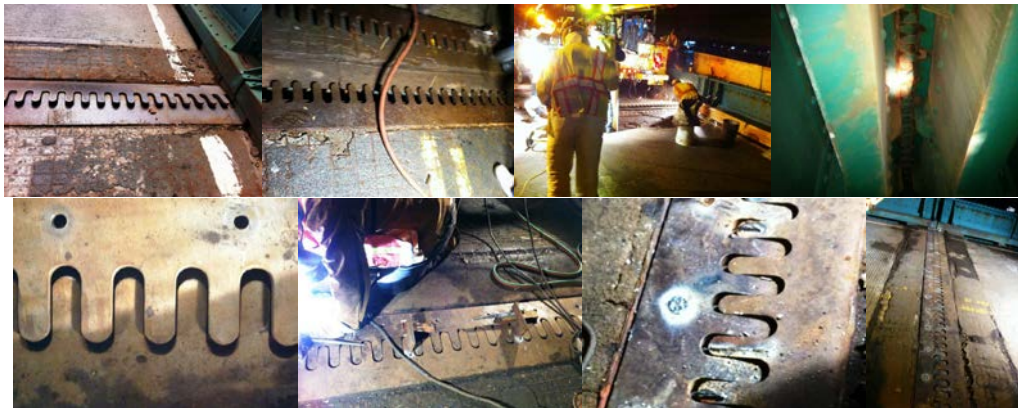
July 2013 PIA Safety Flag on the City Island Bridge. The repairs, conducted after a record-breaking heat wave, involved opening the joint plates and installing plug welds, which helped correct the plates' position and recreated the proper gap to allow the bridge to expand and contract safely. Finger Joint Before the Repair. Open Finger Joint. Division Crews Repairing the Joints. View Beneath the Finger Joint. The Joint Plates are Placed to Check for the Proper Gap. Leveling the Plate Before Welding. Close-Up of a Plug Weld. After 17 Plug Welds, the Finger Joints Sit Flush on the Roadway.
