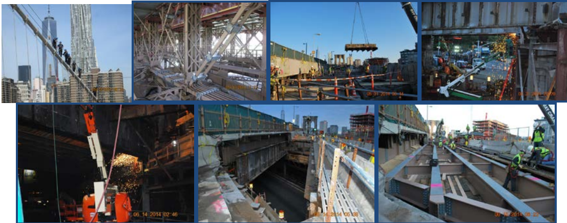
May 2014: Ascending the Cable. Installing Clamping Assemblies at the Franklin Square Structure. May 2014: Main Street Structure Westbound Overpass Replacement During Full Weekend Closure. June 2014: York Street Structure Stage II Westbound Overpass Replacement During the Full Weekend Closure.
