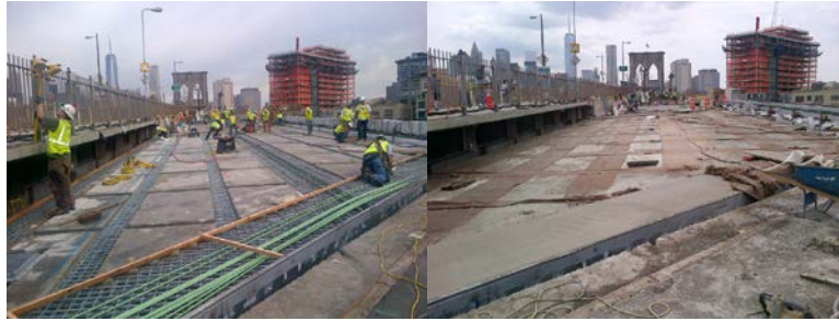
July 2014: Set up for Main Street Structure Concrete Pour. Concrete Pour Complete With Wet Burlap in Place for Cure.
