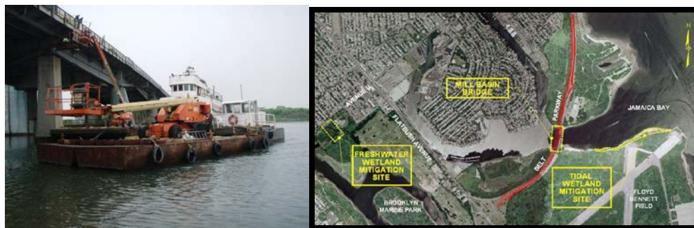
May 2013 – Inspecting the Bridge From a Barge. Freshwater and Tidal Wetland Mitigation Sites.
