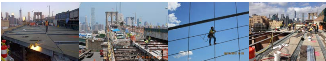
April 2014: Installation of Temporary Deck Units at the York Street Structure Over Brooklyn-Queens Expressway. July 2013: Removal of the Existing Concrete Slab on the Eastbound Main Street Structure. August 2013: Ironworker Replacing Cable Clamp Assemblies on the Suspended Span. October 2013: Grid Deck Panel Installation at the Eastbound Park Row Structure.
