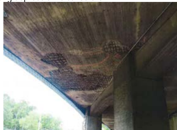
Hollow Sounding And Delaminated Concrete Areas With Exposed Rebars on the Sunrise Highway Bridge Westbound over Laurelton Parkway in 2014.
