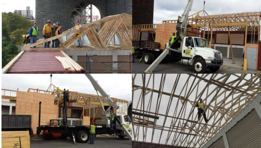
October 2014: Installing Trusses for a Roof to Enclose the Trailers to Create a Shop Area at Vernon Boulevard for Maintenance of Anti Icing Equipment - Carpenters Stephen Buckley, Joseph Moschella, Construction Project Manager Hany Soliman, and Carpenters Edward Alfano and Gregory Nolan. This Replaced the Pulaski Yard Which was Damaged by Hurricane Sandy. (Credit: Thomas Whitehouse) Executive Director of Bridge Preventive Maintenance and Repair Thomas Whitehouse Inspecting the Connections.
