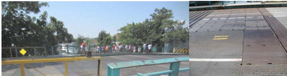
Union Street Bridge - Schoolchildren Crossing in 2012. (Credit: NYSDOT) 2014: Eleven Steel Plates Covering the Steel Grid Deck.
