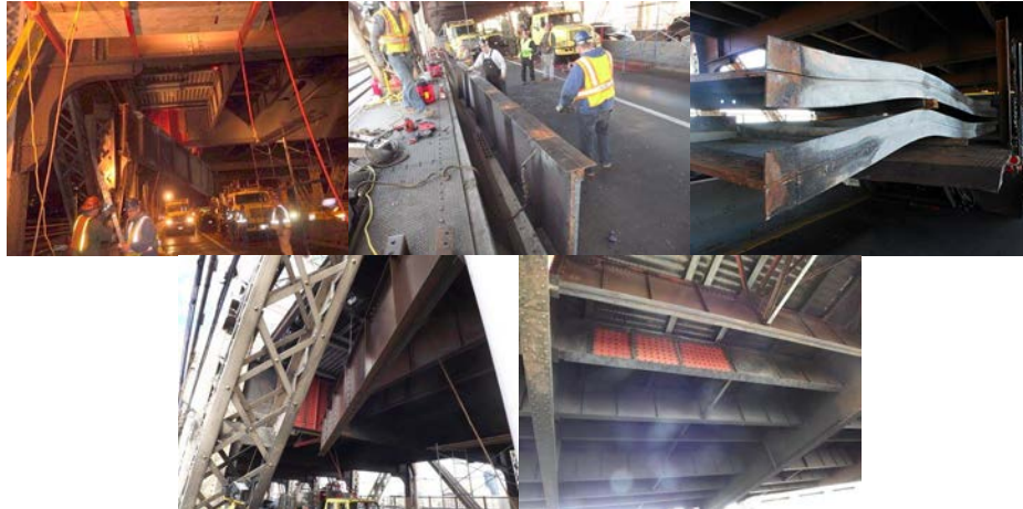
August 2013 Red Flags on the Ed Koch Queensboro Bridge. October 2013: Removing the Warped Beams. The New Beams.
