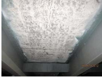
Union Street Bridge over Brooklyn-Queens Expressway in 2012 – Extensive Map Cracking With Efflorescence on the Underside of the Deck. (Credit: NYSDOT)
