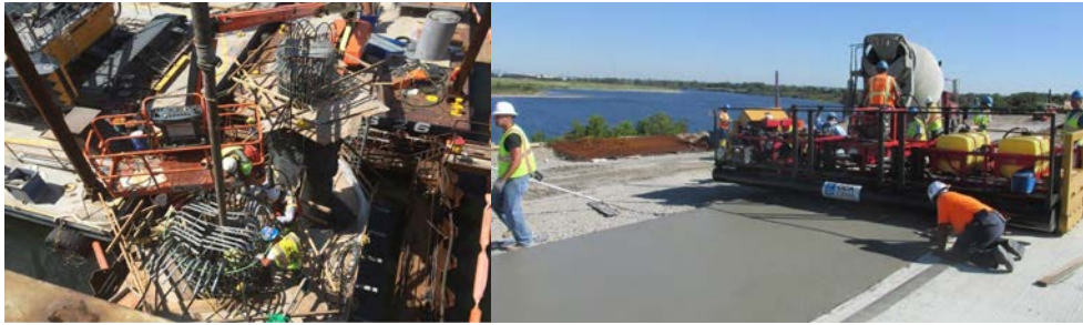
August 2014: Pumping Concrete Into Column Cage at Pier #2. Finishing Pavement at West Approach.
