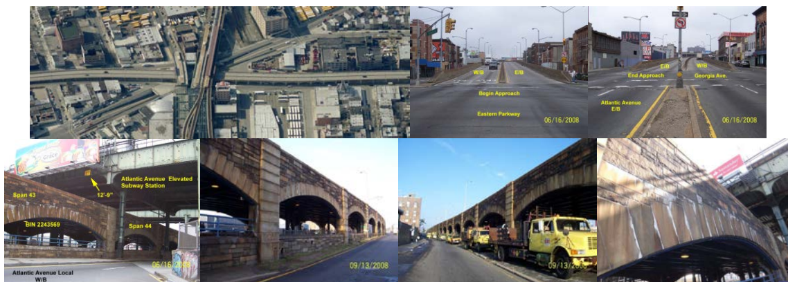
Aerial View in 2009. Beginning and End Approaches. Elevation Right – Spans 43 – 44. Elevation Left Spans 38 -43 and Elevation Right Spans 20 – 34. (Credit: NYSDOT) Span 43 South Arch Shows Typical Efflorescence at Mortar Joints of Ring Stones.
