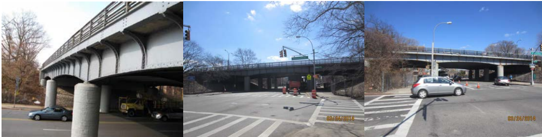
Nostrand Avenue Bridge Right Girder in November 2012. Left and Right Elevations in 2014. (2014 Credit: NYSDOT)
