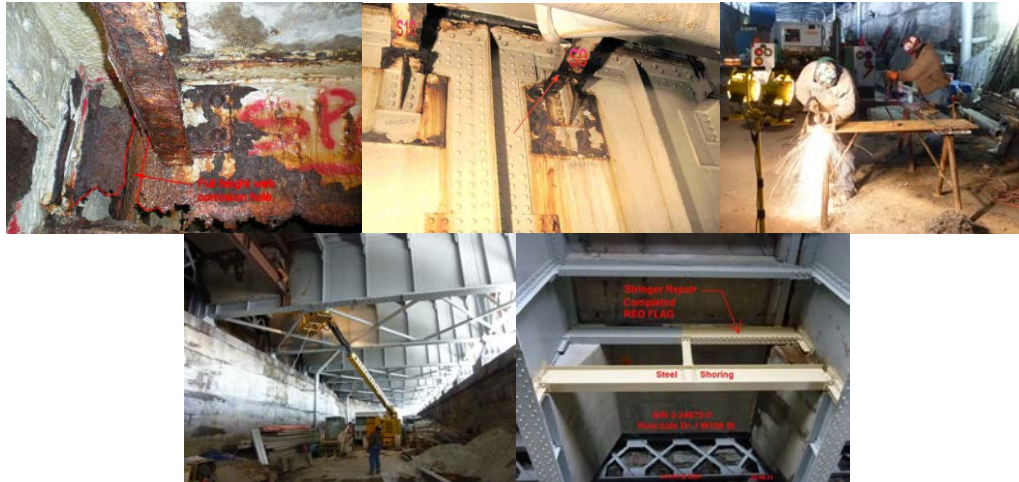
September 2008: Advanced Corrosion of Steel Stringer and Girder. February 2011: Red Flag Stringer Repair at Riverside Drive Viaduct over West 158 th Street.
