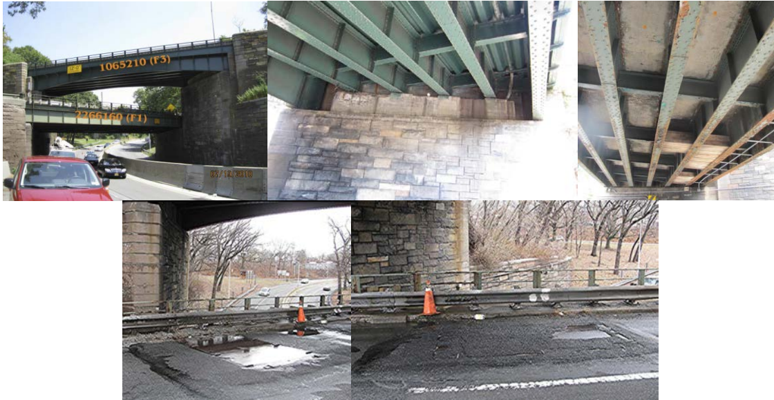
Bridge (Lower Structure) in 2010. (Credit: NYSDOT) Bridge Detail. August 2013: Span 1 Underside of Deck from End Abutment, Looking Northwest - Areas of Spalled Concrete Deck Are Protected With Timber Planks. March 2014: Steel Plates on Wearing Surface.
