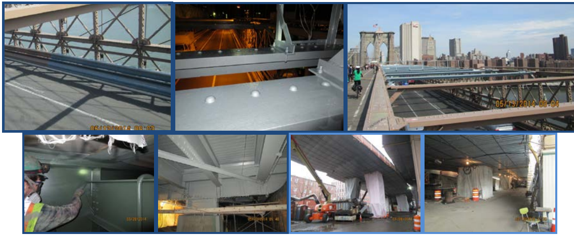
Spring 2014: Painting at Main Bridge – Safety Barrier and Top Struts. Painting at Manhattan Ramps. April 2014: Containment at Manhattan Ramps and Approaches.
