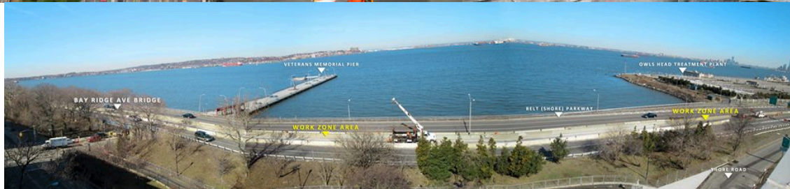
June 2014: Stage II Configuration. Bridge Deck Removed on Westbound Roadway. Panoramic View - Veteran's Pier at Right Above the Entrance to the NYCDEP Wastewater Treatment Plant. NYCDPR Bicycle/Pedestrian Promenade at Upper Right.
