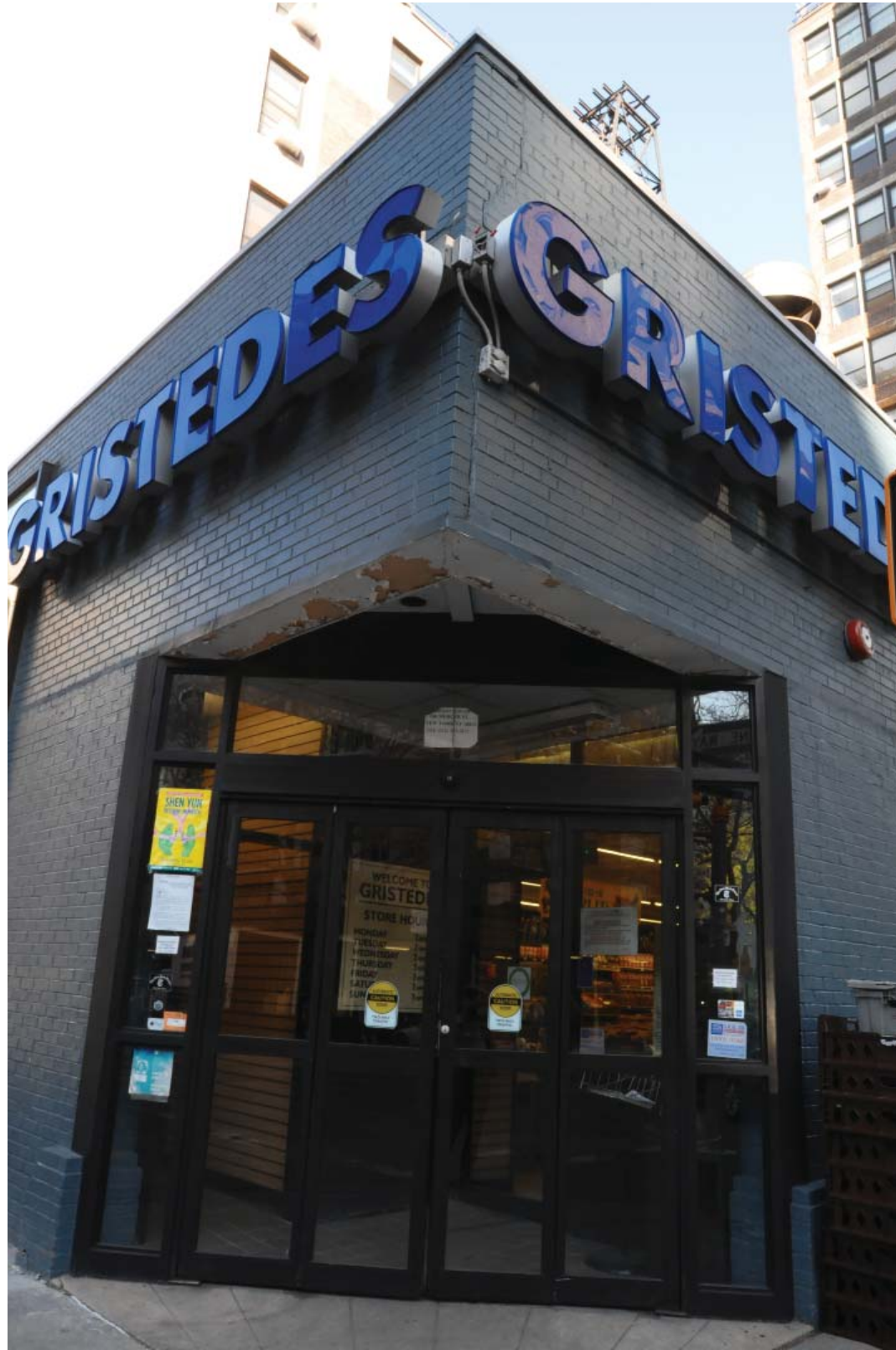
Detail Photo at Altered Corner Sliding Door
