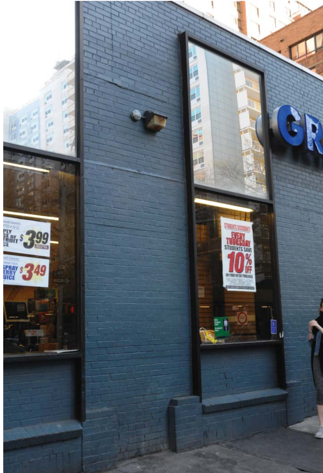
Detail Photo at Typical Altered Window
