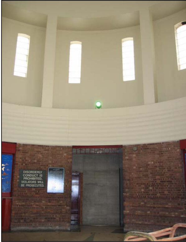
Tompkinsville (Joseph H. Lyons) Pool Bath House Interior: Telephone Alcove Photo: Tara Harrison, 2008
