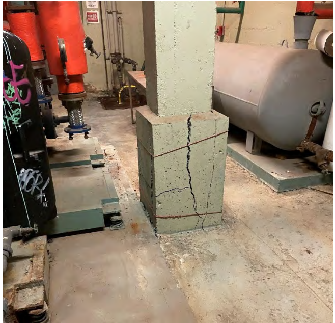
3 - Deteriorated cellar column base - three thus
