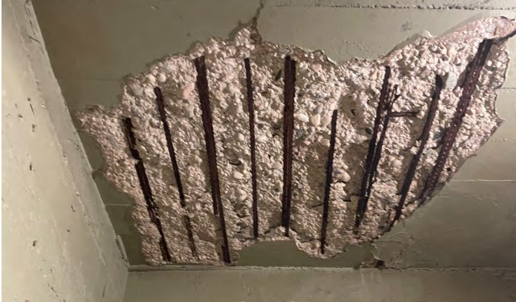
2 - Deteriorated sidewalk vault slab
