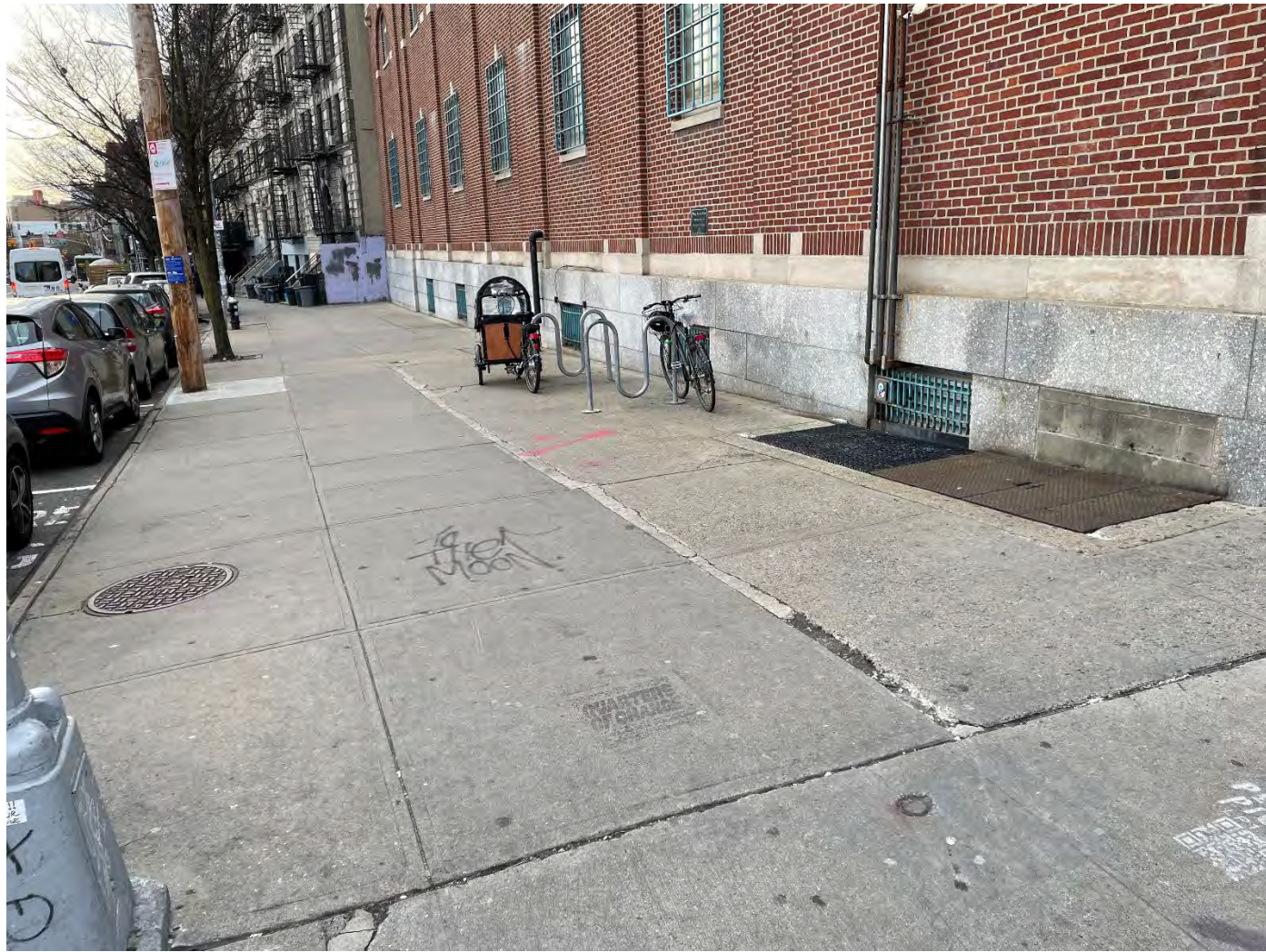
1 – View of sidewalk looking east. Sidewalk wearing surface to be replaced
