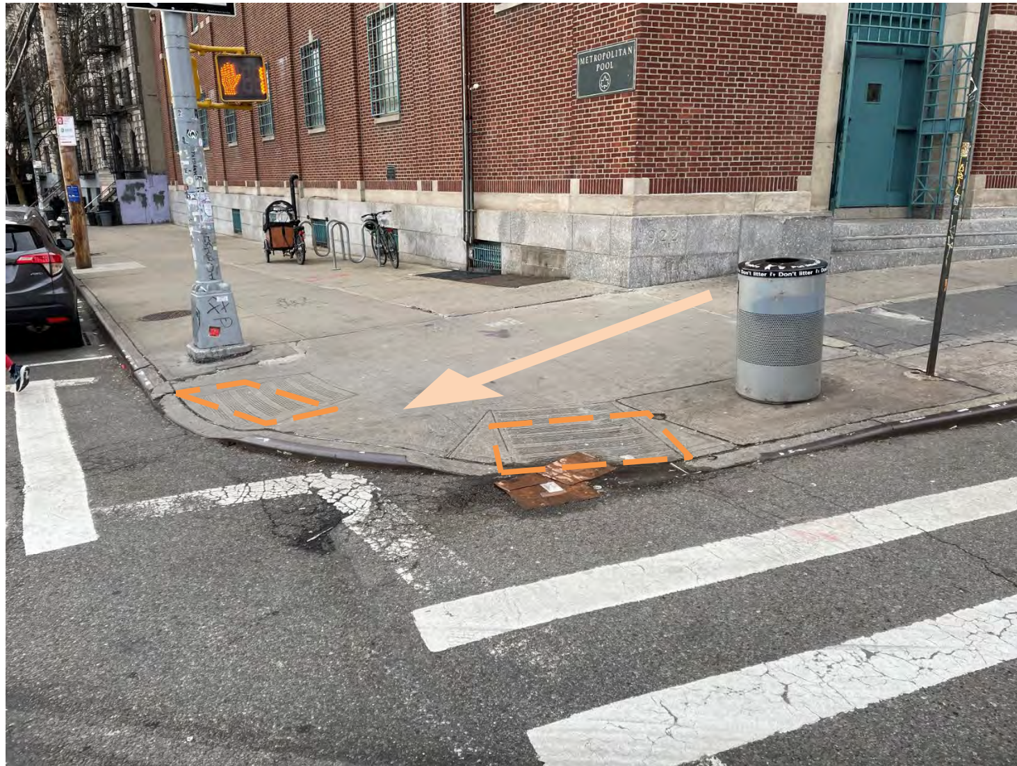
1 – View of sidewalk corner quadrant. Slope exceeds ADA standards at arrow
