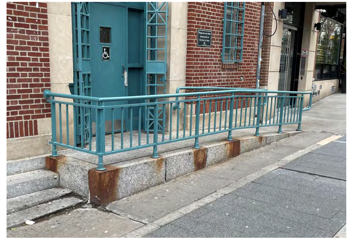
2 – View of ramp and handrail. Handrail to be raised to 34” Ramp staining to be addressed
