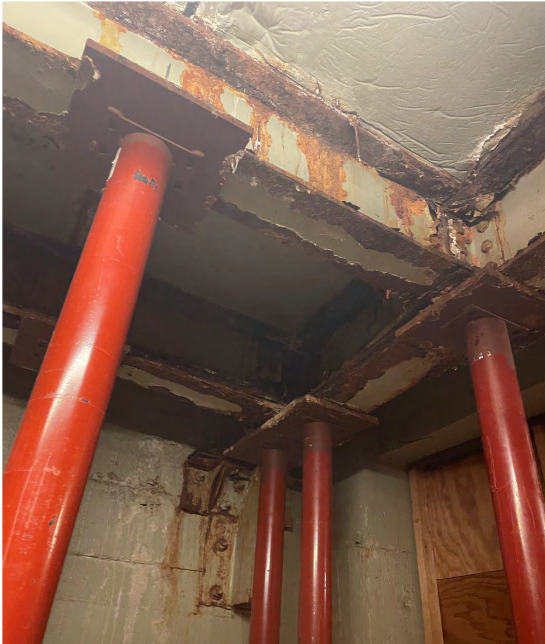
1- Deteriorated vault framing to be replaced
