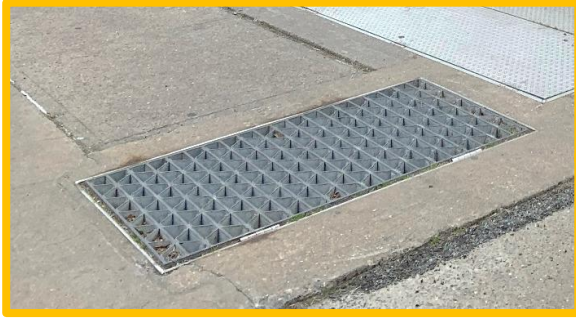
Existing Dry Well Vent at grade to be relocated and provided with new stack above grade to compliment original Ornamental Cast Iron Stack
