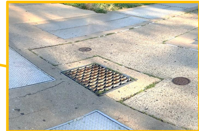
Existing Wet Well Vent at grade to be relocated above grade to compliment original Ornamental Cast Iron Stack
