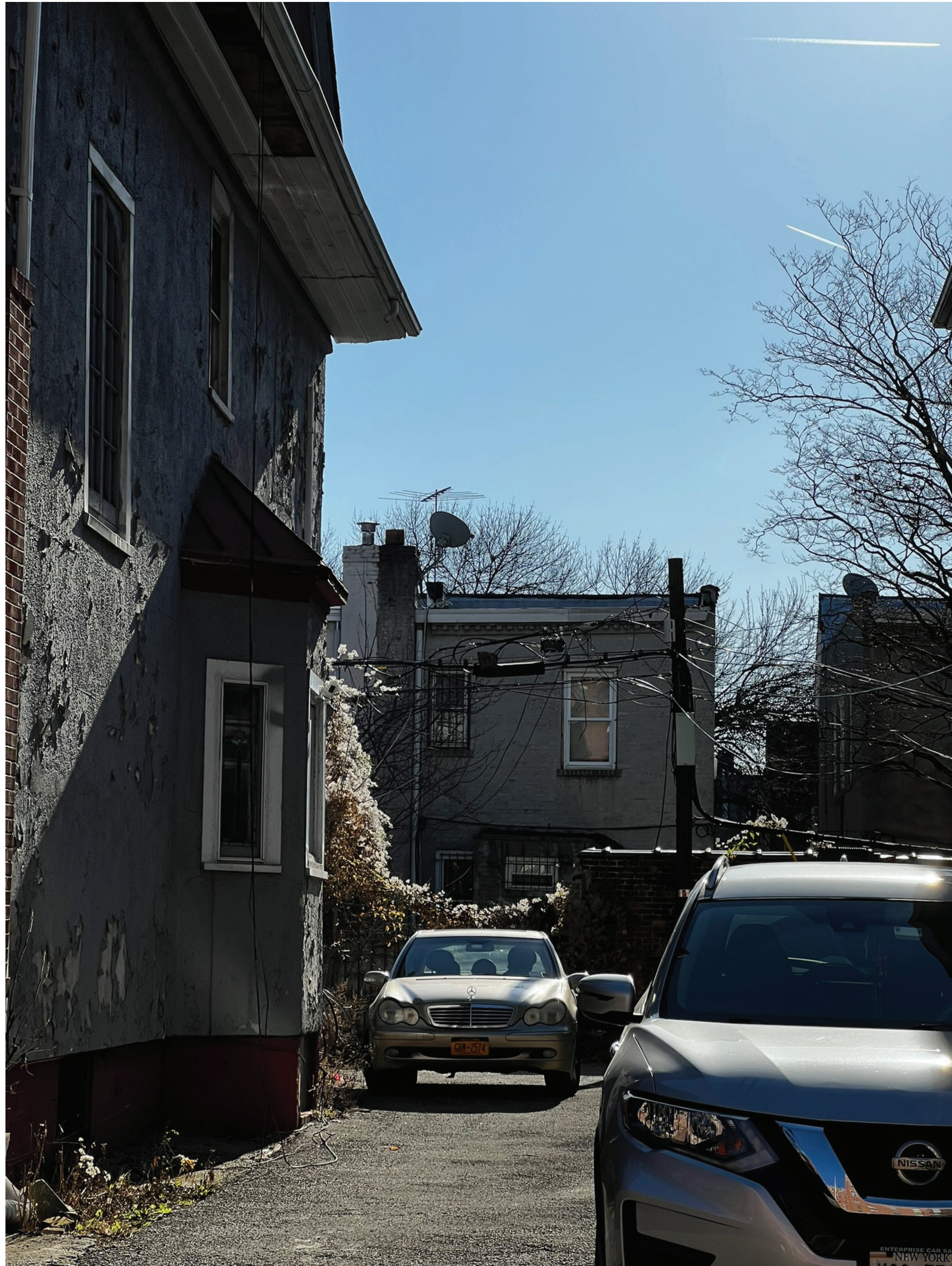
VIEW OF 25 MAPLE STREET REAR FACADE FROM 86 LINCOLN ROAD (EXISTING - ZOOMED IN)
