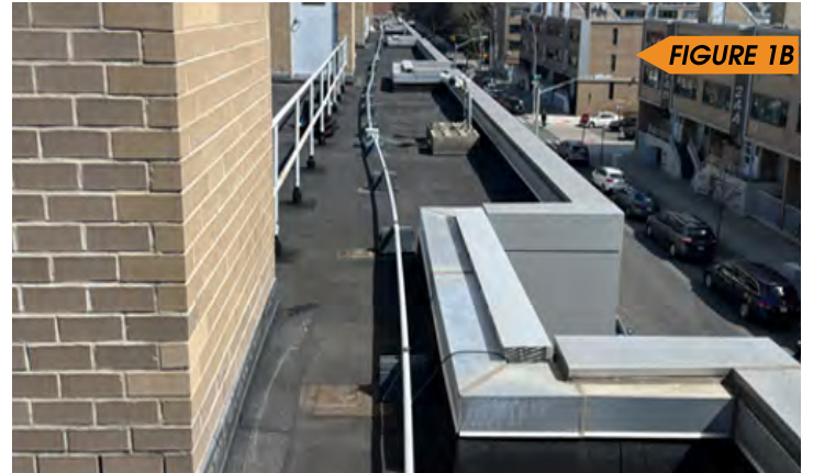
Figure 1B is a low parapet that is also subject to annual inspection.
