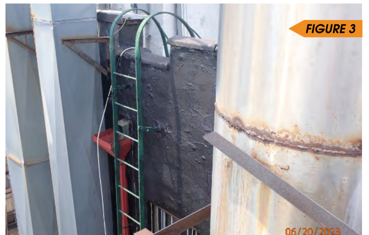
Figure 3 the ladder, ducts, and pipes are all examples of parapet appurtenances subject to annual inspection
