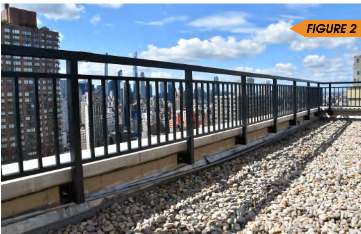
Figure 2 the guardrail is a parapet appurtenance and therefore is subject to annual inspection.
