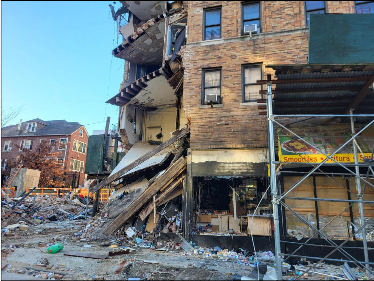
Image #3: Partial collapse at Exposure 1/2 Corner. (2023-12-11, FEU)
