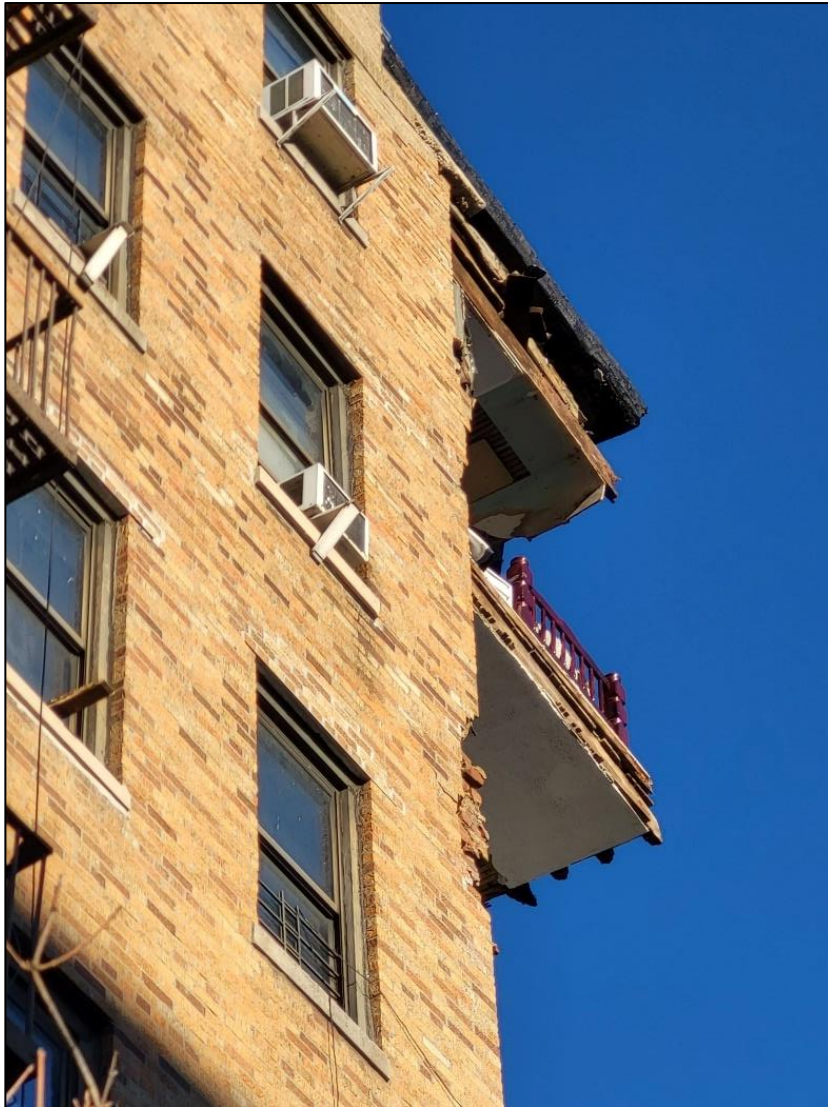
Image #6: Partial collapse at Exposure 1/2 Corner. Roof and 6 th floors at risk of further collapse (2023-12-11, FEU)
