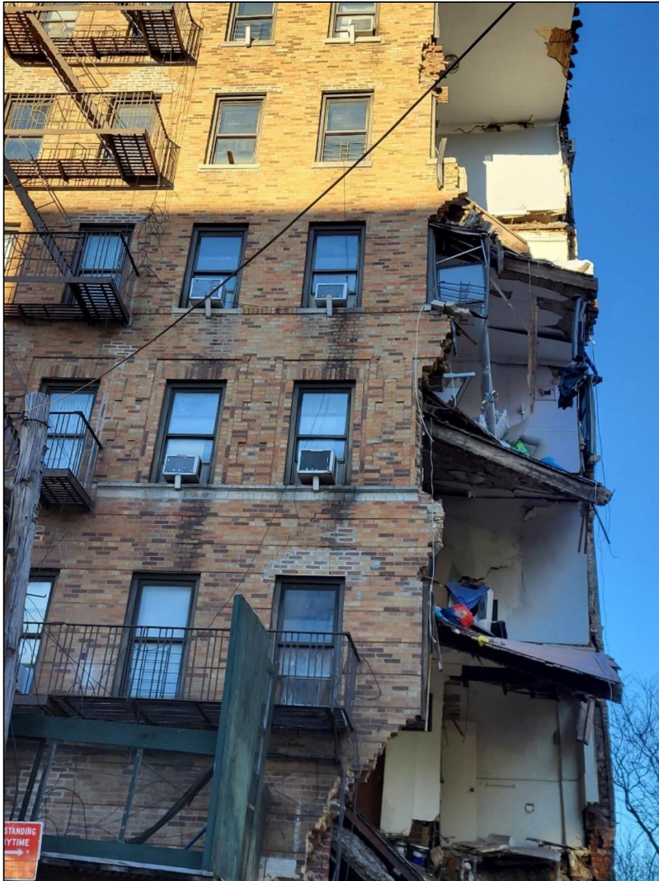
Image #4: Partial collapse at Exposure 1/2 Corner (2023-12-11, FEU)
