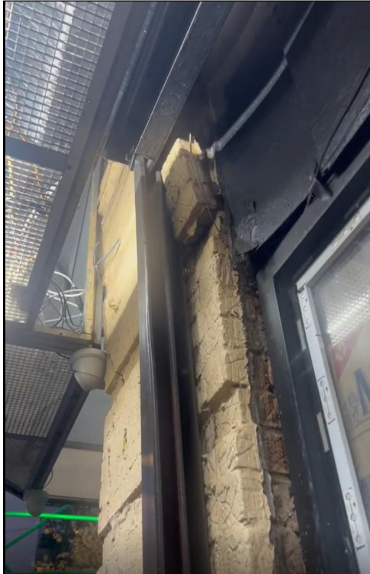
Image #11: Prior to collapse, photos extracted from video taken on October 29, 2023 – Bulging, displaced brick from the top of the cellar level load-bearing masonry pier along Phelan Ave. (2023-10-29, Deli owner )
