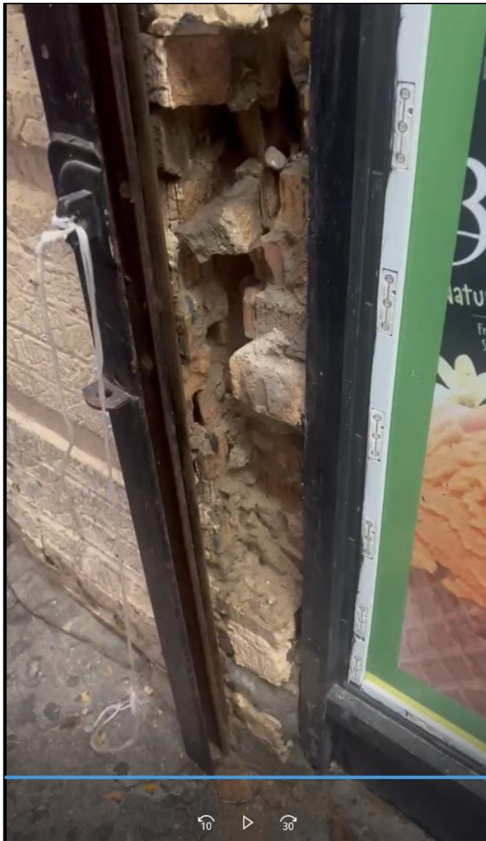
Image #12: Prior to collapse, photos extracted from video taken on October 29, 2023 – Bricks removed from cellar level load-bearing masonry pier along Phelan Ave. (2023-10-29, Deli owner)
