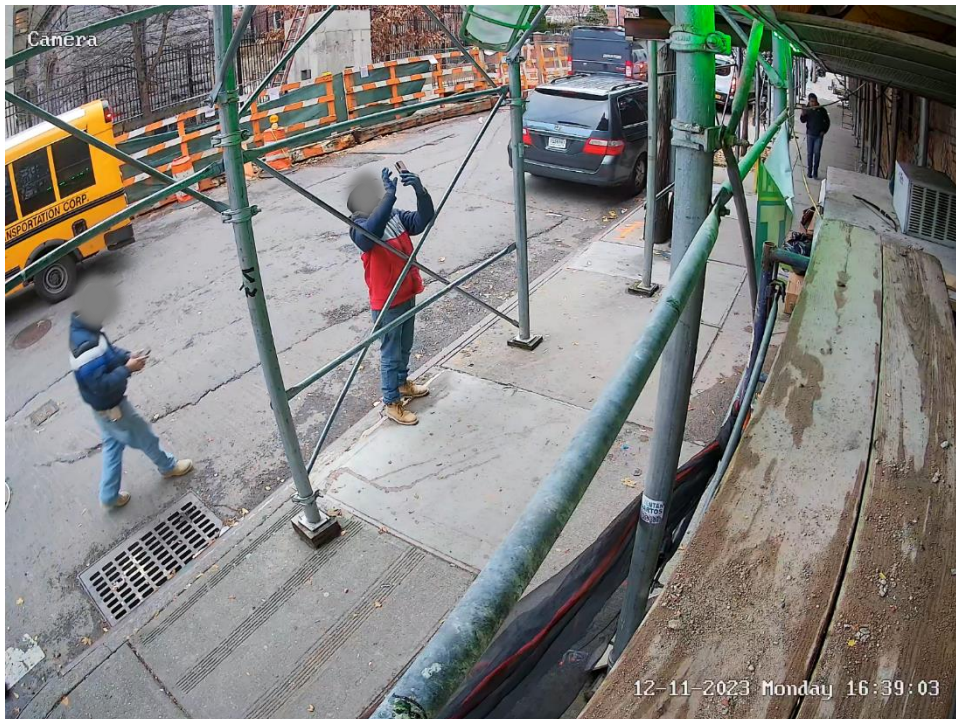
Image #42: D20 Camera Worker filming upper stories of building (2023-12-11, 172 W. Burnside Ave. Security Camera)
