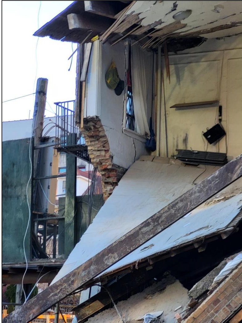
Image #5: Partially collapsed floor at Exposure 1/2 Corner. (2023-12-11, FEU)
