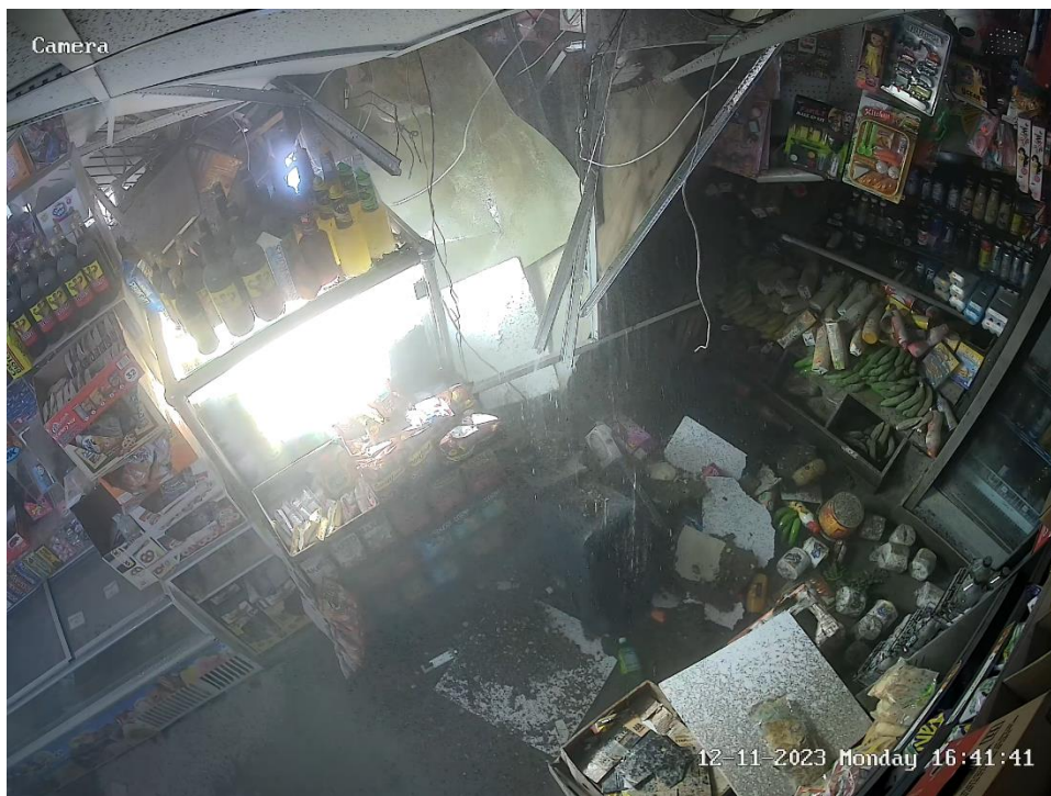
Image #20: D8 Camera Post-Collapse (2023-12-11, 172 W. Burnside Ave. Security Camera)
