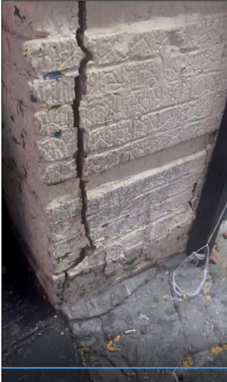
Image #10: Prior to collapse, photos extracted from video taken on October 29, 2023 – Vertical crack from grade at the cellar level load-bearing masonry pier along Phelan Ave. (2023-10-29, Deli owner)
