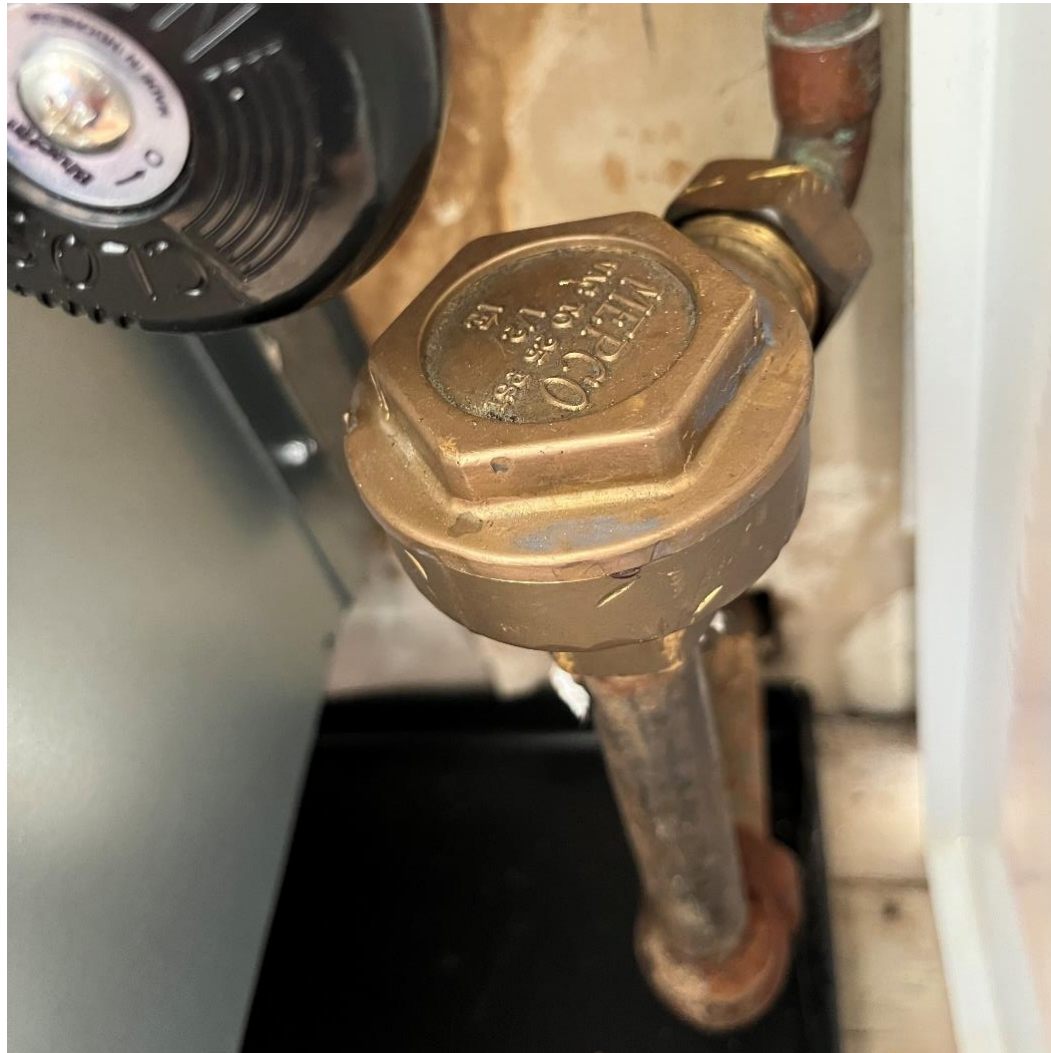
Thermostatic steam trap in a dwelling unit
