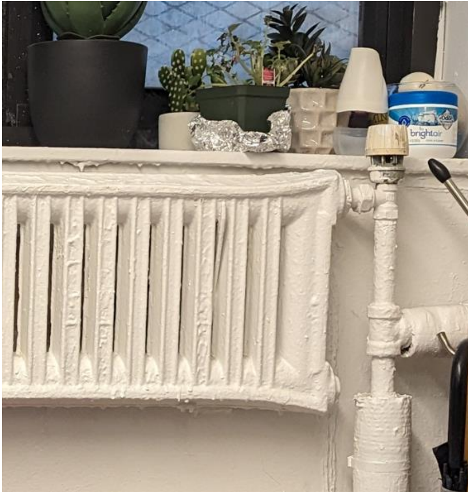
Two-pipe steam radiator with a TRV
