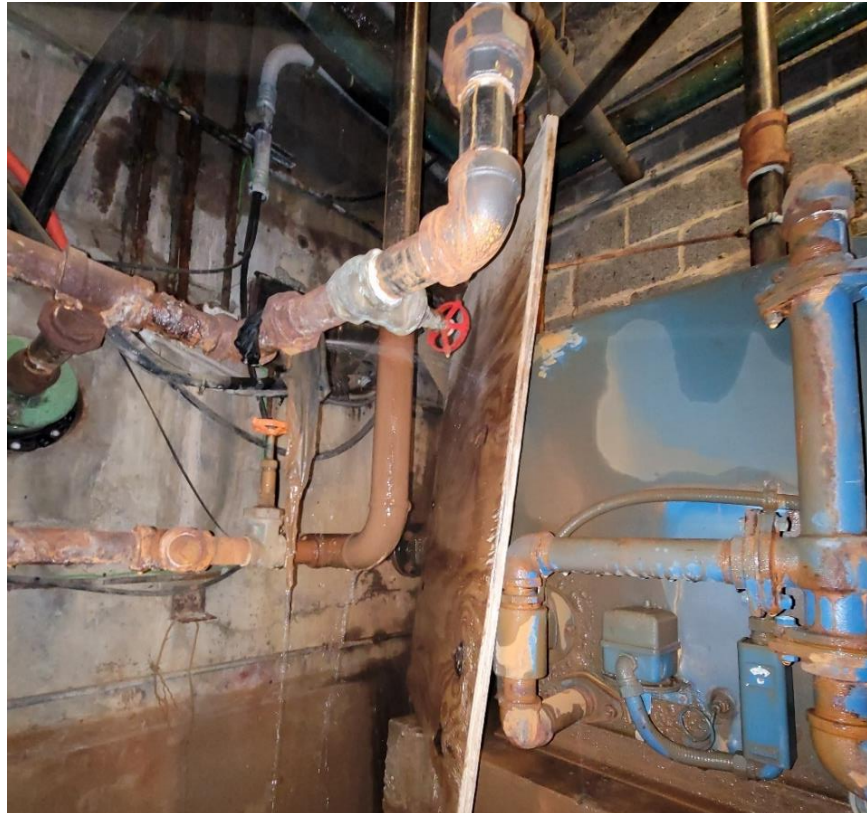
Water leak requiring repair
