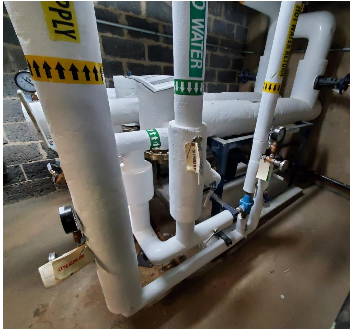
Insulated and labeled water pipes
