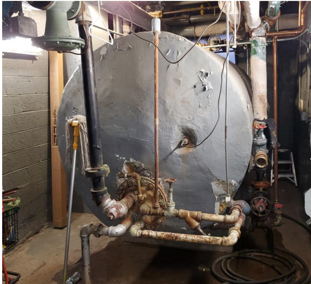
Insulated hot water tank
