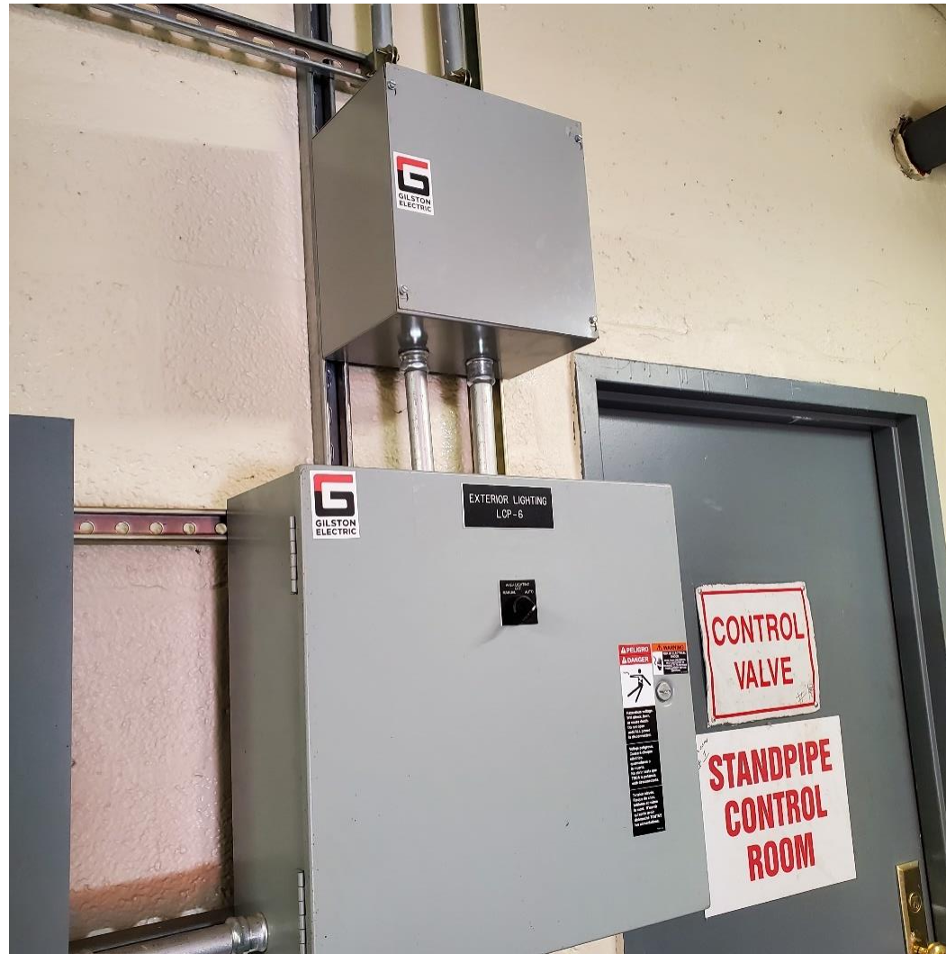
Exterior Lighting Controls
