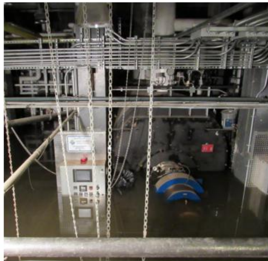
Mechanical room flooding following PTC Ida, Sept 2021
