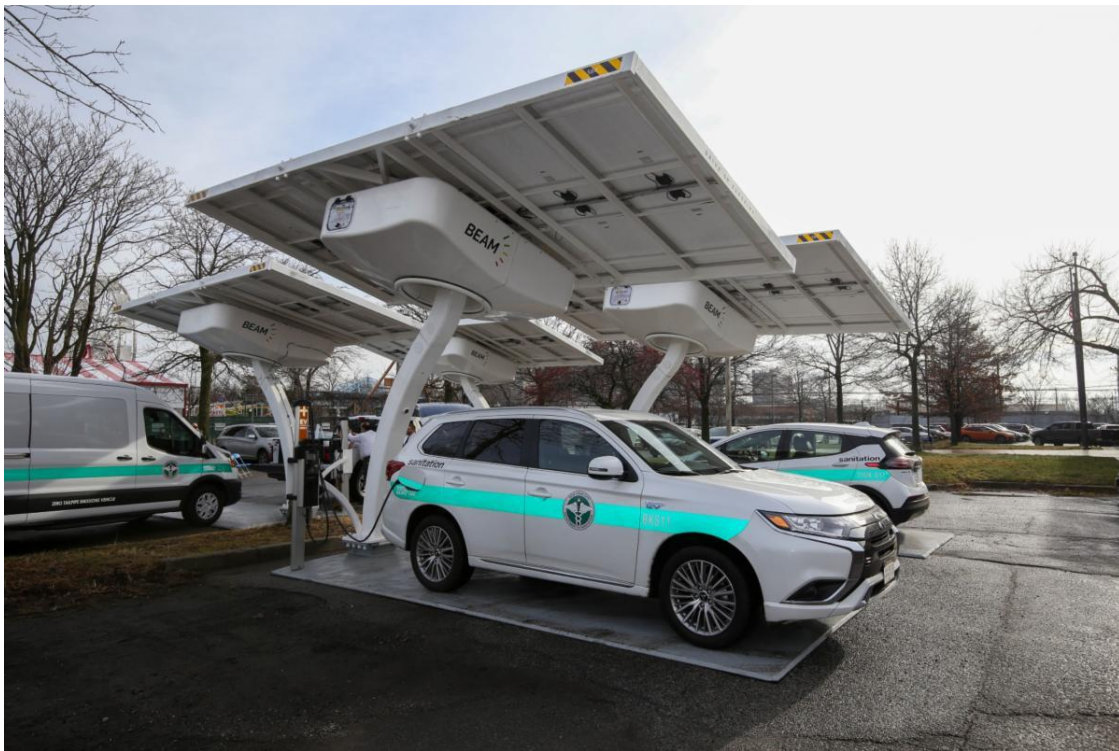
Solar carports charging NYC Department of Sanitation vehicles.
