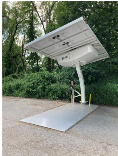
Recently installed free standing solar carport.
