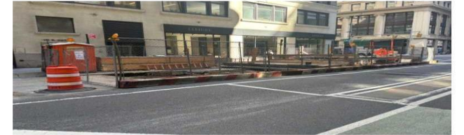
Hand care excavations on E. 29 th Street between Madison Avenue and 5 th Avenue.
