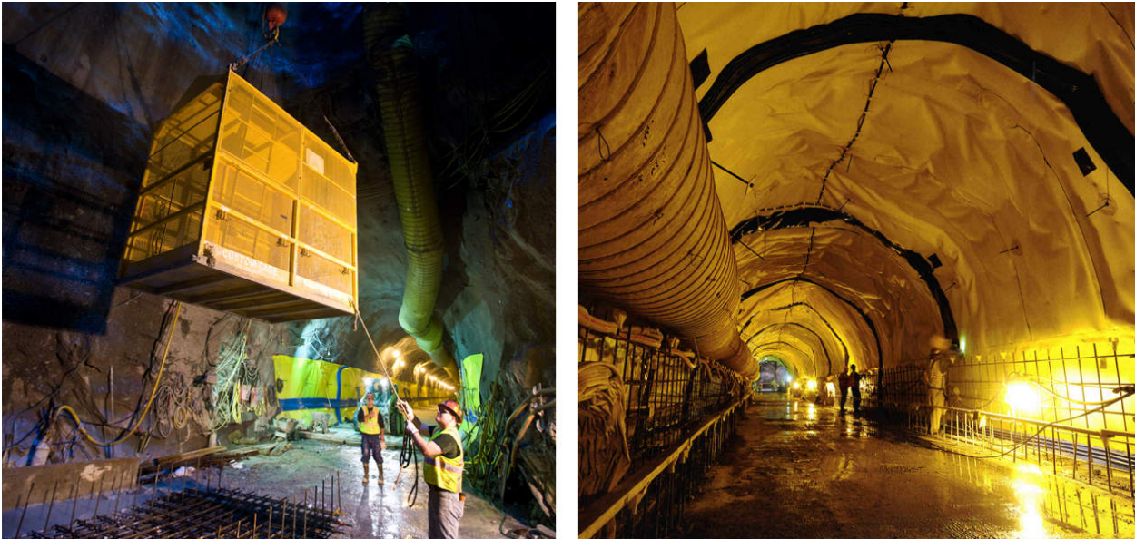
Figure 4: Con Edison Harlem River Utilidor Tunnel ( https://mrce.com/project/con-edison-harlem-river-utilidor-tunnel/ )
