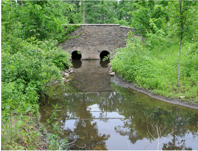
Figure 4. The Bluebelt system preserves natural drainage corridors to convey stormwater.
