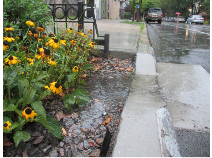
Figure 5. A green infrastructure "bioswale" intercepts stormwater runoff before it enters the combined sewer system.
