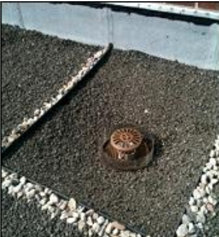
Broken Stone Weir at Roof Drain
