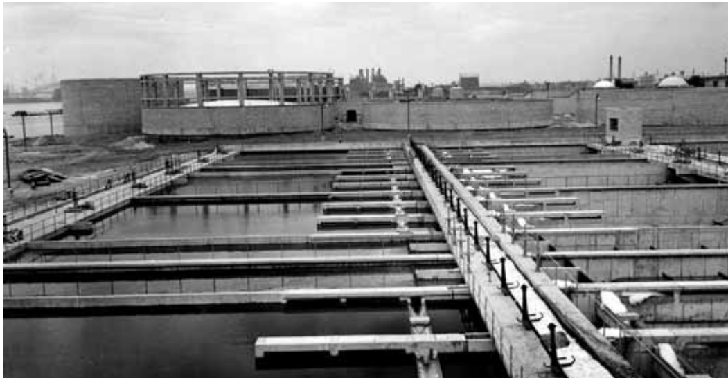
Final settling tanks at Bowery Bay Wastewater Treatment Plant
