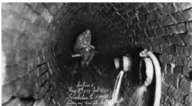
Sewer worker inside the New Street sewer; from Beaver to Wall Street, Manhattan (1928)
