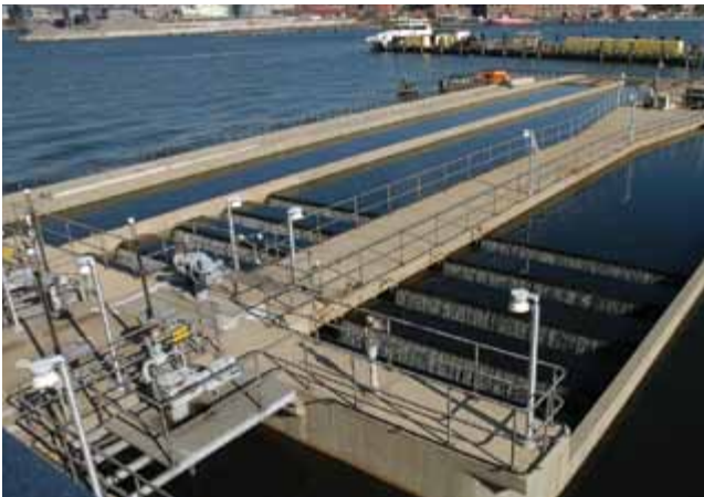
Red Hook Wastewater Treatment Plant chlorine contact tanks and the East River
