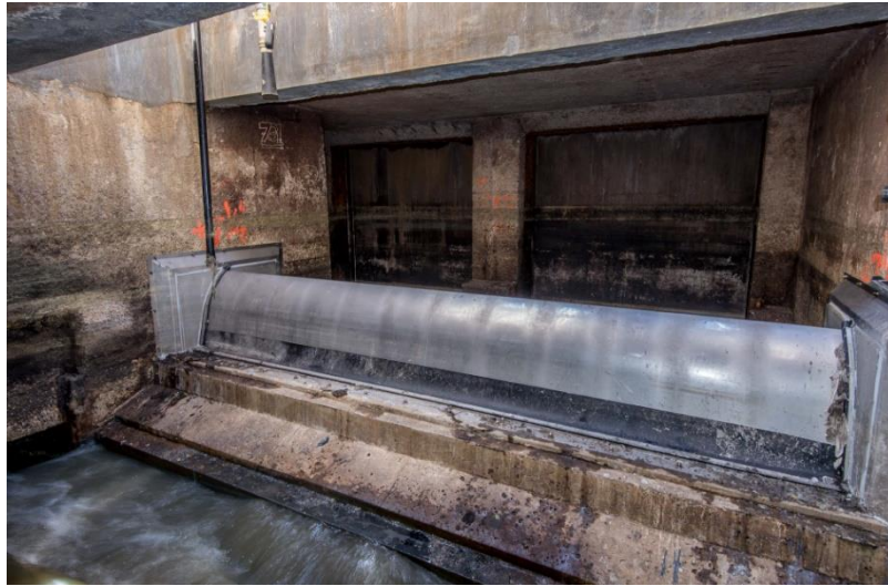
Figure 4-3: Bending Weir in Regulator JA-14
