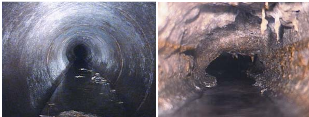
Images 7.2 and 7.3—The sewer on the left is clean while the sewer on the right has reduced capacity due to grease buildup.
