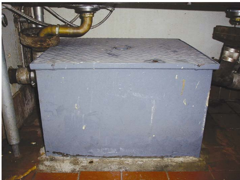
Image 3.2—Grease traps are small installed devices that remove grease from a sink’s wastewater.
