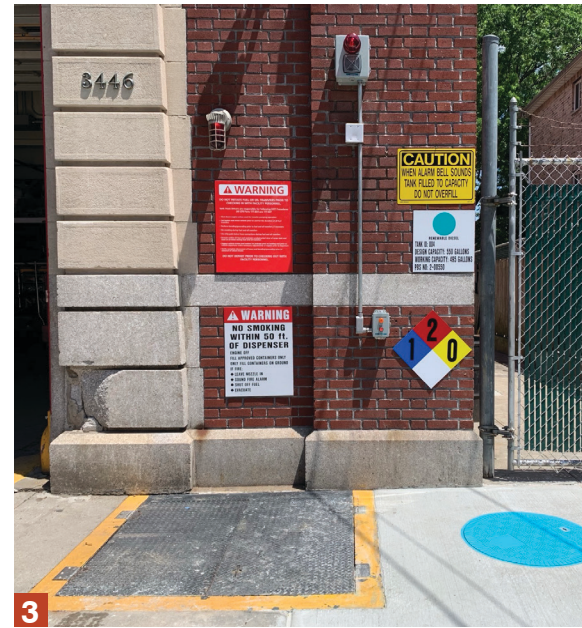
3. A standardized fuel tank access hatch and associated signage, switches, and alarms outside a Fire Department of New York Engine Company building
