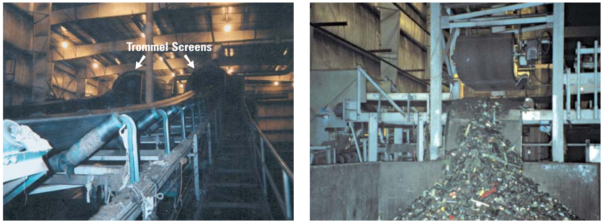
Photo 3-14: Conveyor to primary trommel screens (left) in the Edmonton facility and recovery of ferrous metals (right) Material discharged from the drum travels via conveyor to one of two three-inch trommel screens, which separates two fractions—"overs" and "unders." Before the three-inch unders move to the aeration bays, a magnet removes ferrous metals for recycling.
