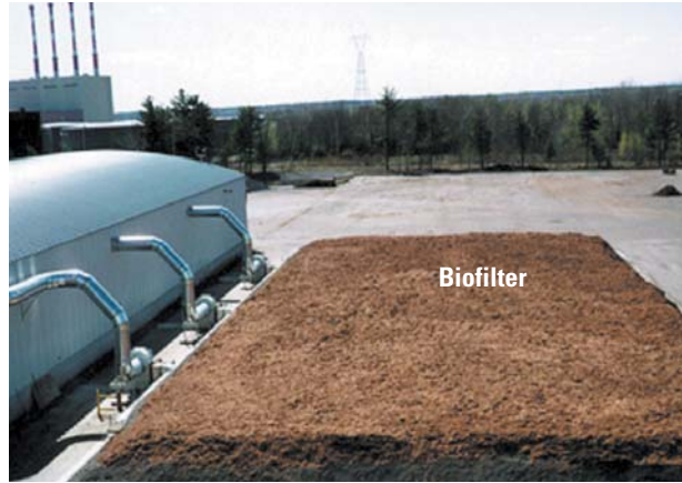
Photo 3-11: Conporec biofilter All process air from the receiving building, digester drum, and maturation building is filtered through a 200-by-80 foot biofilter.
