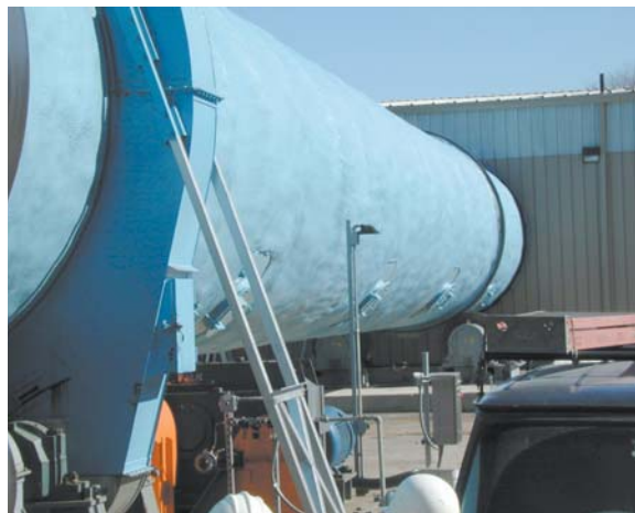
Photo 1-8: Digester Drum at the Marlborough Facility MSW loaded into the digester drum from the receiving building is discharged two to three days later in the air floor building.
