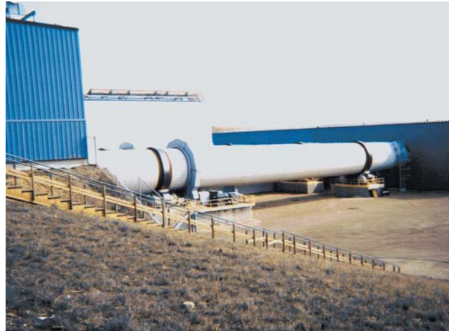
Photo 3-13: Digester drums at Edmonton facility
