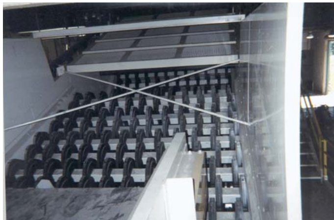
Photo 5-2: Debris Roll Screen at a Mixed-Waste MRF in Oakland, CA. Debris roll screens could be used in a pilot NYC facility to remove any small pieces of glass or plastic that were missed by the first screen.
