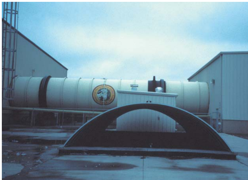
Photo 3-26: Digester drum at the Rapid City MSW-composting facility The facility uses two digester drums, each 14 feet in diameter and 79 feet long. The loading and discharge ends are enclosed inside two different buildings.
