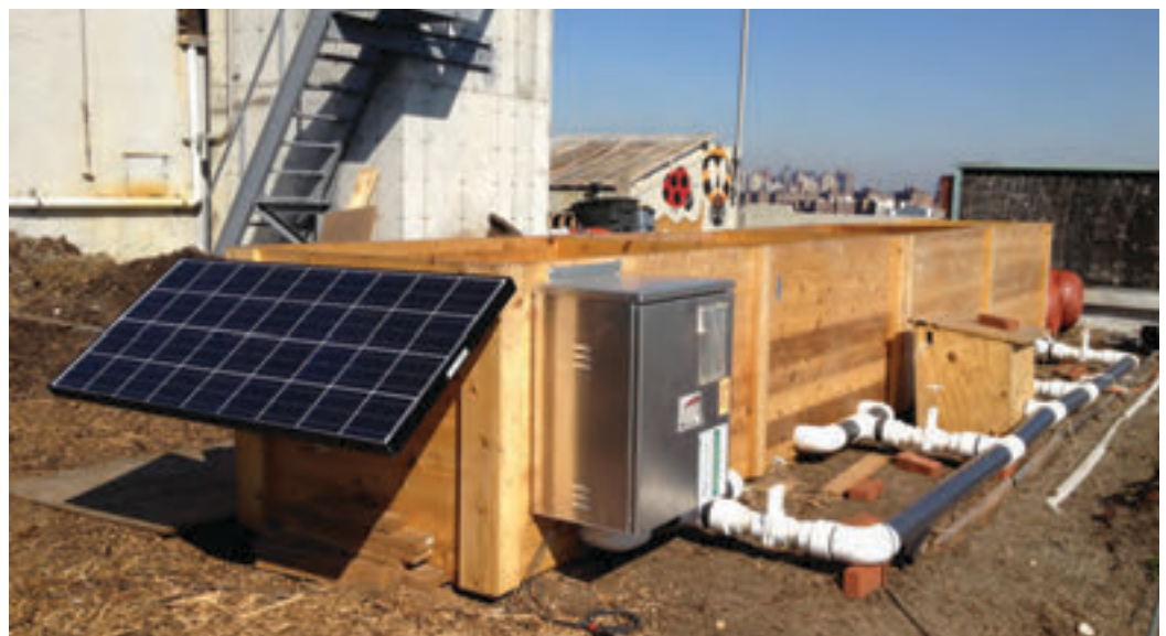
Solar-powered aerated static pile composting system built by the NYC Compost Project hosted by Build It Green!NYC at Brooklyn Grange's rooftop farm in Long Island City, Queens.
