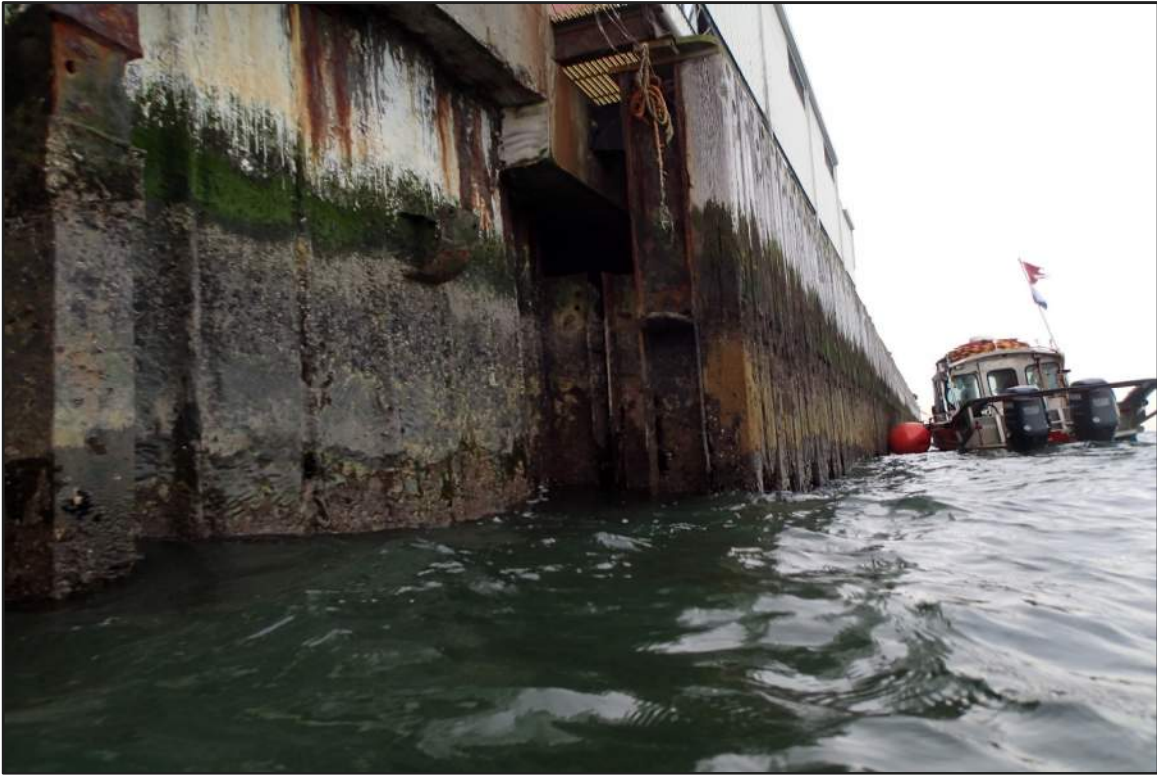
Photograph 5: West Bulkhead – Transition between West Bulkhead and North Pier steel sheet pile cofferdams (Looking west)
