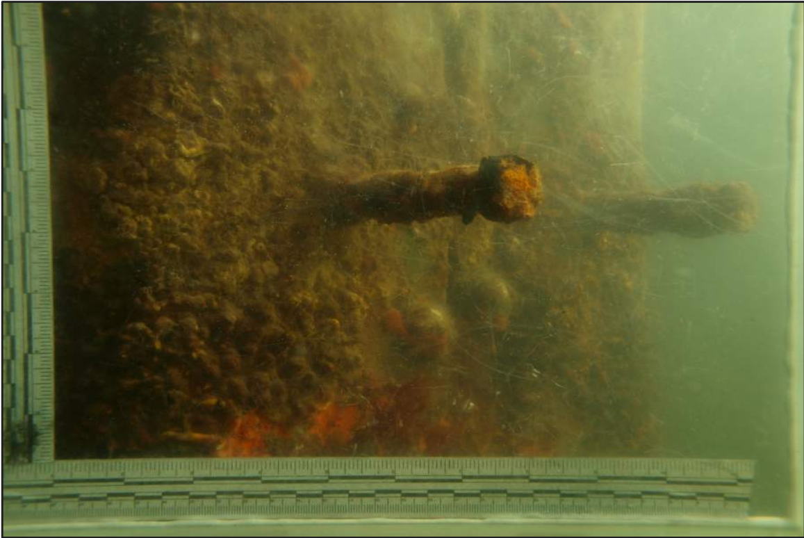
Photograph 17: North Bulkhead –Elevation of shear bolts below wale system on outer flanges
