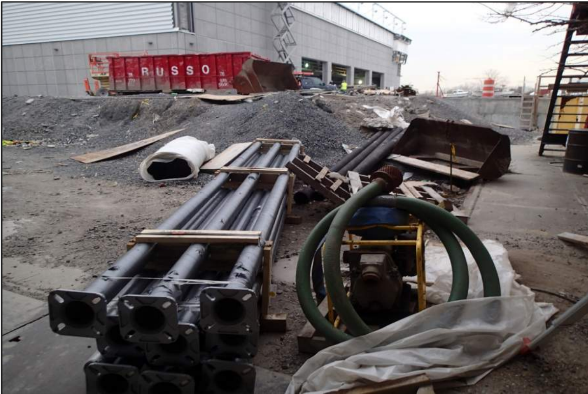
Photograph 38: North Bulkhead – Construction material storage in area of cofferdam cell hatches Note: Previous inspections found no access to sand fill (Looking southeast)
