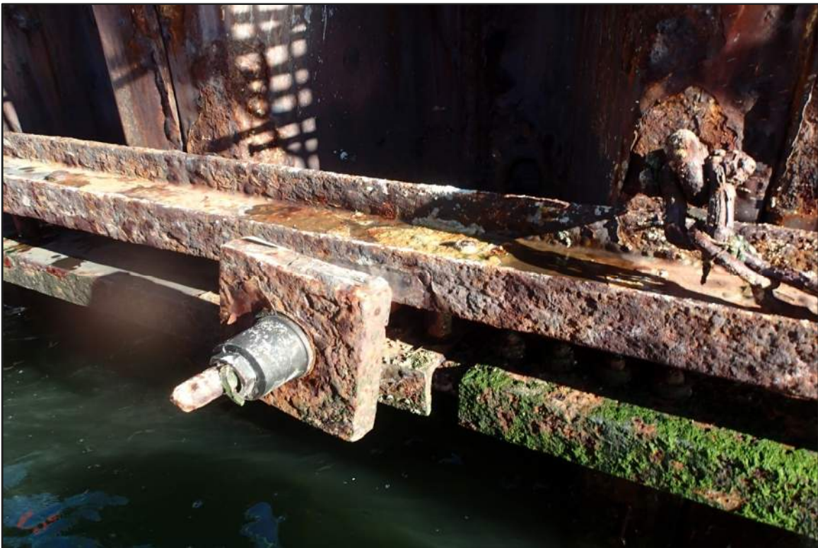
Photograph 34: North Bulkhead – Isolated disengaged tie-back anchor and washer (Looking northeast)
