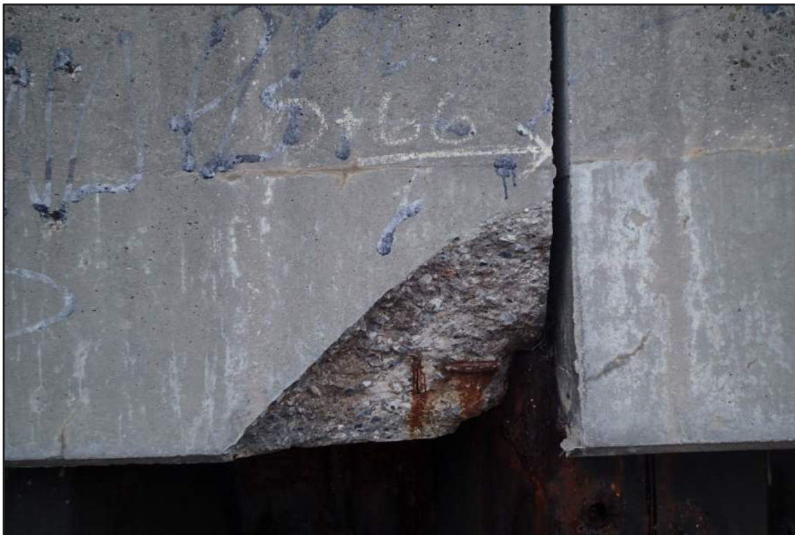
Photograph 41: East Bulkhead – Open spalling with exposed reinforcement at Sta. 0+66(Looking north)
