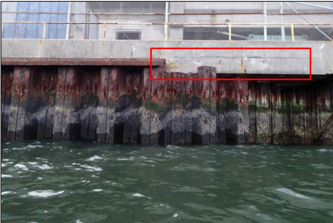
Photograph 30: West Bulkhead - Missing steel pile cap (Looking south)
