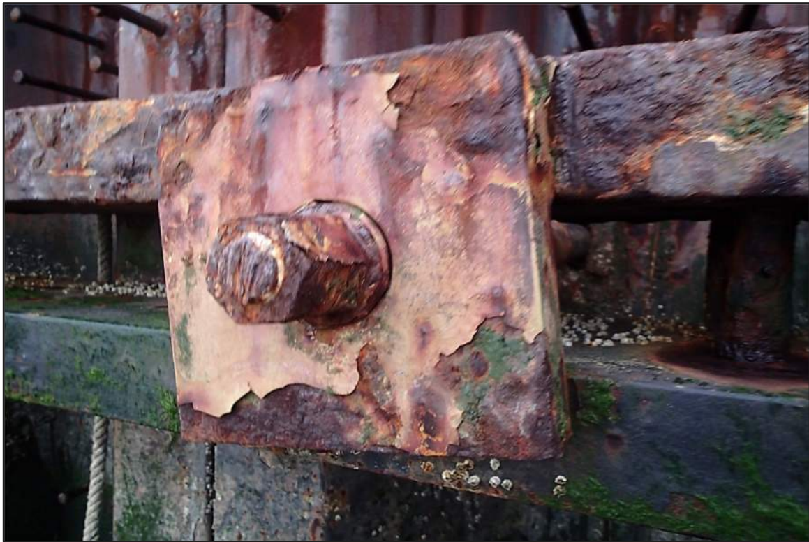
Photograph 9: North Bulkhead - Typical steel double channel wale, anchor rod, and hardware (Looking southeast)
