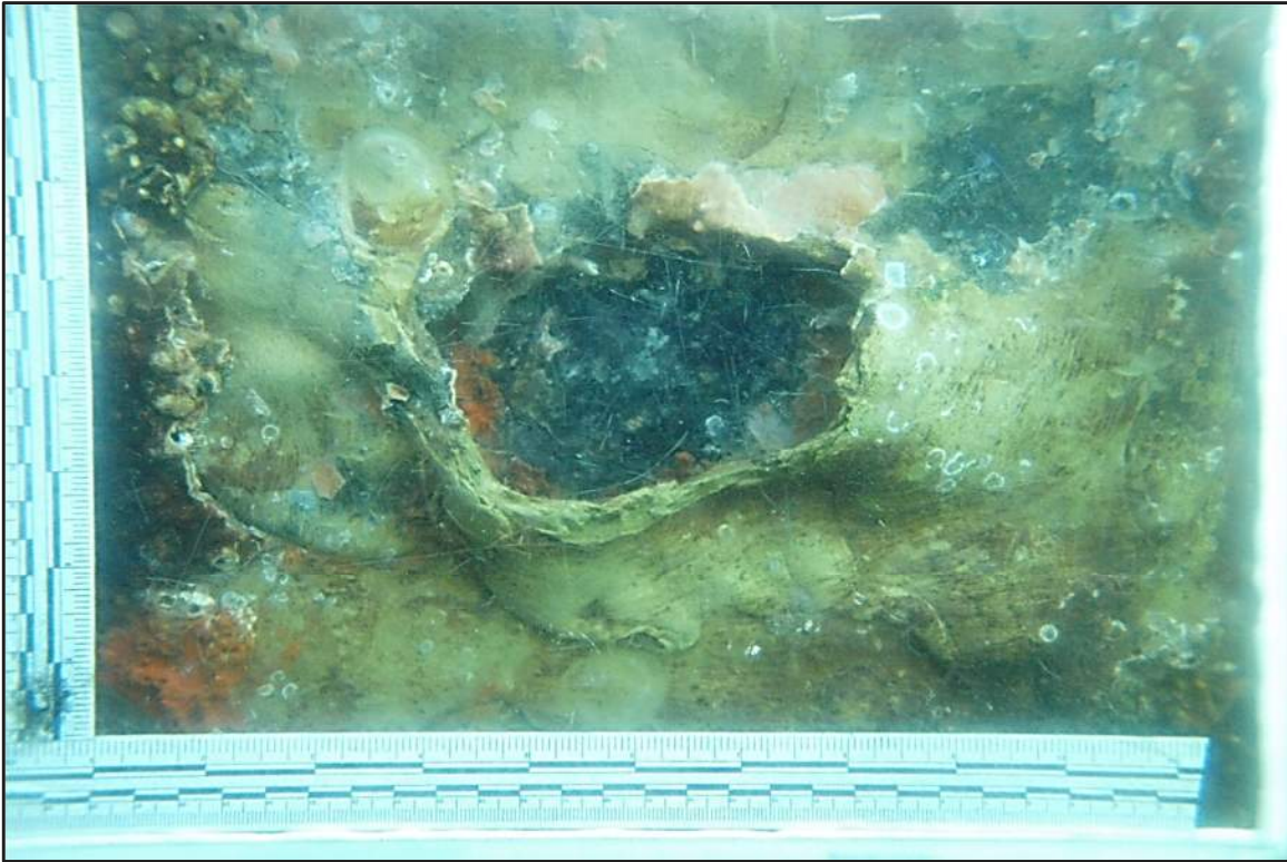
Photograph 29: West Bulkhead – Typical splash zone repair failure with moderate corrosion of exposed steel sheet pile
