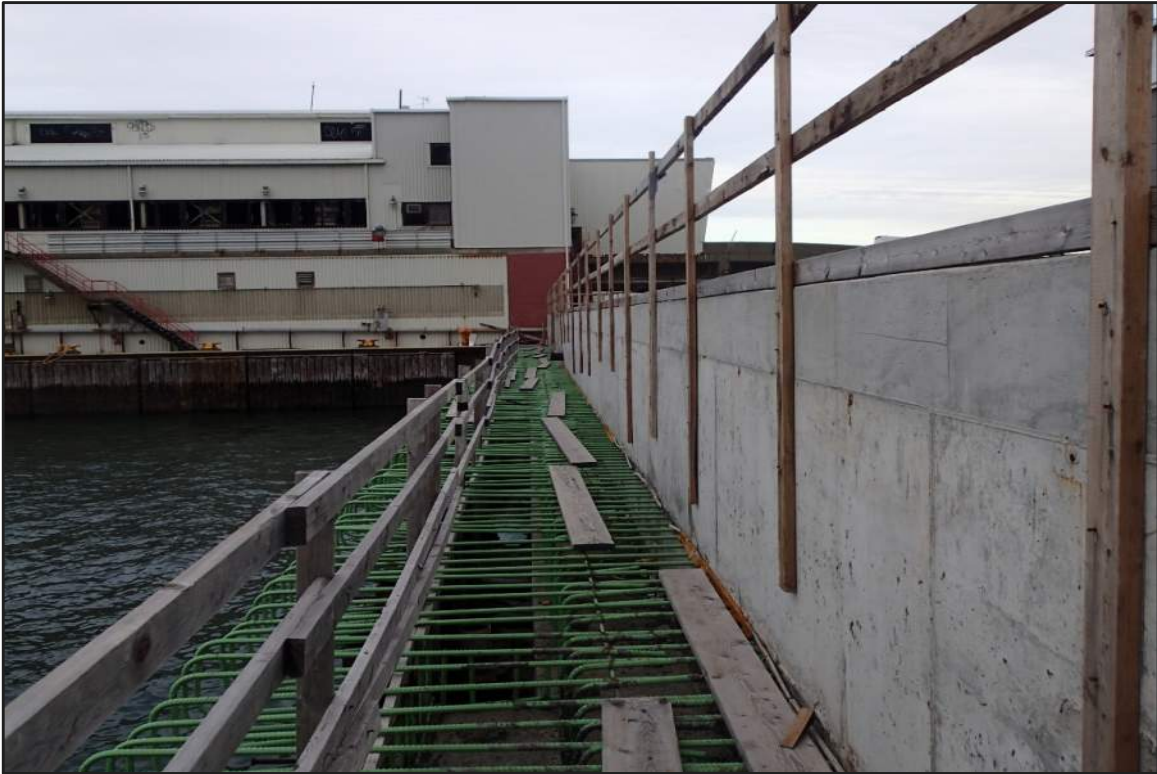
Photograph 13: North Bulkhead – Partially constructed structure with exposed epoxy coated reinforcement (looking north)
