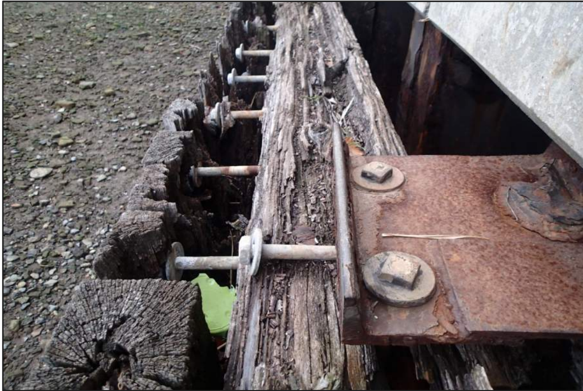
Photograph 43: East Bulkhead - Failed timber fender system connections due to rot (Looking west)
