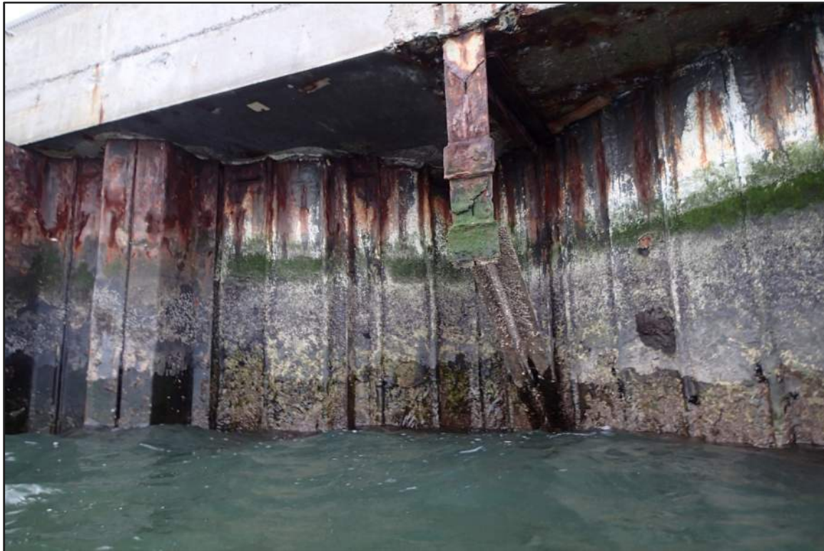
Photograph 4: West Bulkhead - Steel sheet pile cell interface with steel sheet pile bulkhead (looking southeast)
