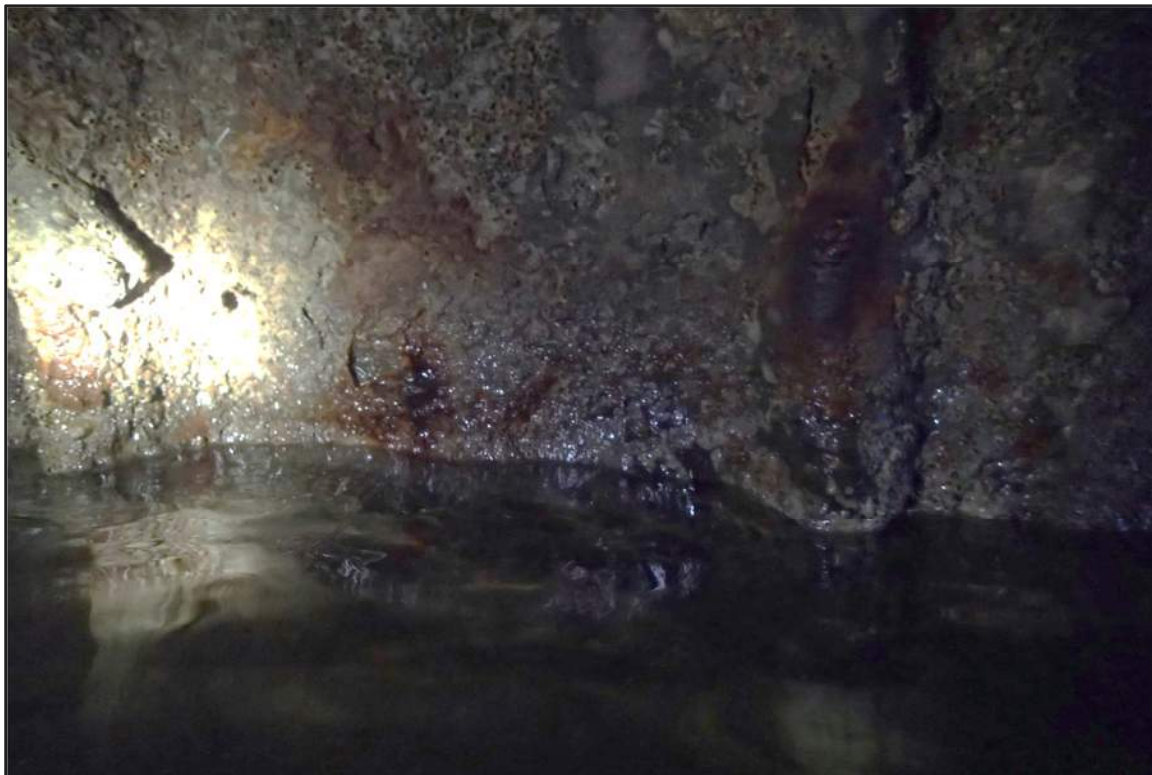
Photograph 36: North Bulkhead - Typical isolated epoxy failures with corrosion of steel cellular cofferdam in tidal zone (Looking east)
