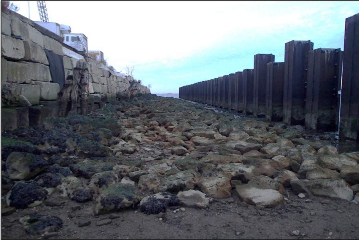
Photograph 21: Overview of revetment and steel sheet piles extending offshore from intersection of North and East Bulkheads (Looking west)
