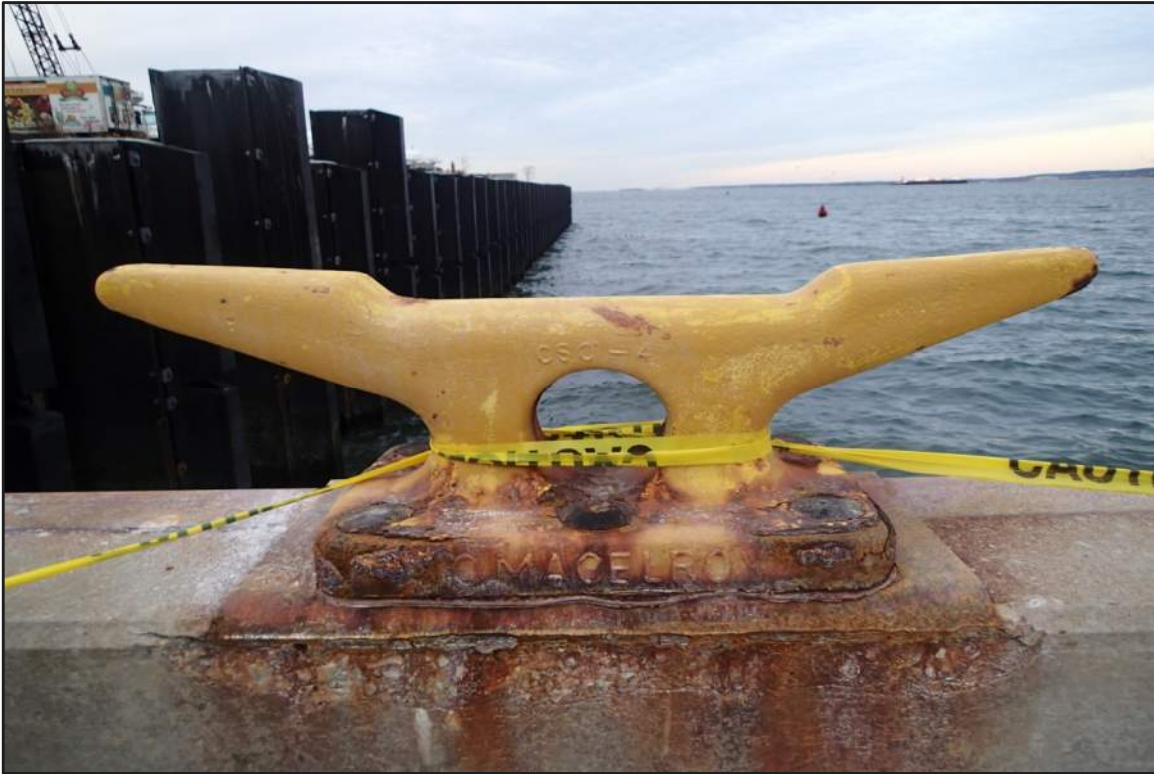
Photograph 37: North Bulkhead - Typical light to moderate corrosion of mooring hardware cleat (Looking west)
