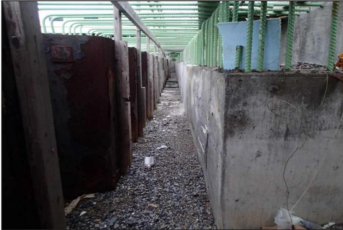
Photograph 11: North Bulkhead – Concrete bulkhead with partially filled annulus between concrete and steel sheet pile bulkheads (Looking north)
