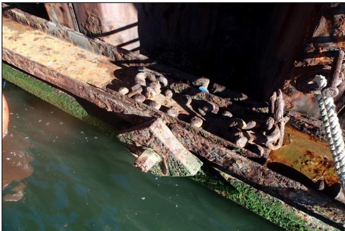
Photograph 32: North Bulkhead - Typical coating failure with moderate corrosion of steel channel wale, anchor rod, and hardware in splash/tidal zone
