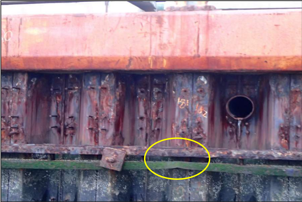
Photograph 33: North Bulkhead – Impacted steel wale at approximate Station 0+65 (Looking east)
