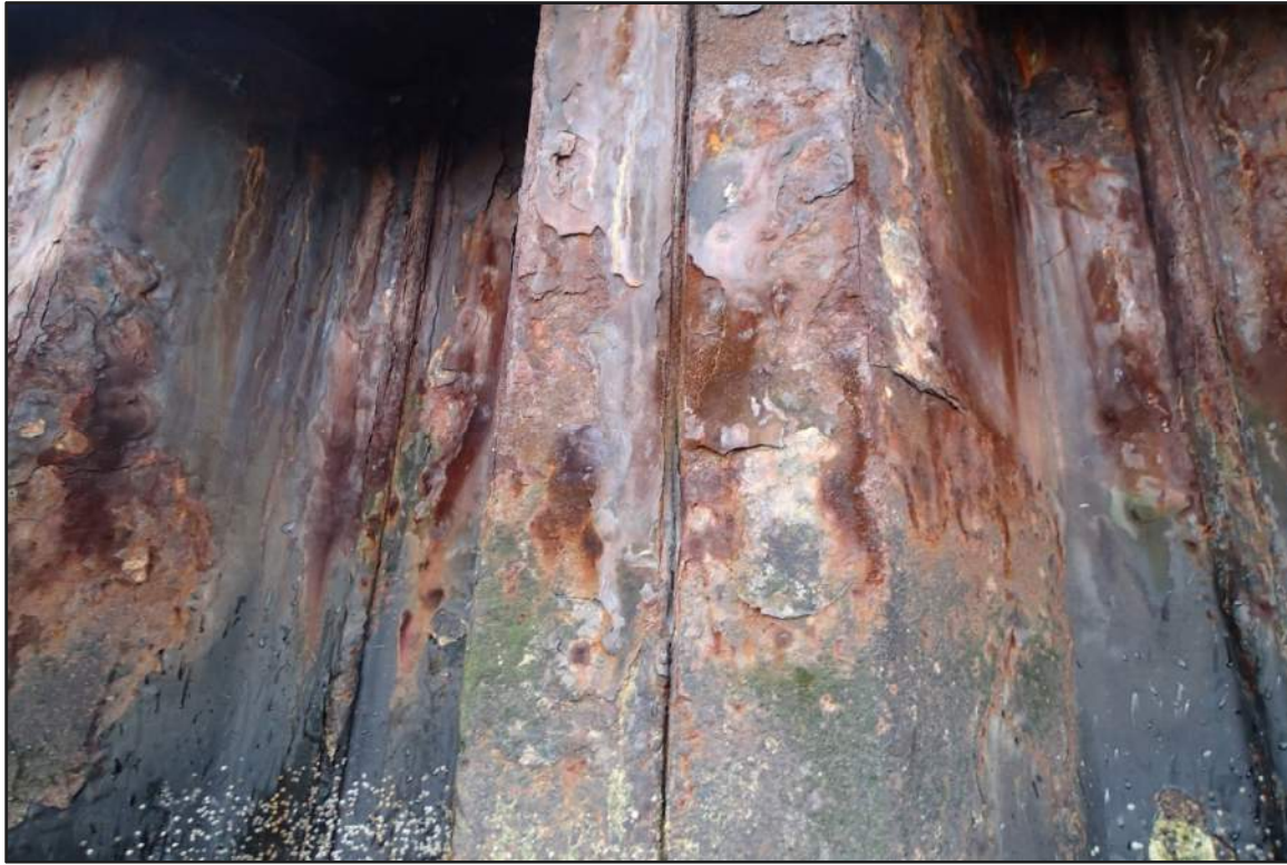
Photograph 27: West Bulkhead – Typical coating failure with moderate corrosion of steel sheet pile in splash/tidal zone (Looking southeast)
