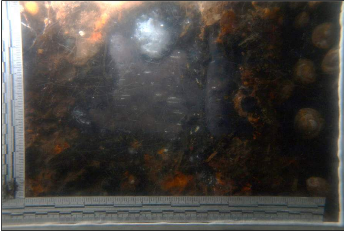
Photograph 35: North Bulkhead - Isolated coating failure with moderate corrosion of steel sheet pile below water
