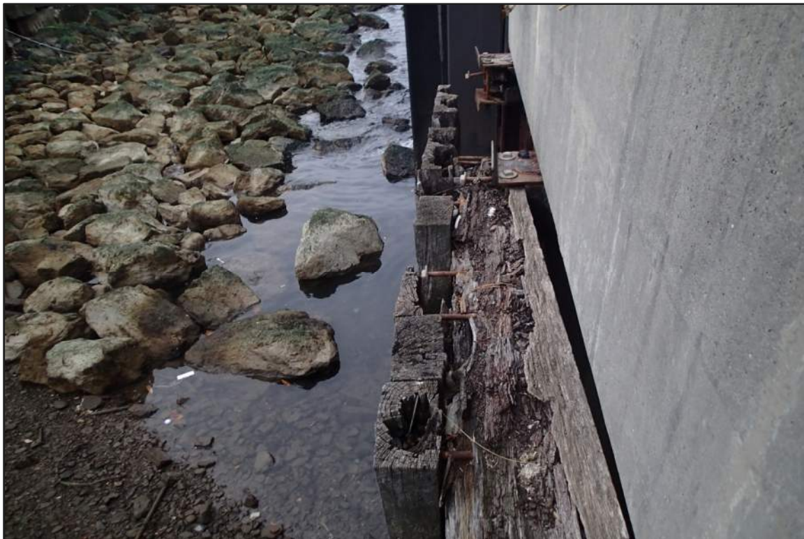
Photograph 44: East Bulkhead - Heavy rot of the upper timber horizontal wale and panels (Looking west)
