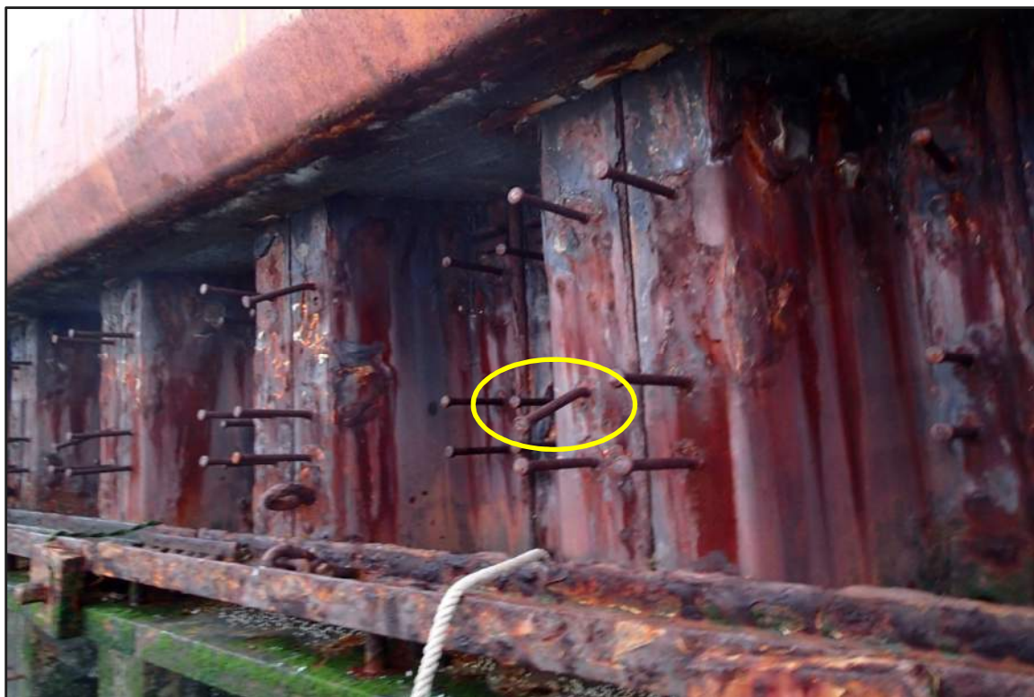
Photograph 31: North Bulkhead - Typical coating failure with moderate corrosion of steel sheet pile in splash/tidal zone and an isolated damaged shear stud (Looking northeast)
