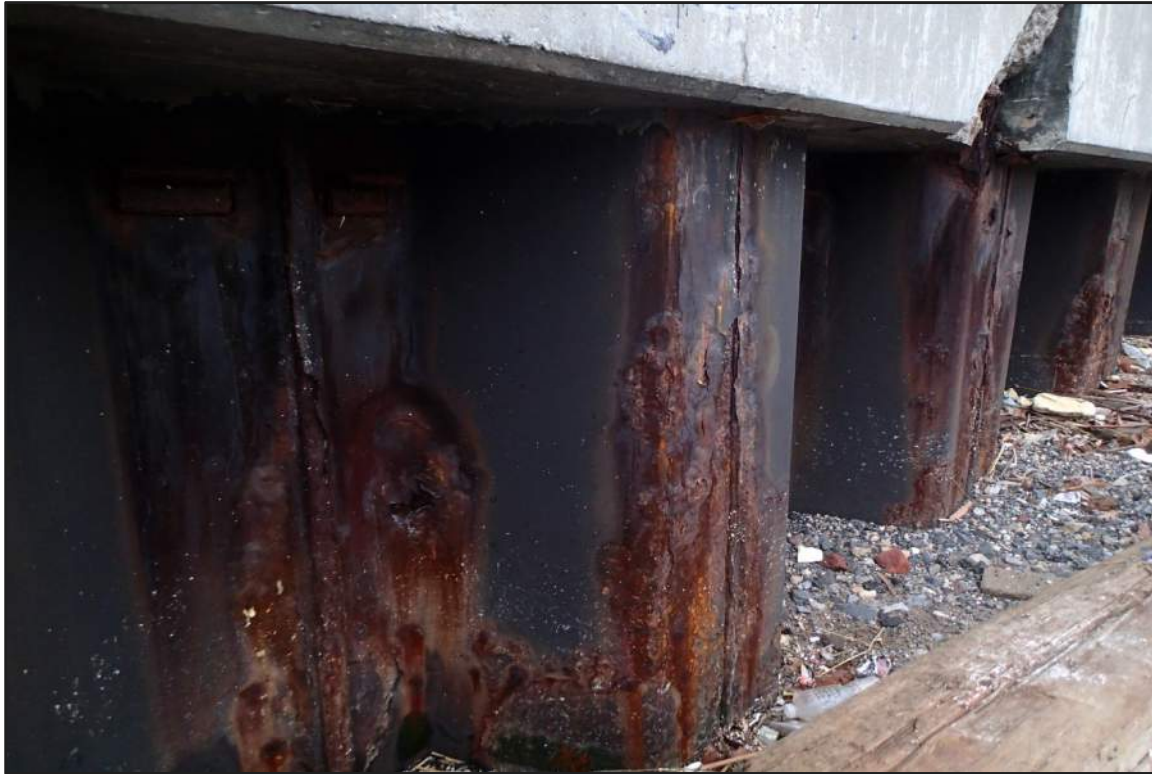
Photograph 39: East Bulkhead - Typical coating failure and moderate corrosion in the splash/tidal zone (Looking northeast)
