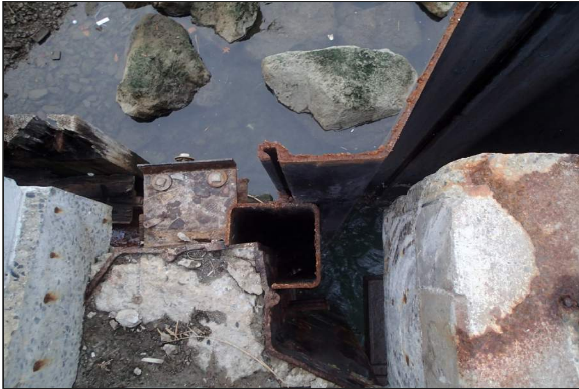
Photograph 15: North Bulkhead – Deck demolition at North and East bulkhead interface to install transition element for new steel sheet pile to the west
