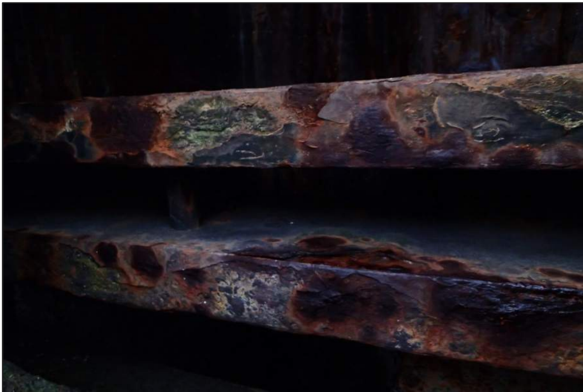
Photograph 42: East Bulkhead - Typical coating failure with moderate corrosion of steel channel wale inshore of timber fender system in splash/tidal zone (Looking north)
