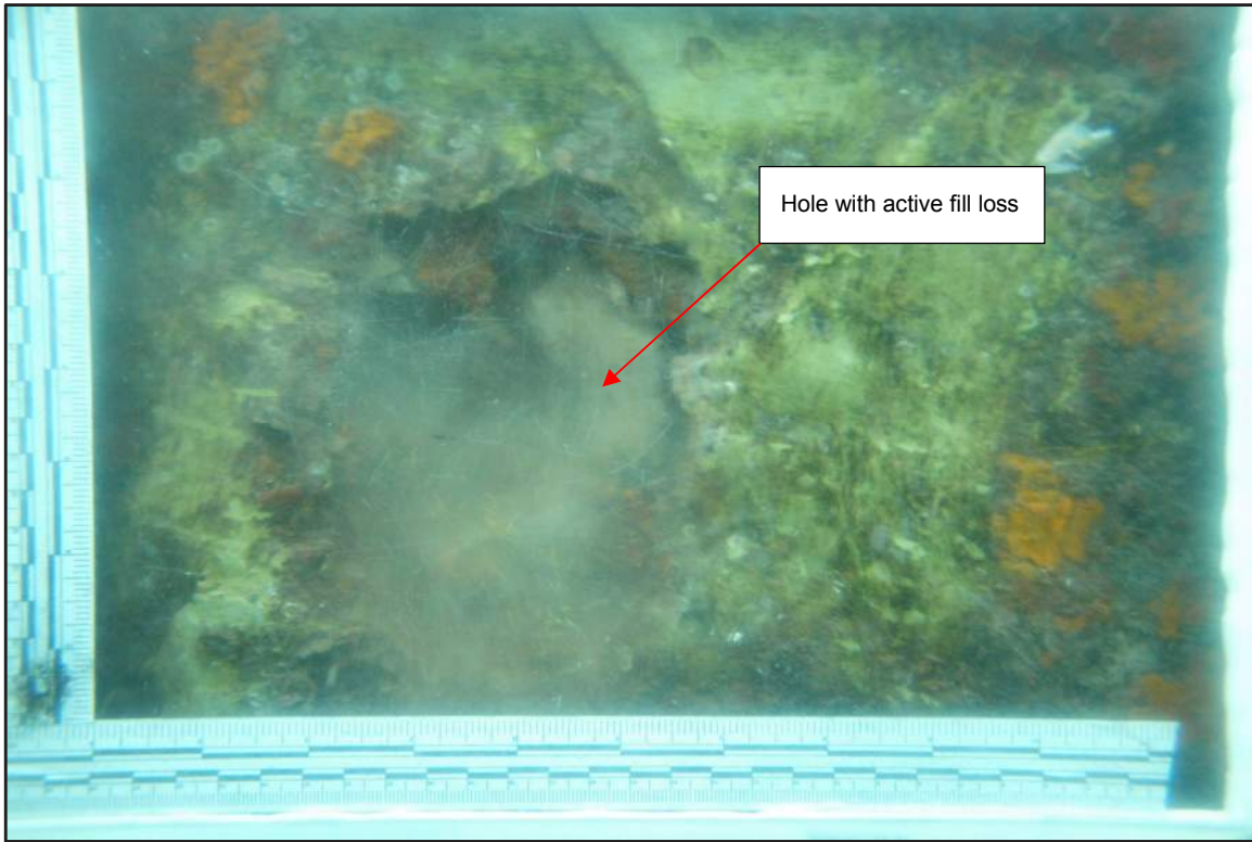
Photograph 25: West Bulkhead – Hole through splash zone repair and steel sheet pile cell with exposed fill and active fill loss at intermediate cell adjacent to Cell F-1
