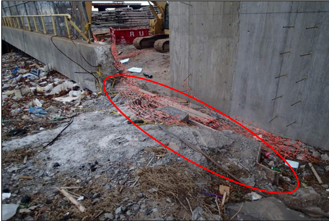
Photograph 23: East Bulkhead – Exposed steel sheet pile bulkhead where curb and deck are removed (Looking northwest)
