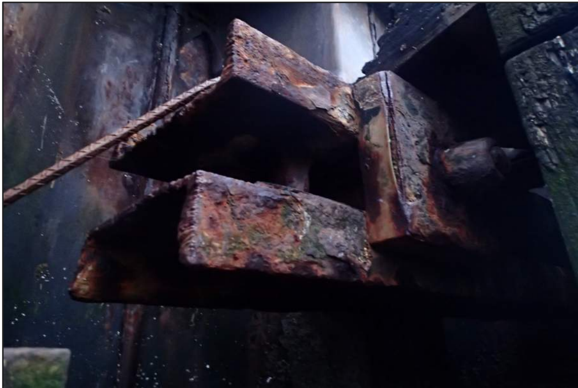
Photograph 40: East Bulkhead - Typical coating failure with moderate corrosion of steel channel wale, anchor rod, and hardware in splash/tidal zone (Looking northeast)
