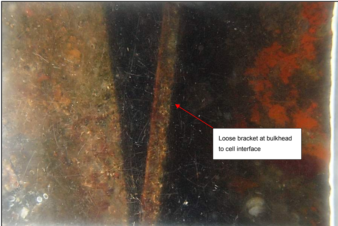
Photograph 26: West Bulkhead – Loose bracket at interface between steel sheet pile bulkhead and steel sheet pile cell
