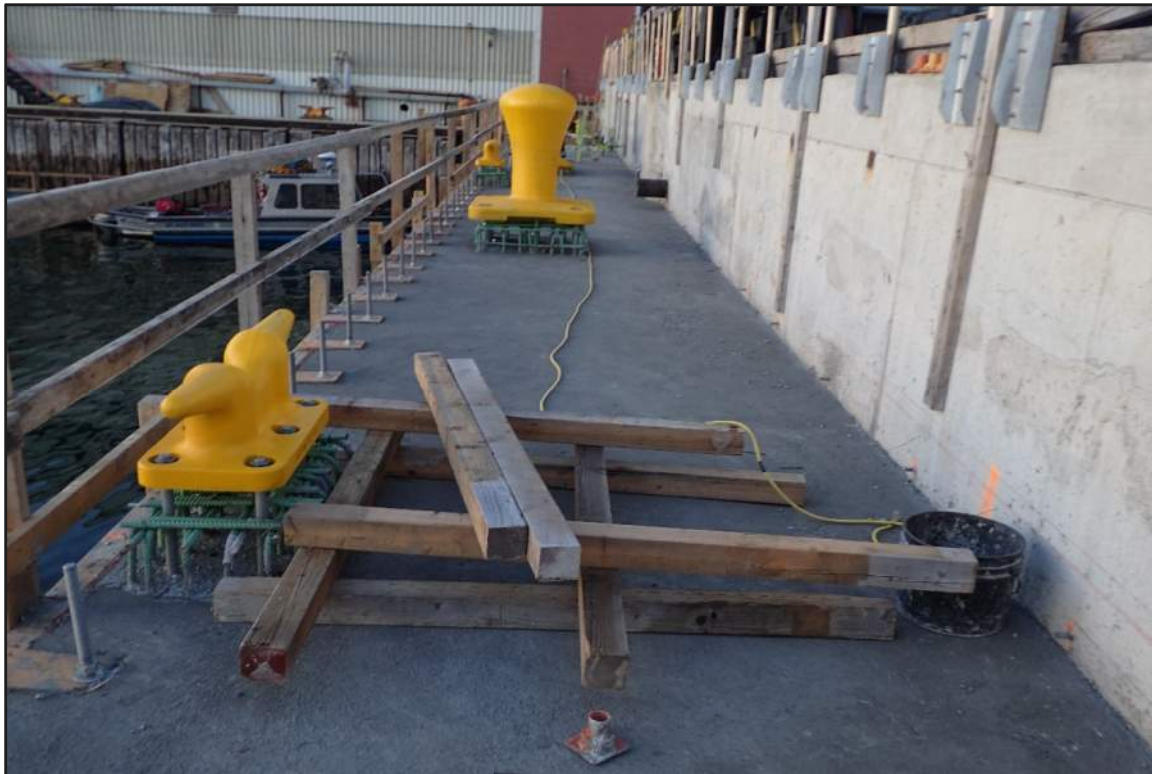
Photograph 14: North Bulkhead – Nearly fully constructed deck structure with exposed epoxy coated reinforcement at the base of the new mooring hardware installations (Looking north)
