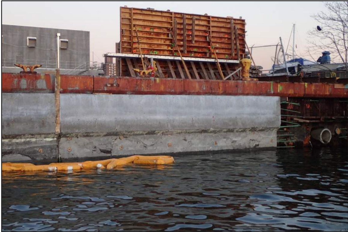
Photograph 23: North Bulkhead – Encased-to-exposed transition at south end of the North Bulkhead (Looking east)
