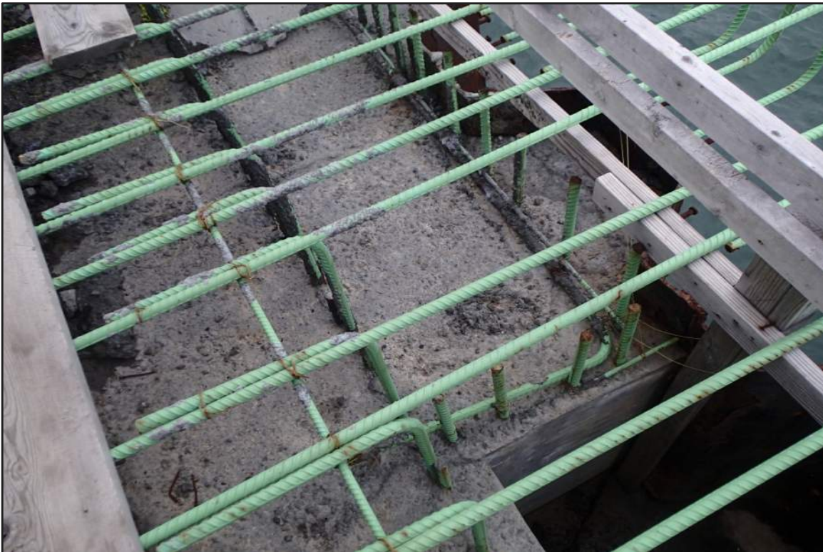
Photograph 12: North Bulkhead – Extended concrete bulkhead between Sta. 1+90 and 1+97 from 2016 inspection (Looking southwest)
