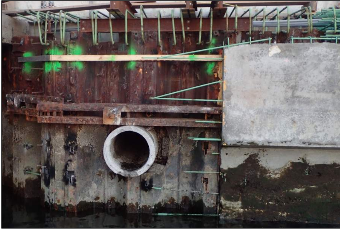
Photograph 21: North Bulkhead – Encased-to-exposed transition at north end of the North Bulkhead (Looking east)
