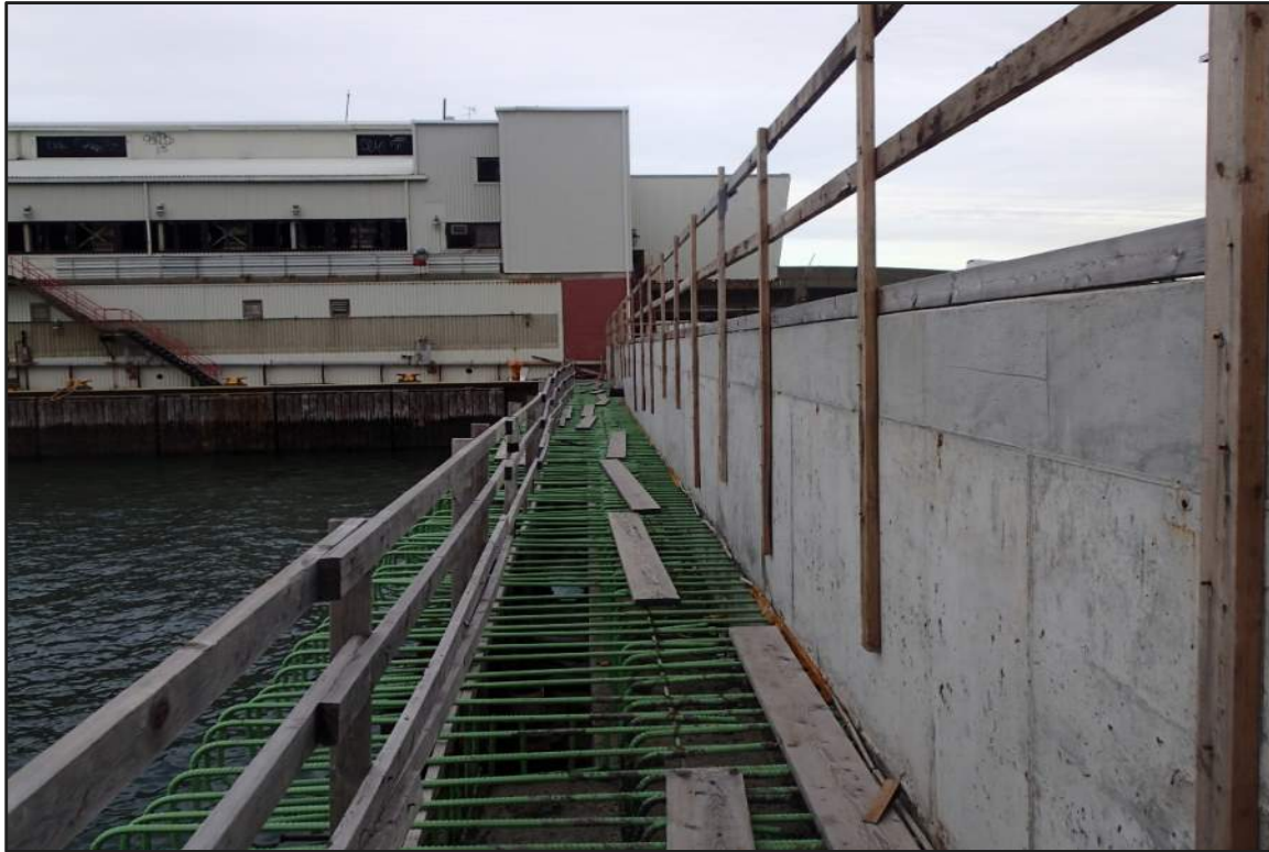
Photograph 13: North Bulkhead – Partially constructed structure from 2016 inspection with exposed epoxy coated reinforcement (Looking north)
