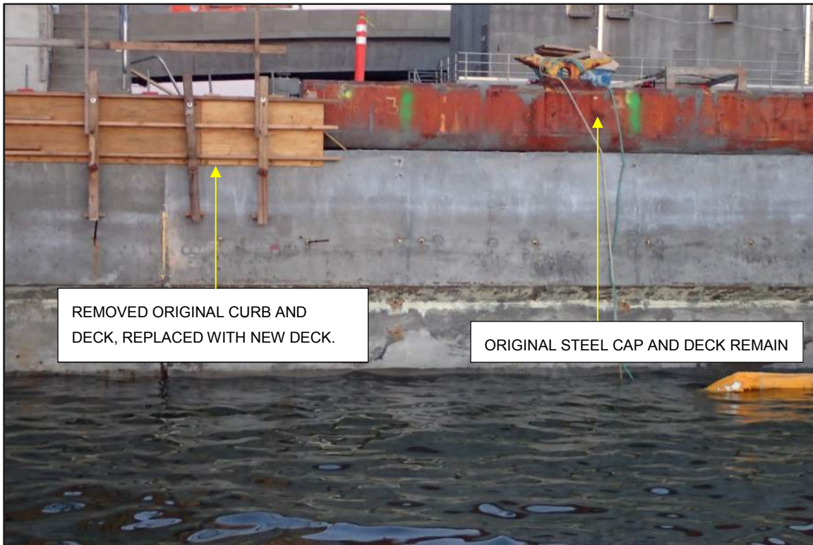
Photograph 10: North Bulkhead – Area of removed curb and deck replaced with new deck, which interfaces with an original steel cap (Looking northeast)
