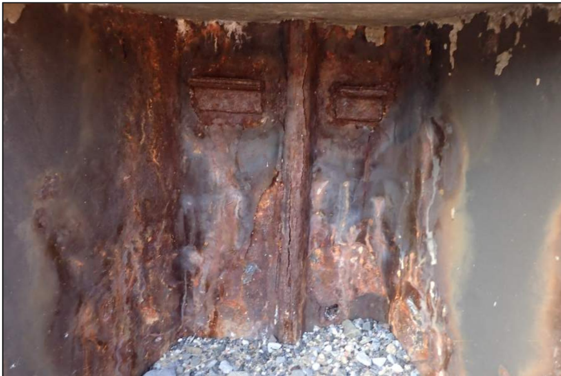
Photograph 46: East Bulkhead - Typical coating failure and moderate corrosion in the splash/tidal zone (Looking northwest)
