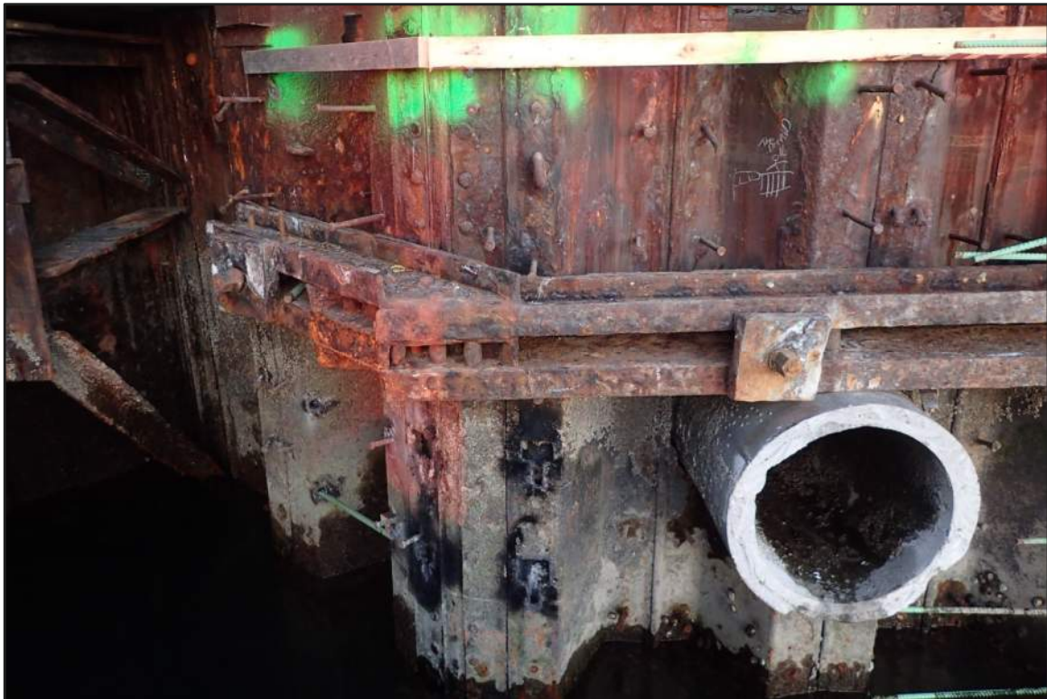
Photograph 40: North Bulkhead - Moderate to advanced corrosion of steel sheet in the splash zone and tidal zone in the areas still pending concrete encasement (Looking east)
