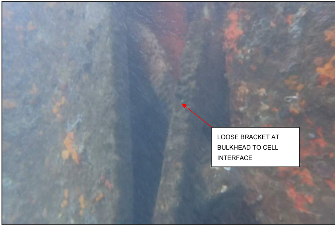
Photograph 29: West Bulkhead – Loose bracket at interface between steel sheet pile bulkhead and steel sheet pile cell
