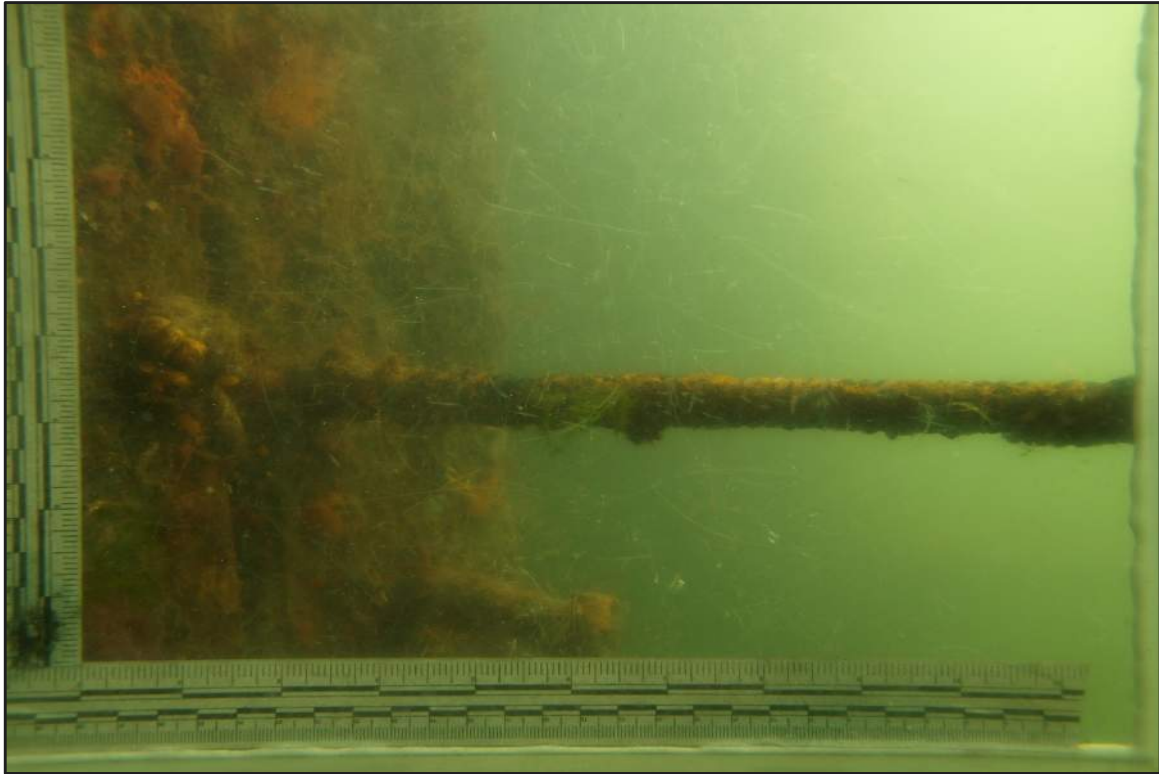
Photograph 19: North Bulkhead – Threaded rod installed between shear bolt elevations observed prior to installation of partial encasement during the 2016 inspection
