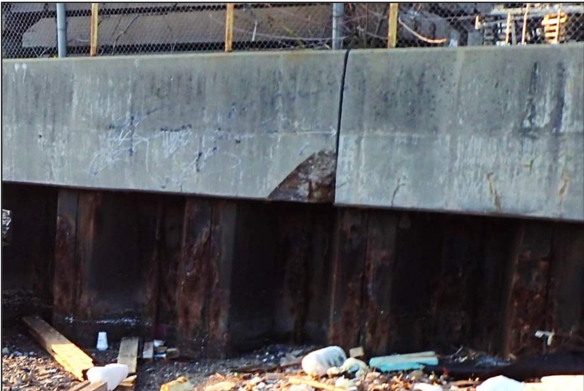
Photograph 48: East Bulkhead – Open spalling with exposed reinforcement at Sta. 0+66 (Looking northwest)
