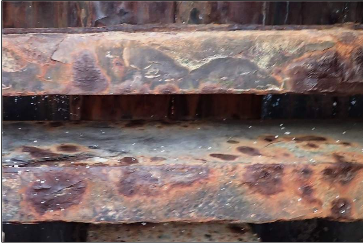
Photograph 49: East Bulkhead - Typical coating failure with moderate corrosion of steel channel wale inshore of timber fender system in splash/tidal zone (Looking north)
