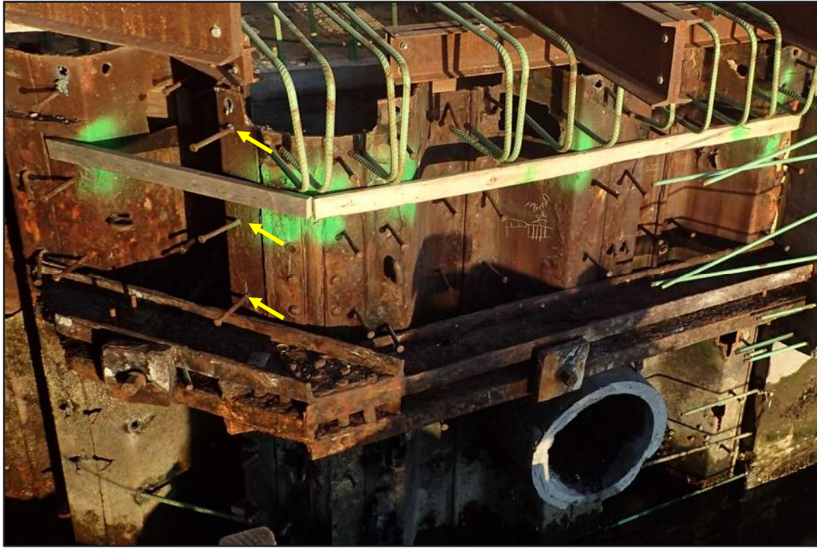
Photograph 17: North Bulkhead – Typical shear bolt installation above water on exposed steel sheet piles (Looking southeast)
