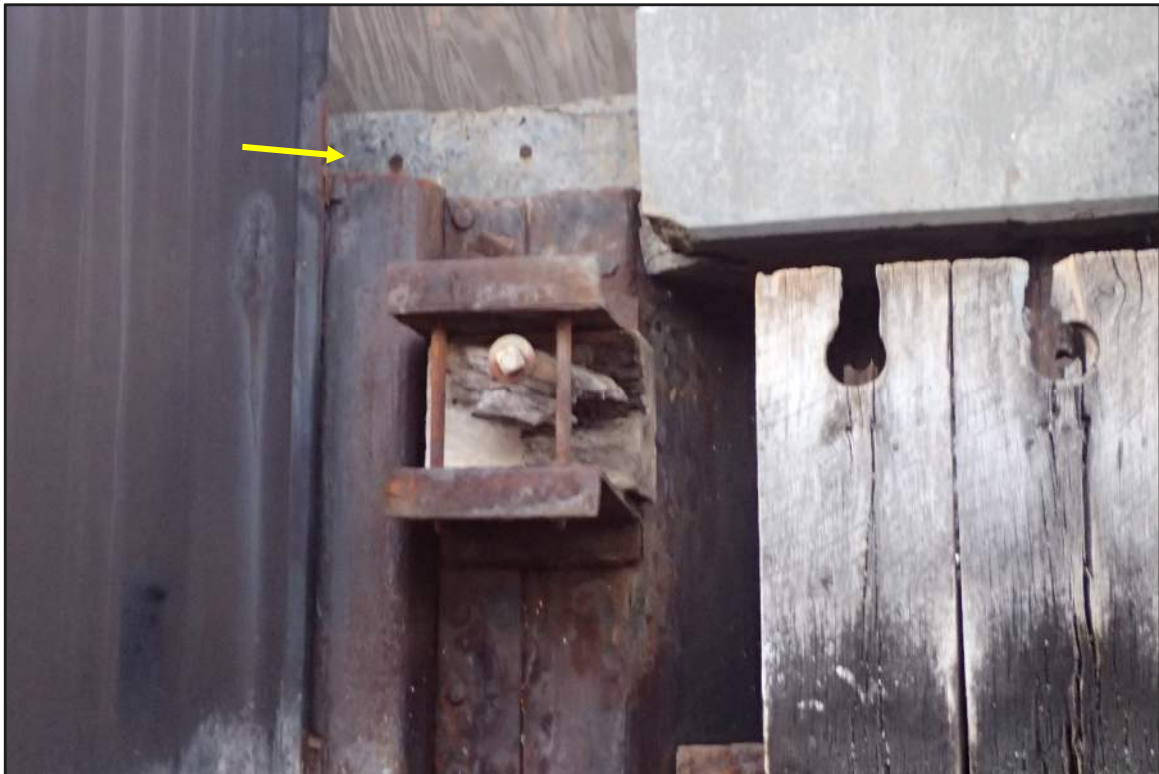
Photograph 16: North Bulkhead – Deck demolition at North and East bulkhead interface to install transition element for new steel sheet pile to the west
