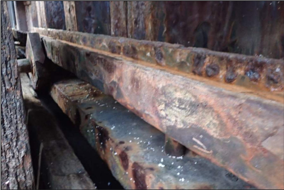
Photograph 47: East Bulkhead - Typical coating failure with moderate corrosion of steel channel wale, anchor rod, and hardware in splash/tidal zone (Looking southwest)
