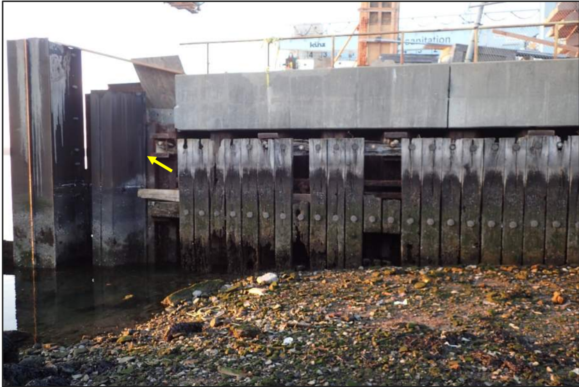
Photograph 15: North Bulkhead – Interface between North and East bulkheads and steel sheet pile fender and revetment retaining structure to the west (Looking northwest)
