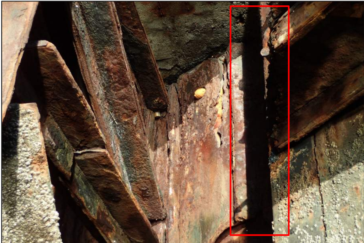
Photograph 8: North Bulkhead – Transition from steel sheet pile cell to steel sheet pile bulkhead (Looking east)
