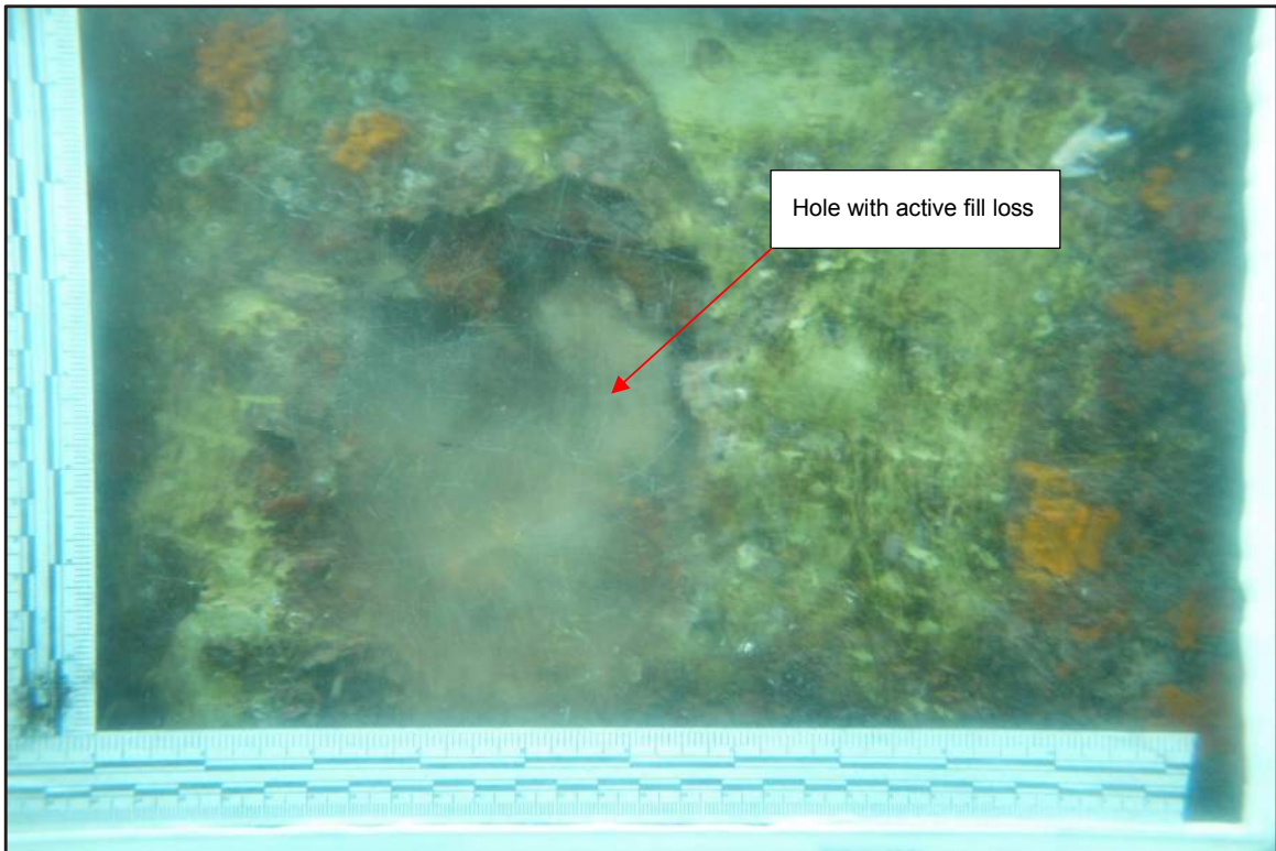
Photograph 28: West Bulkhead – Hole through splash zone repair and steel sheet pile cell with exposed fill and active fill loss at intermediate cell adjacent to Cell F-1 observed in 2016 inspection
