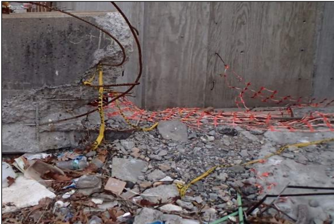
Photograph 26: East Bulkhead – Demolished concrete curb and deck at Sta. 0+14 (photograph reference from 2016 inspection) (Looking north)
