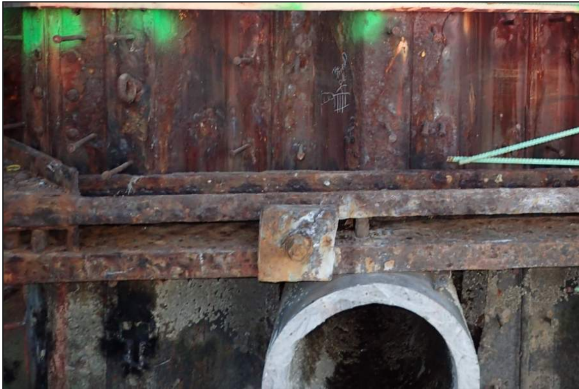
Photograph 34: North Bulkhead - Typical coating failure with moderate corrosion of steel channel wale, anchor rod, and hardware in splash/tidal zone that is not yet encased in concrete (Looking east)
