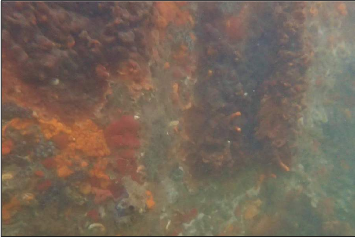
Photograph 31: West Bulkhead – Typical isolated coating loss on steel sheet pile bulkhead below water
