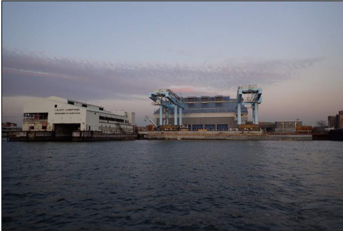
Photograph 1: Former southwest Brooklyn Marine Transfer Station and ongoing inshore construction (Looking east)
