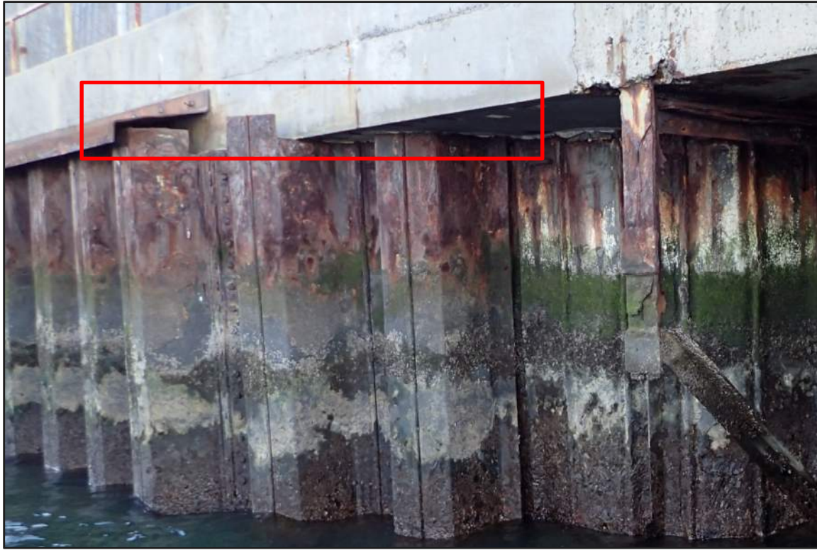
Photograph 33: West Bulkhead - Missing steel pile cap (Looking southeast)
