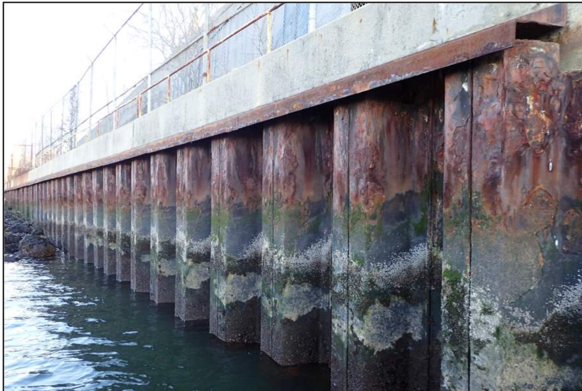
Photograph 30: West Bulkhead – Typical coating failure with moderate corrosion of steel sheet pile in splash/tidal zone (Looking east)
