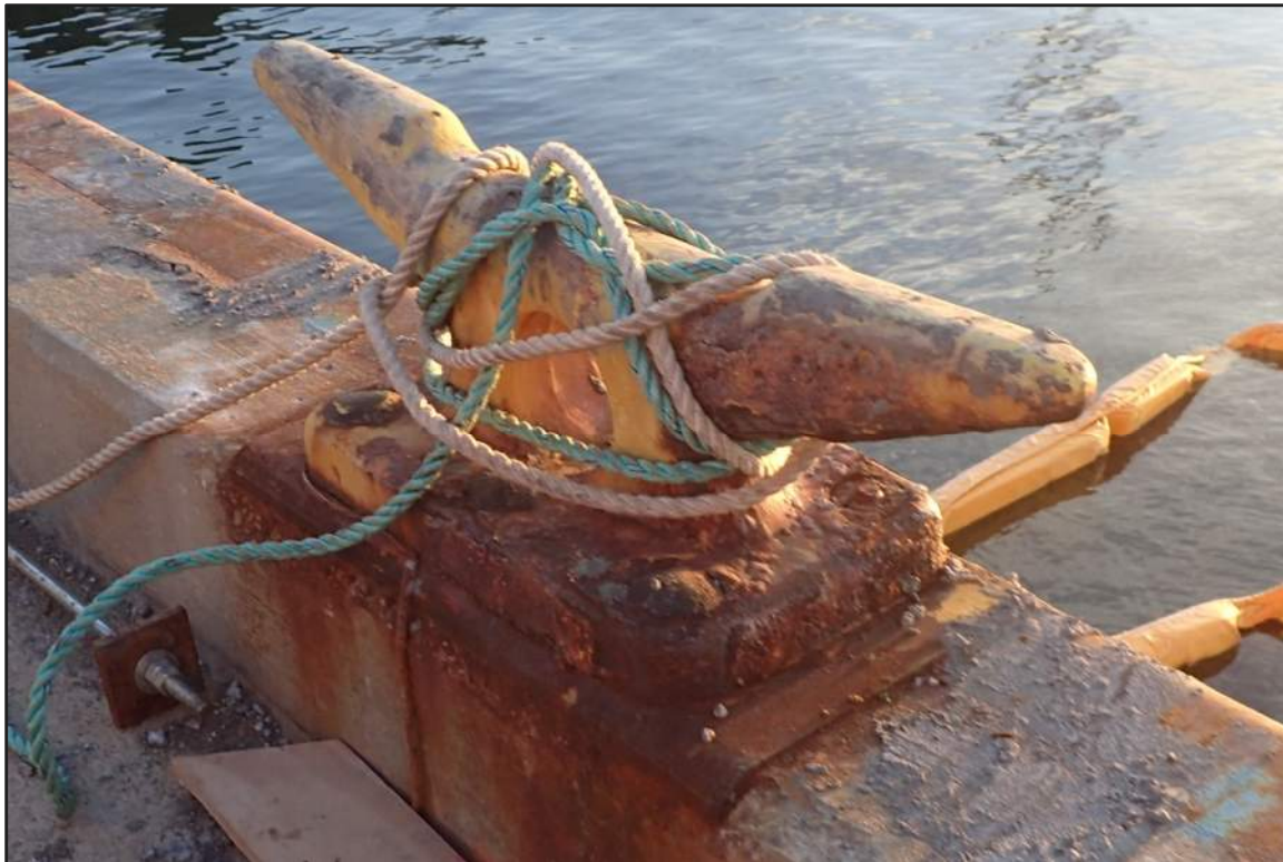
Photograph 42: North Bulkhead – Typical moderate corrosion of original vintage mooring hardware cleat (Looking south)
