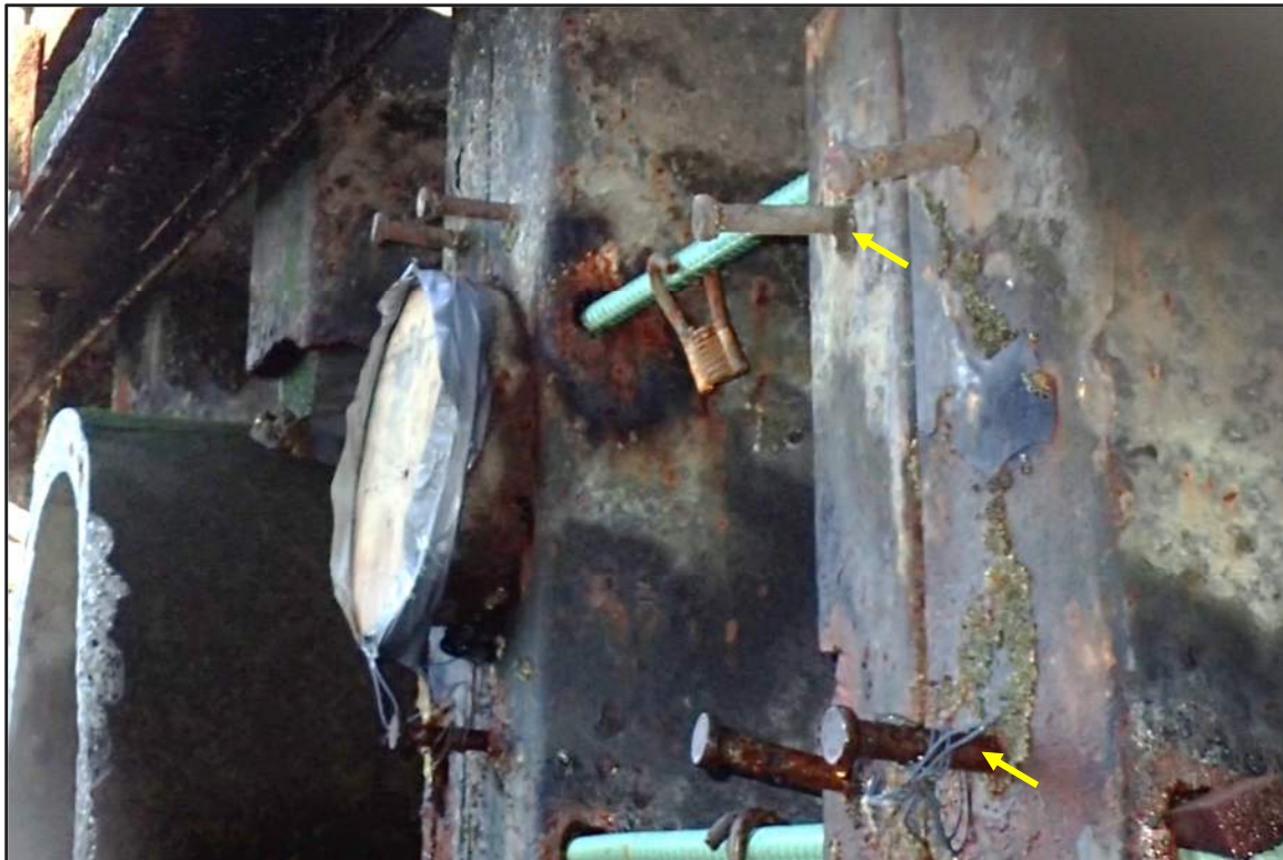
Photograph 18: North Bulkhead –Elevation of shear bolts below wale system on outer flanges
