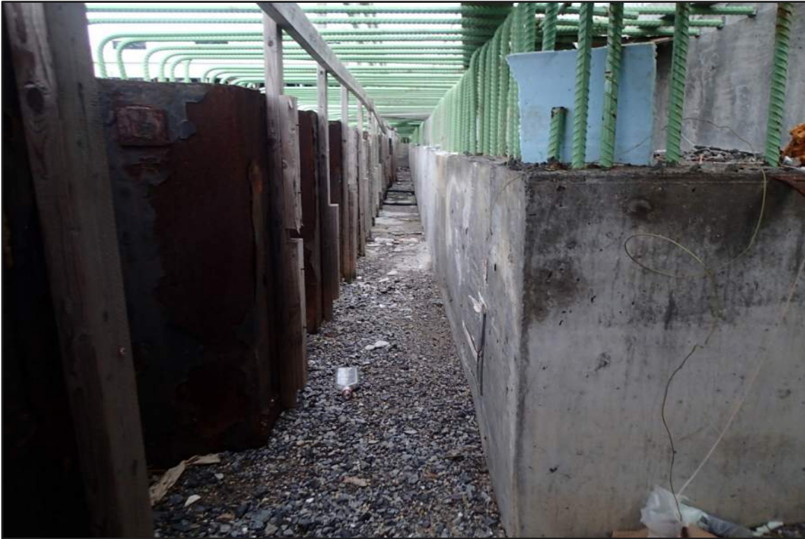
Photograph 11: North Bulkhead – Concrete bulkhead with partially filled annulus between concrete and steel sheet pile bulkheads from 2016 inspection (Looking north)
