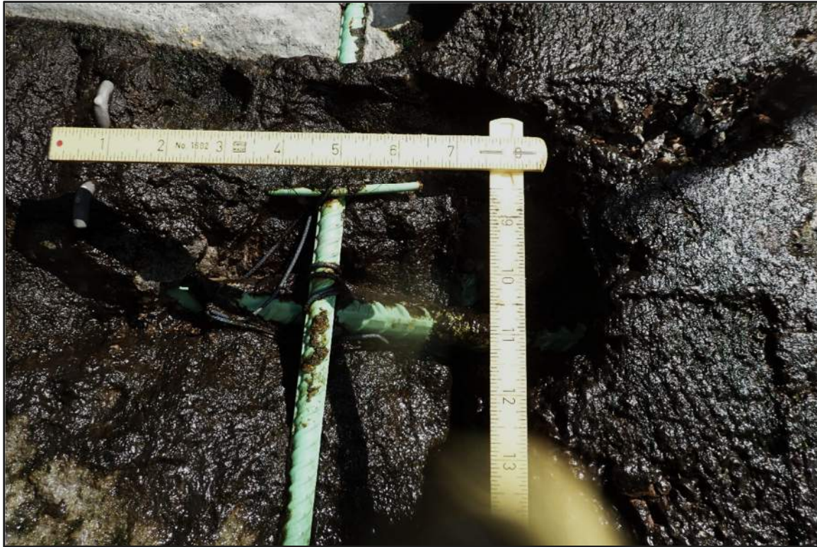
Photograph 37: North Bulkhead – Poor consolidation of the concrete at the vertical cold joints of the partial concrete encasement (Looking east)
