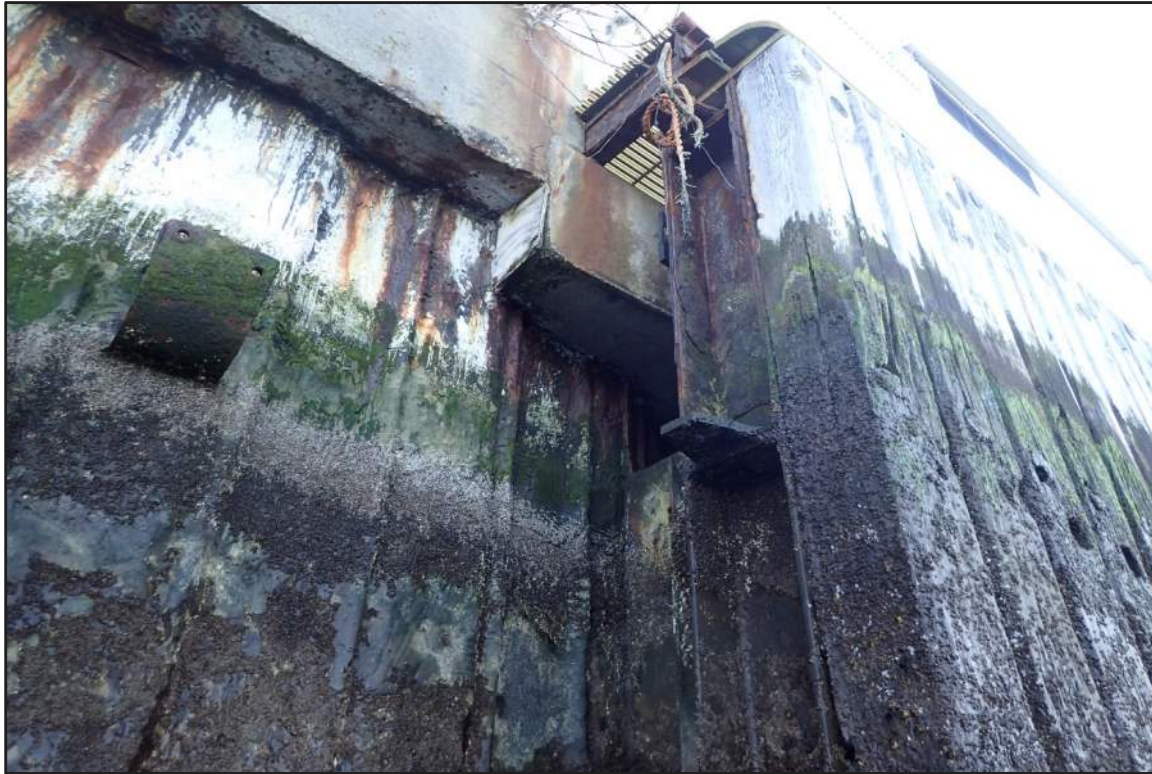
Photograph 5: West Bulkhead – Transition between West Bulkhead and North Pier steel sheet pile cofferdams (Looking southwest)
