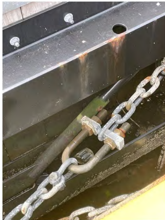
Photo No. 2 – General Conditions of Bracing Chains
