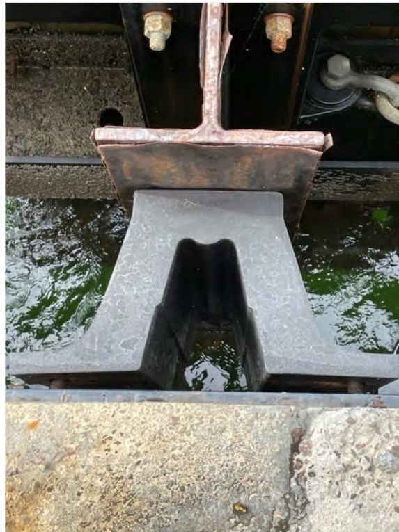
Photo No. 4 – Anchor Bolts from Fender to Base Plate are loose. Rubber Fender no longer flush with concrete wall. Typical from Fenders No. 13-20.
