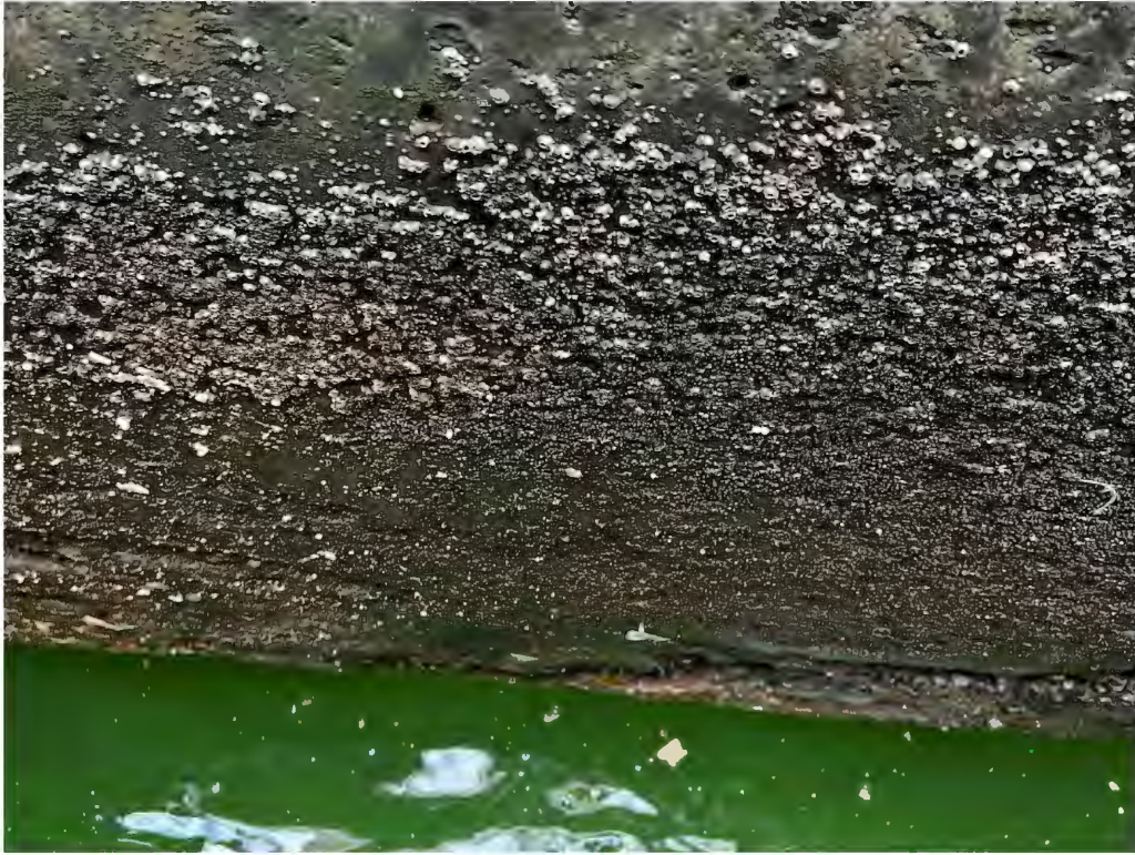
Photo No. 7 – Crack at concrete bulkhead spanning the width of Fender No. 12.
