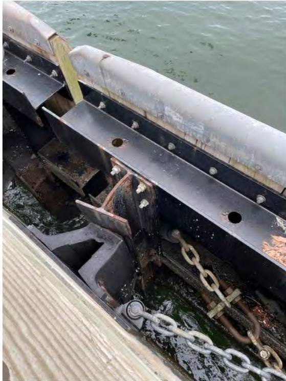
Photo No. 5 – H-Pile, Timbers and Deformed at Fender No. 9 as a result of Impact.
