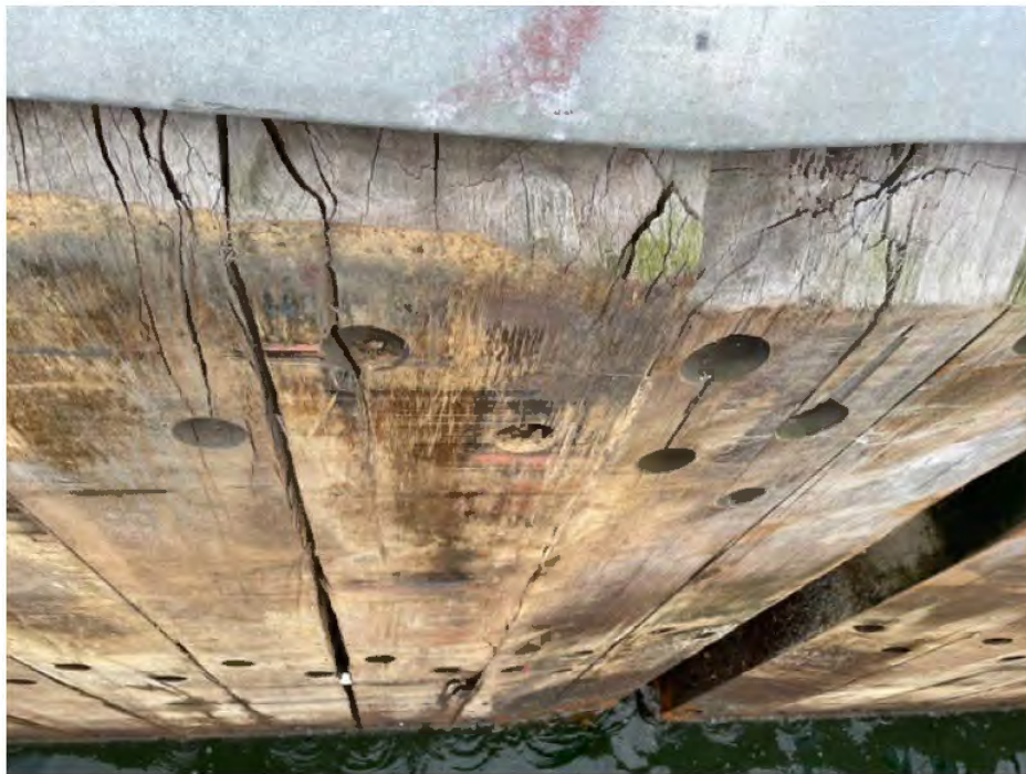
Photo No. 6 – Timber cracked at Fender No. 7 as result of impact.
