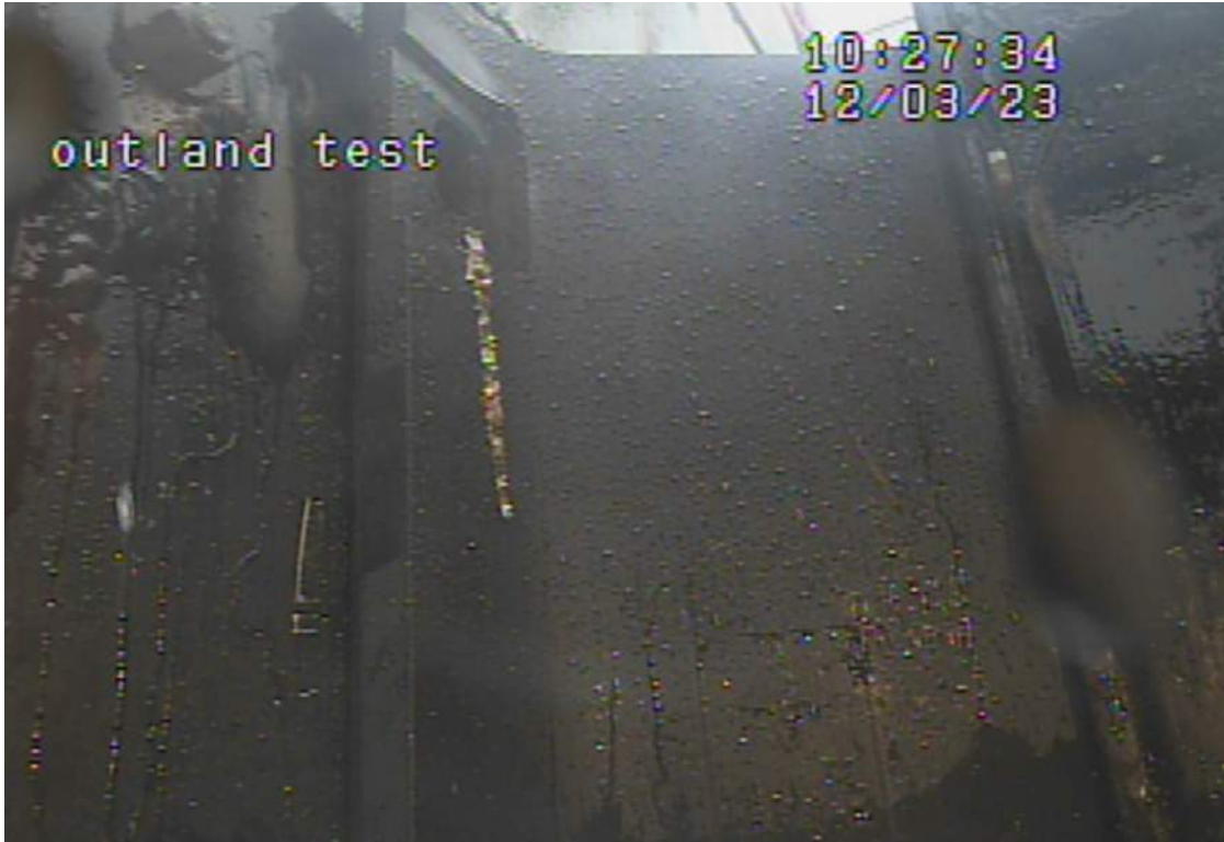
Photo 18. Bolt and washer missing at the connection rubber fender to HP pile at fender #8
