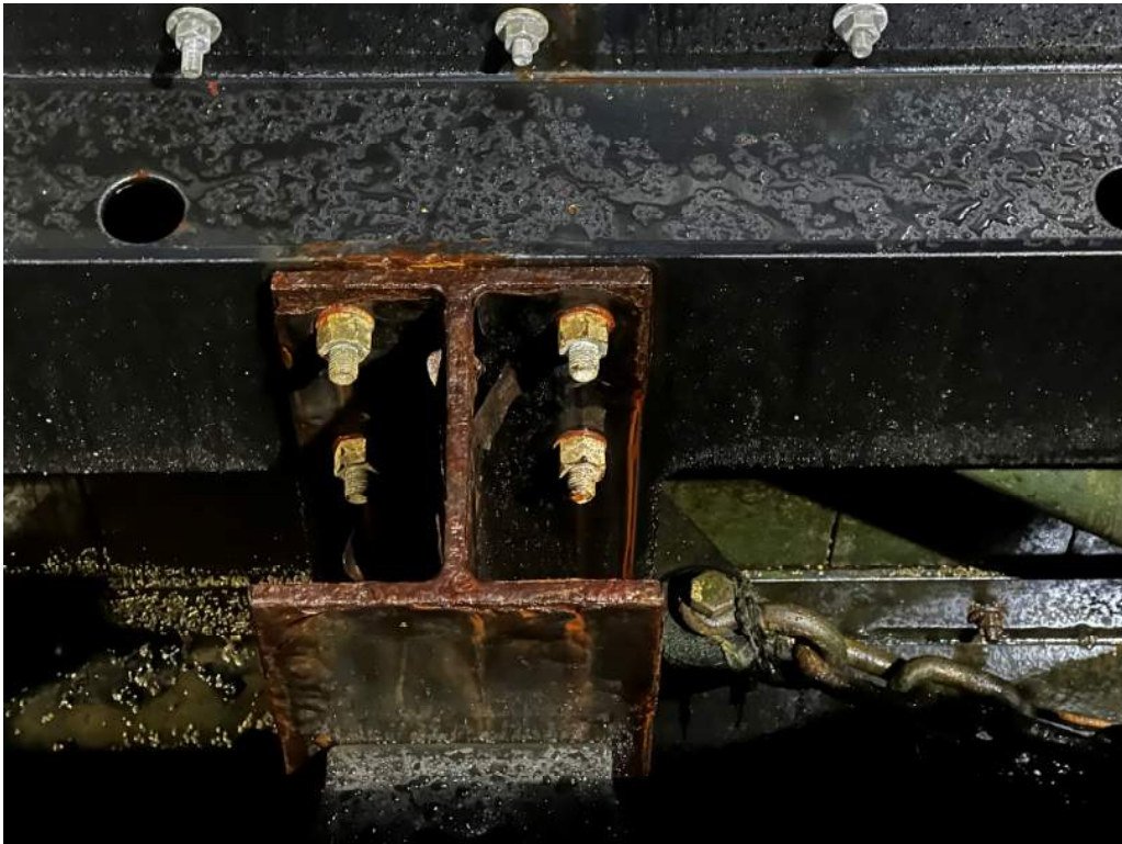
Photo 4. Typical corrosion at top of HP Piles.
