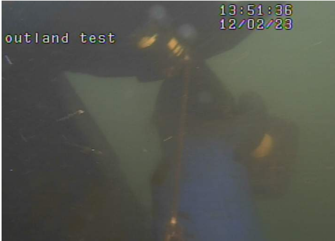
Photo 7. Rubber Fender Peeling Off.
