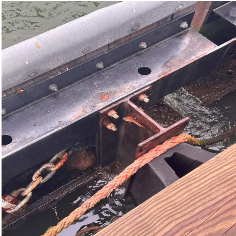
Photo 8. Corrosion at HP Pile.
