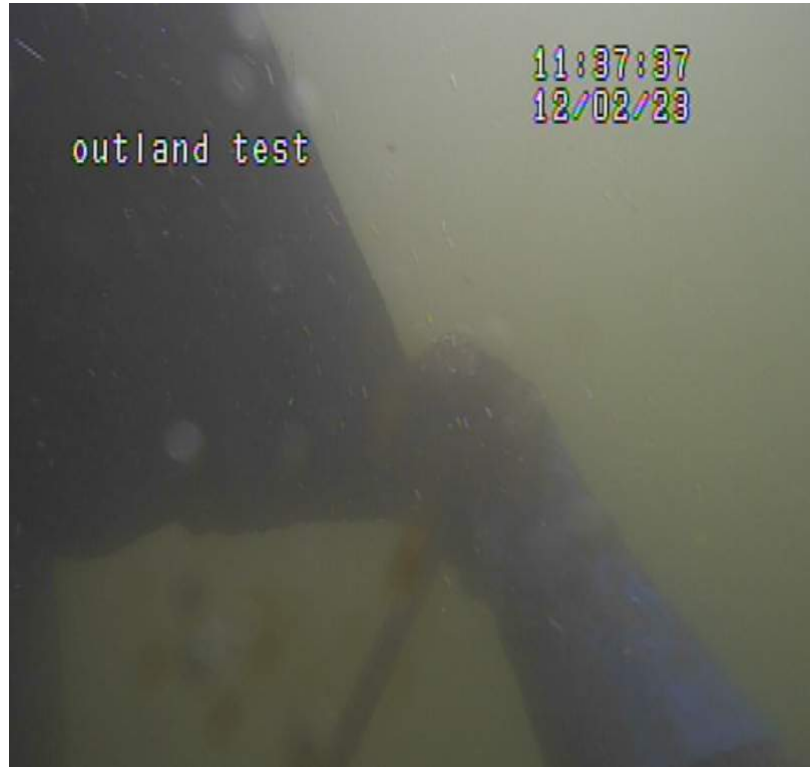
Photo 4. Rubber Fender Peeling Off.
