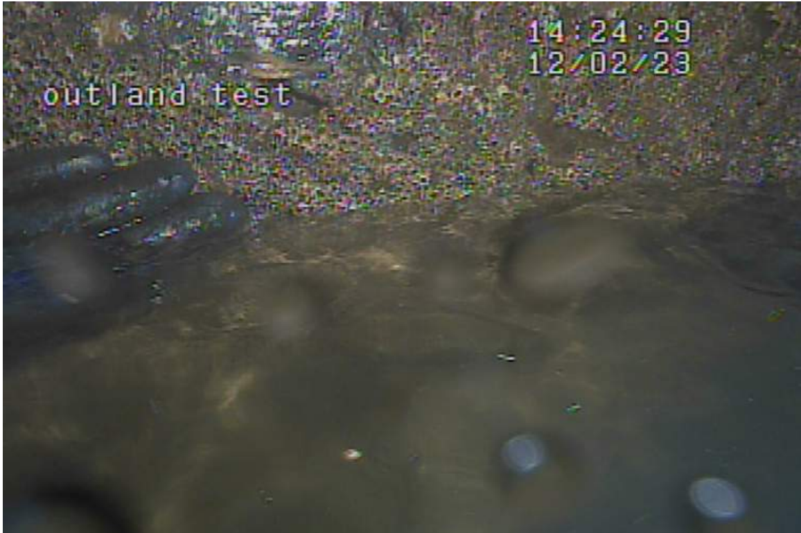
Photo 9. Typical divet at Concrete Bulkhead.
