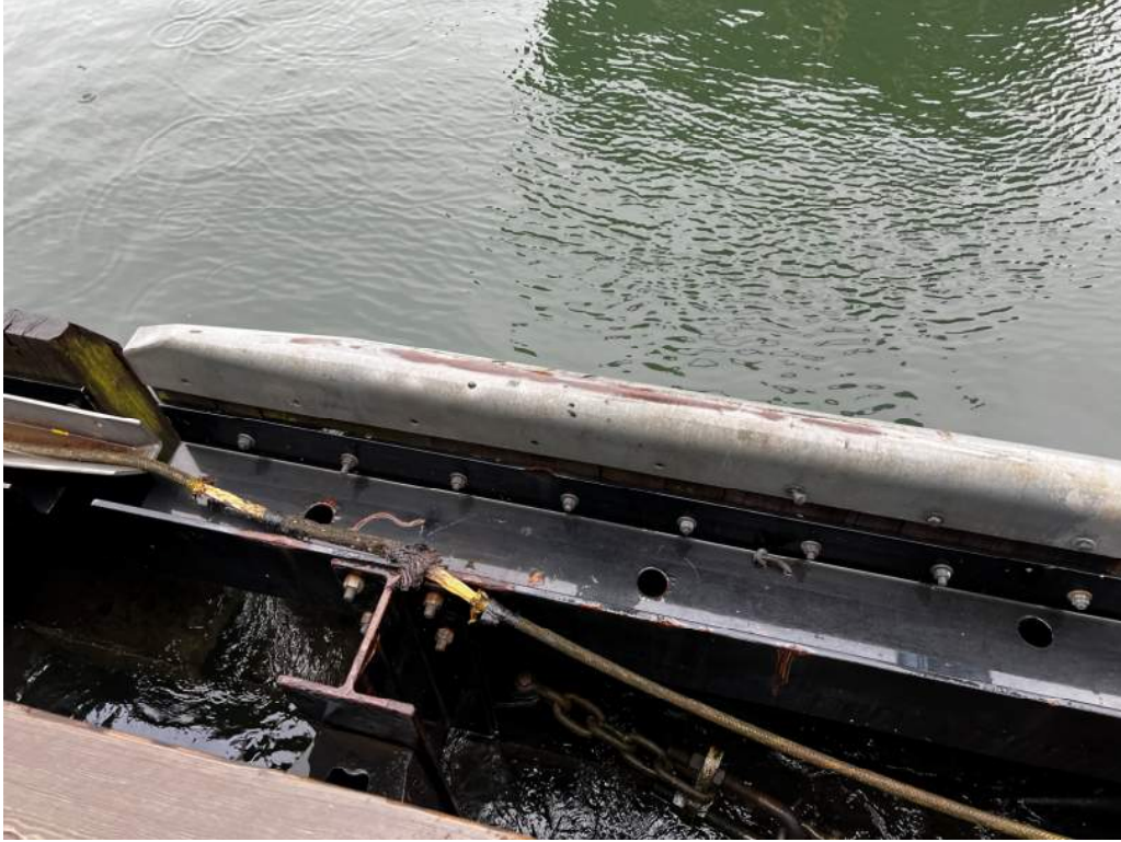
Photo 5. Typical missing bolts for the cap plate.
