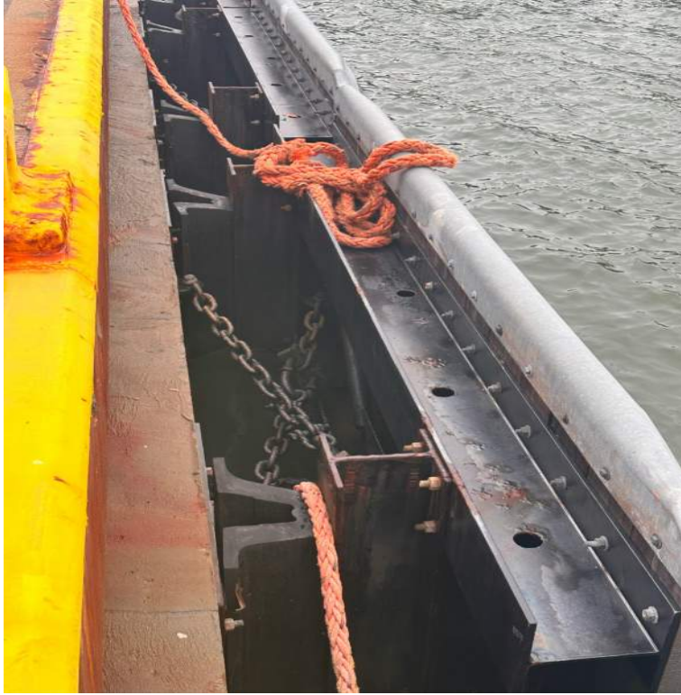
Photo 9. Rubber fender detached from concrete bulkhead at fender #17.
