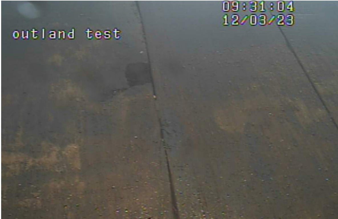
Photo 15. Minor rot at top of fender #5.
