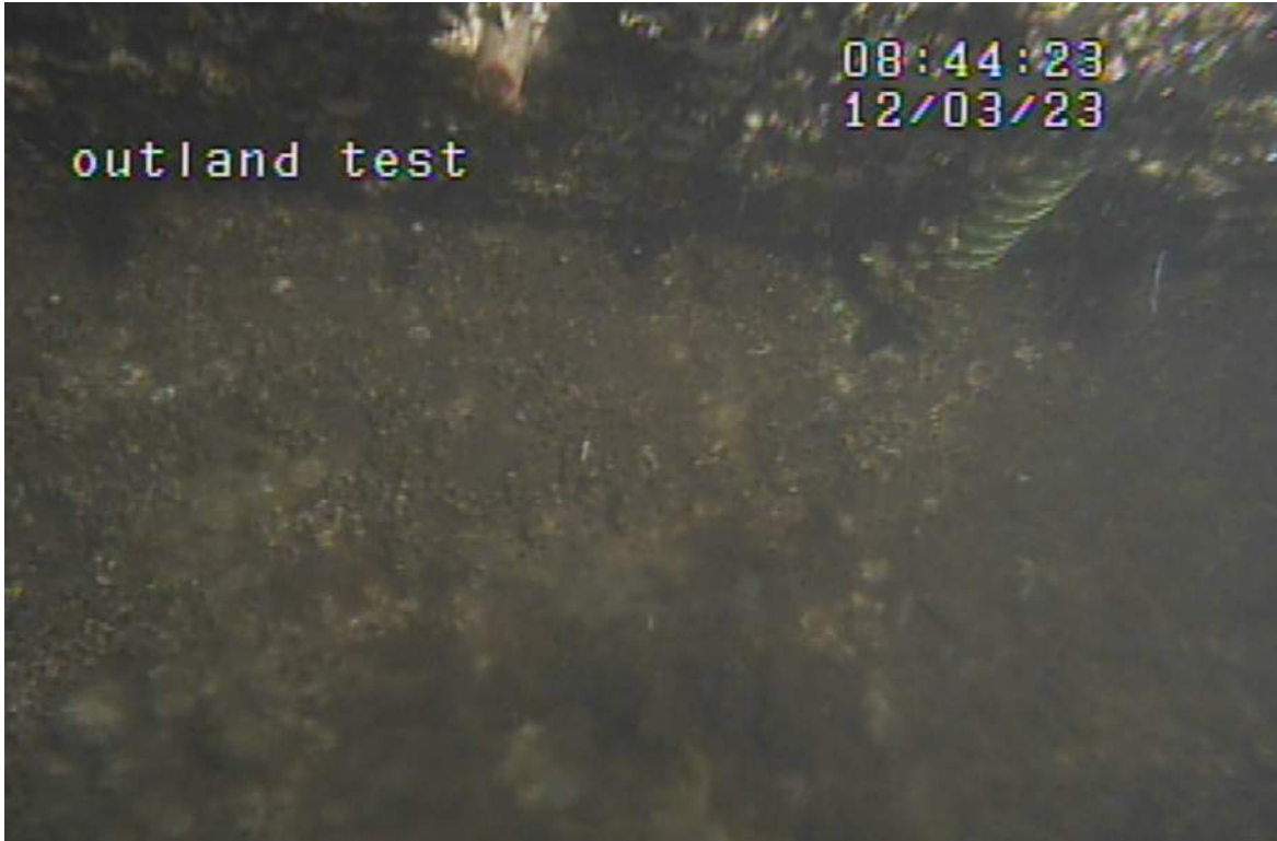
Photo 11. Exposed rebar at concrete bulkhead at fender #1.
