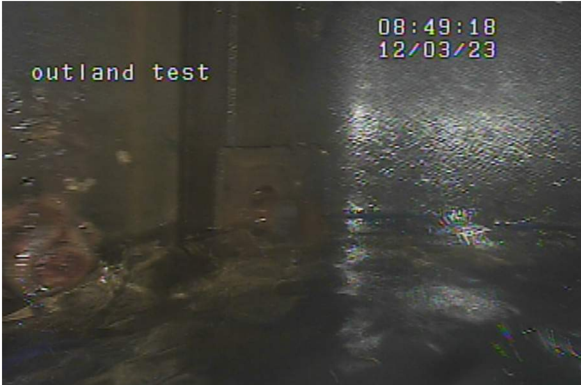
Photo 11. Loose bolt at fender #1.
