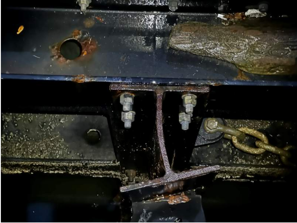
Photo 7. Close view of bent HP Pile and rubber fender at fender #9.
