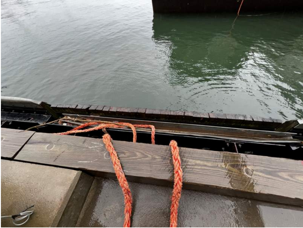
Photo 3. Missing cap plate at fender #3.
