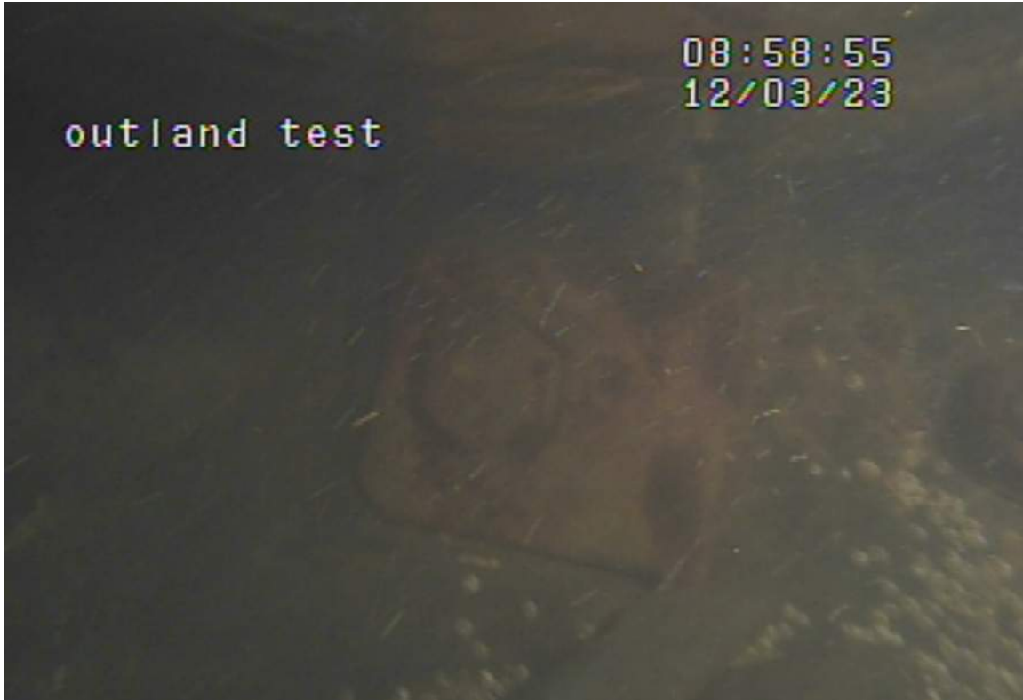
Photo 13. Loose washer at fender #2. (typical)
