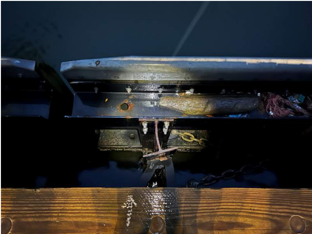
Photo 6. Bent HP Pile and rubber fender at fender #9.
