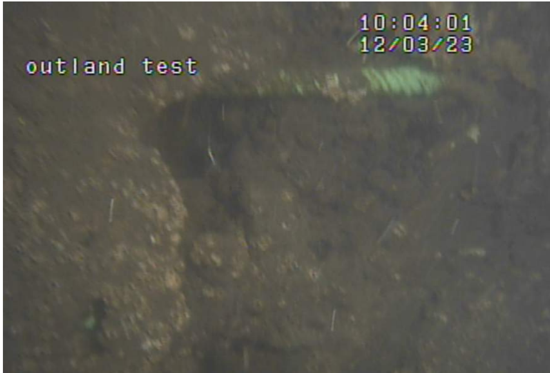
Photo 17. Exposed rebar at fender #7.
