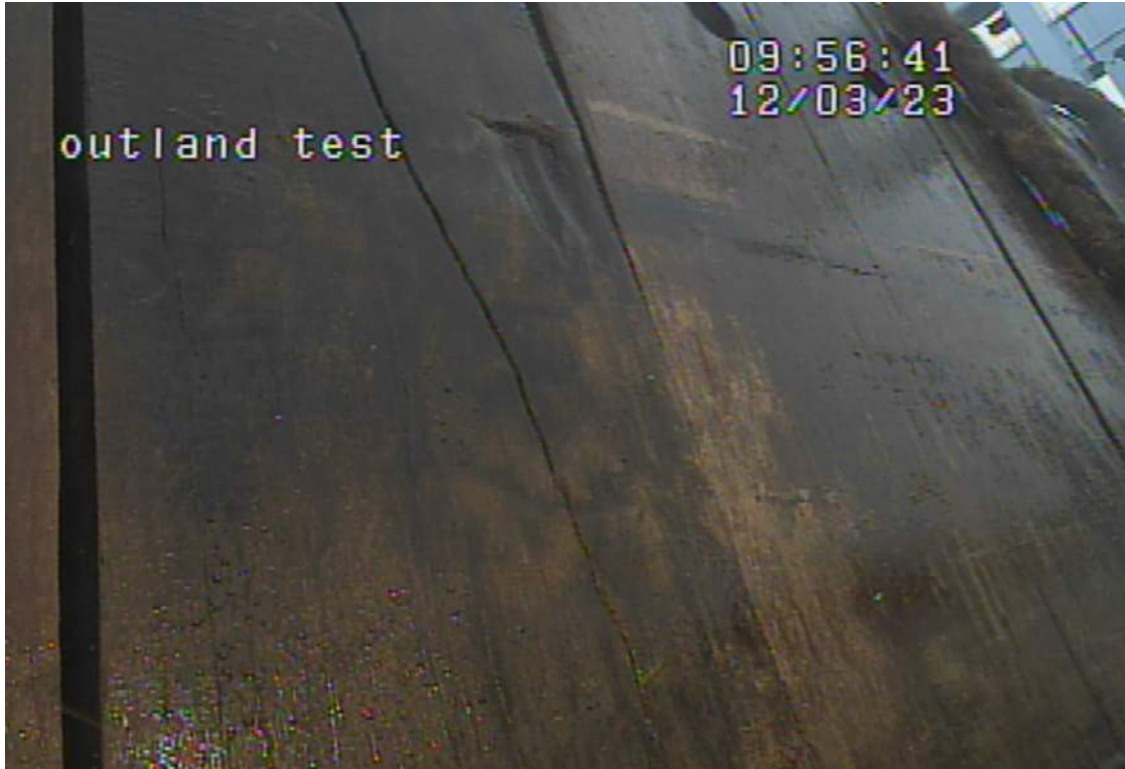
Photo 16. Vertical Split at face board at fender #7.
