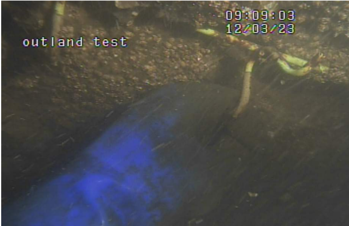
Photo 14. Exposed chair at underside of concrete deck.
