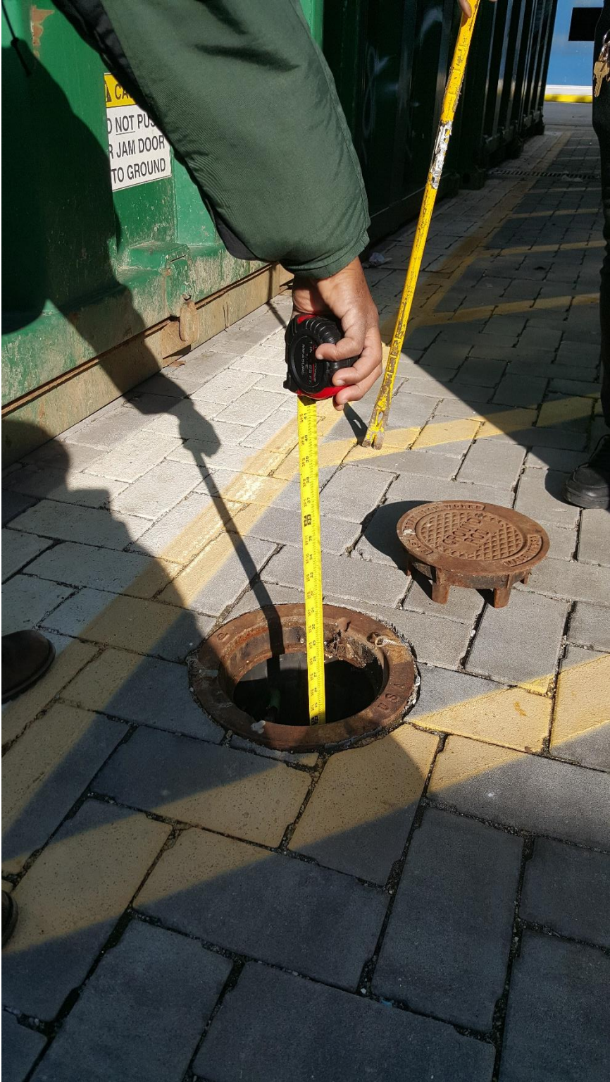
Photo 3 – Inspection Port with Cover Removed
