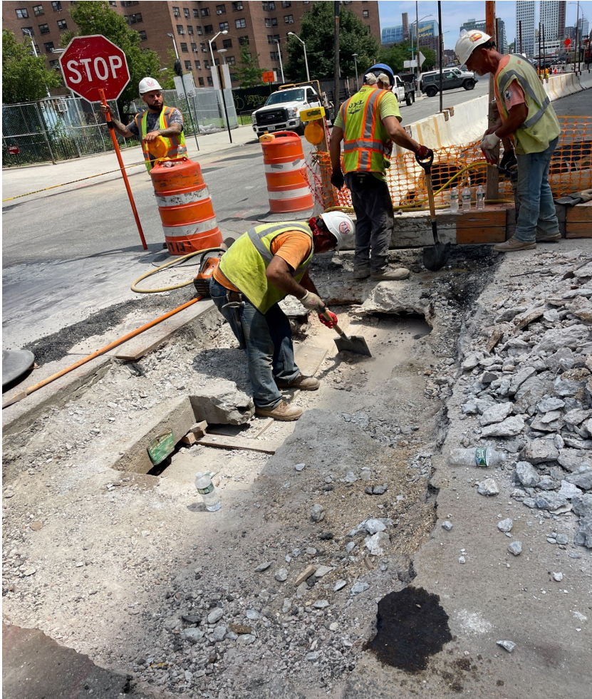
Con Ed manhole roof slab replacement at Delancey Street North and Baruch Drive – August 2024
