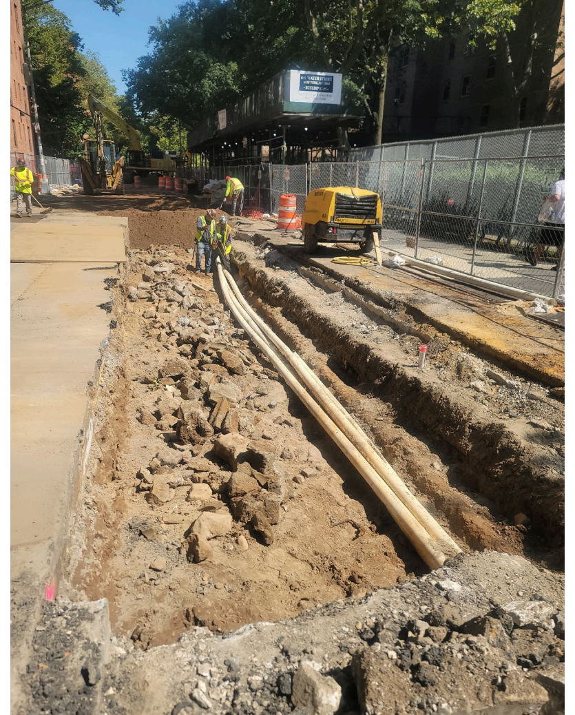
Utility wingback on Water Street – September 2024
