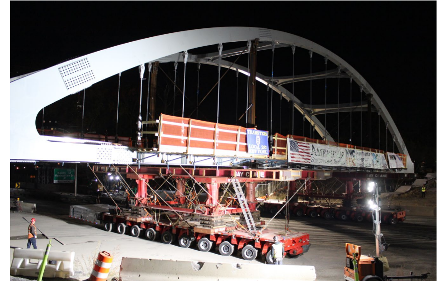
Corlears Hook Bridge rolled via SPMTs along FDR Drive during overnight closure – October 2024
