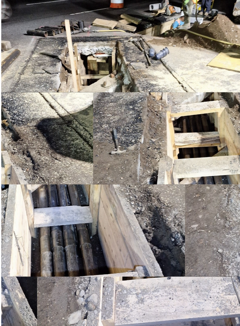
Con Ed conduit installation near FDR Drive and Corlears Hook Park – November 2024
