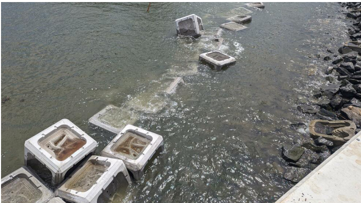
ECO Armor Blocks and Tide Pool Armors, June 2024
