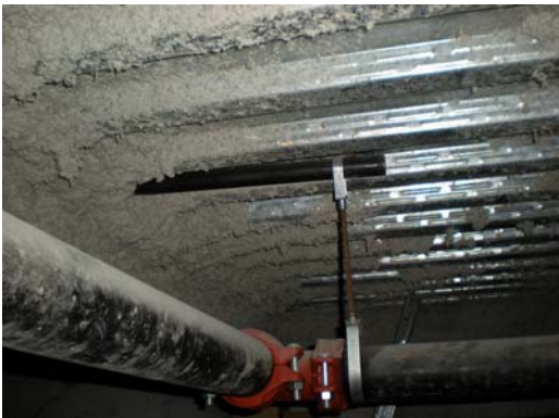
Sprinkler System Improper Hanger
