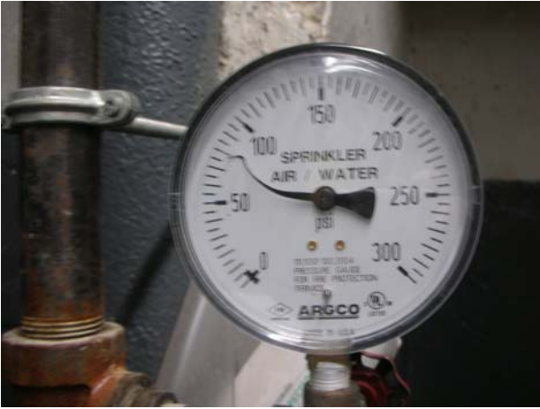
Defective Water Pressure Gauge
