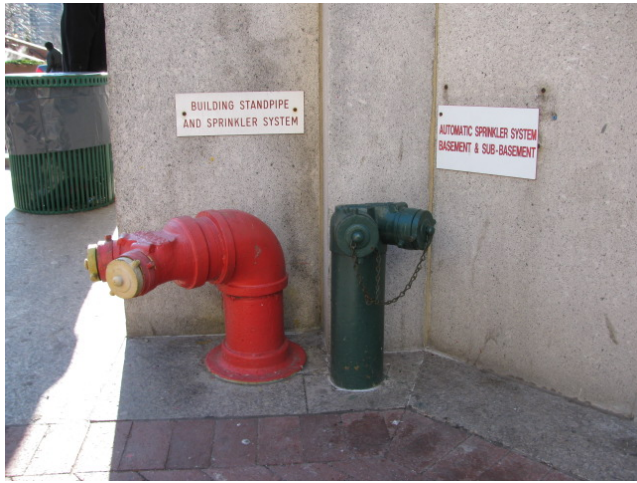
Sprinkler & Standpipe Fire Department Connections
