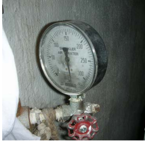
Defective Water Pressure Gauge Exposed to Freezing Temps
