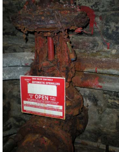
Corroded Curb Valve in Sidewalk Vault
