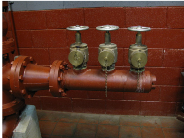
Fire Department Test Manifold
