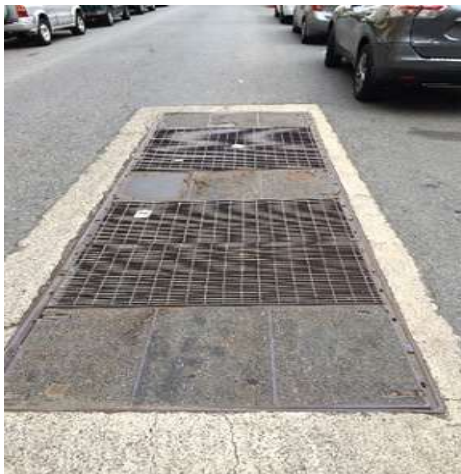
Transformer Vault (Street)
