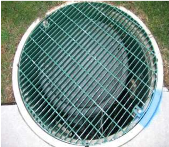
Silo Transformer (Generic Grate Cover no Con Ed Logo)
