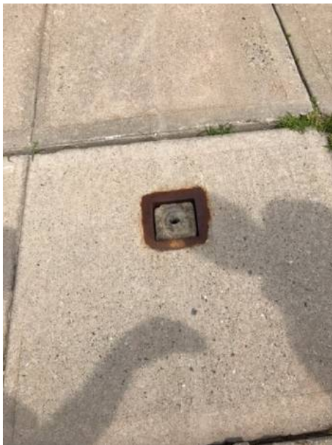
Curb Valve/Service Valve Cover
