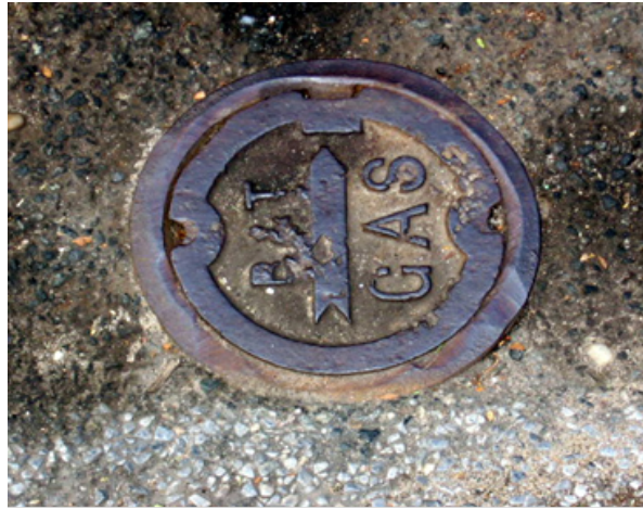
National Grid Long Service Curb Valve/Service Valve Cover
