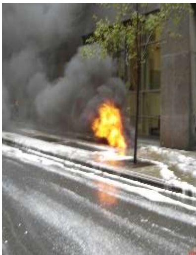
Cable Fire in a Transformer Vault
