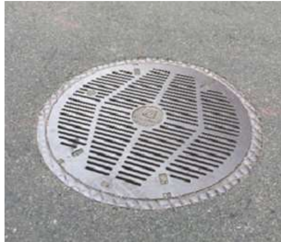
Regular Vented Manhole Cover (Note the presence of the Con Ed Logo)
