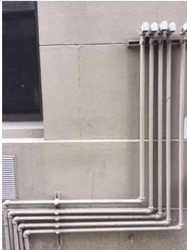
Multiple Peck Vents on a Building with Multiple Service Regulators
