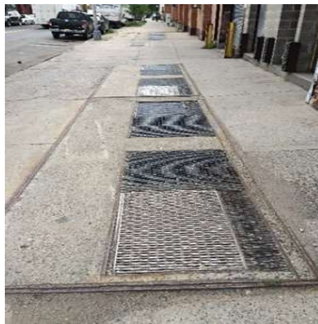
Transformer Vault (Sidewalk)
