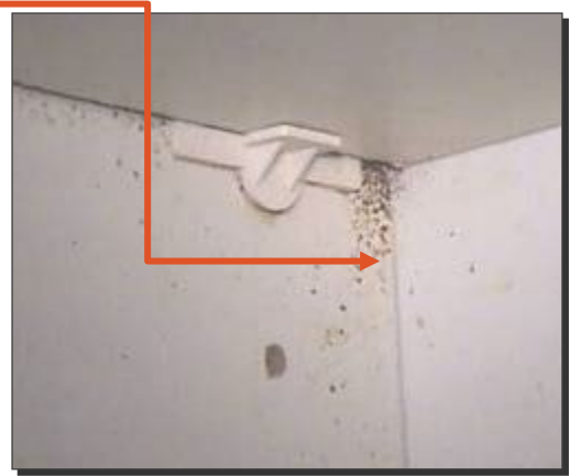
Cockroach dropping ("frass") under cabinets
