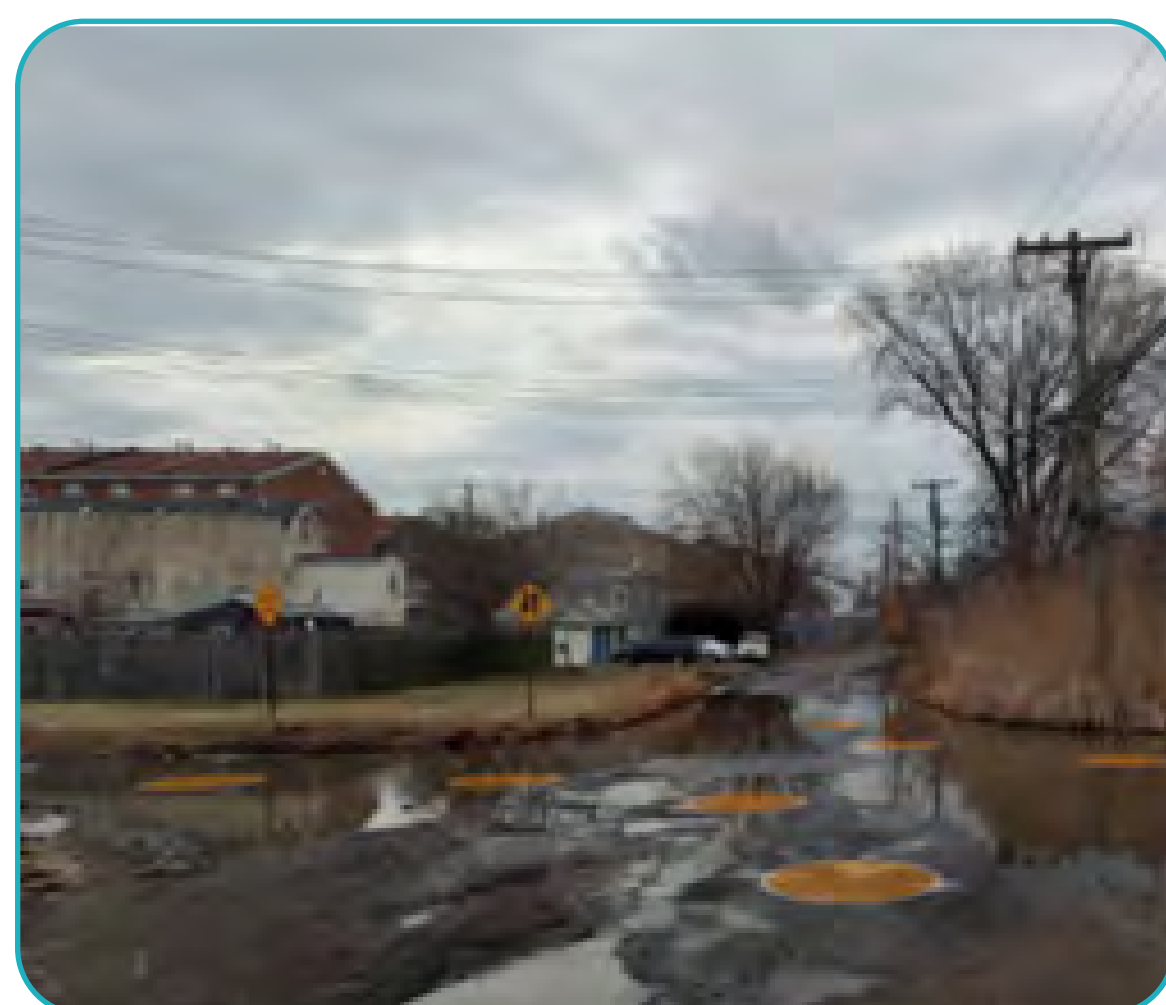
intersection of Loring Avenue and Sapphire Street with water ponding
