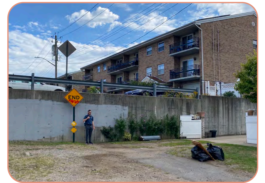
3 Drainage challenge: Privately-built retaining walls in the south Jewel Streets show the significant elevant change and create dead ends around the neighborhood
